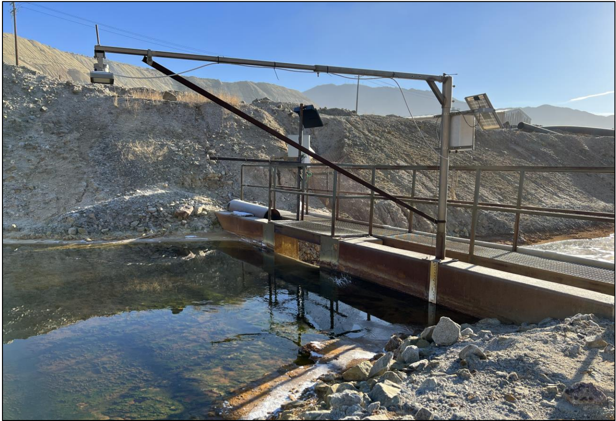
Photo 5.1 HsB Weir and Sensors (November 28, 2023)
