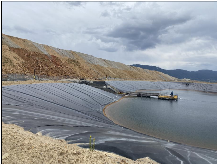
PHOTO 4 – August 30, 2023 – WED Extraction Pond and Dewatering System.
