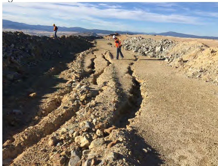
North-South Embankment Crest Cracking (2016)
