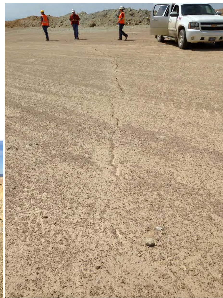
North-South Embankment Crest Cracking (2015)
