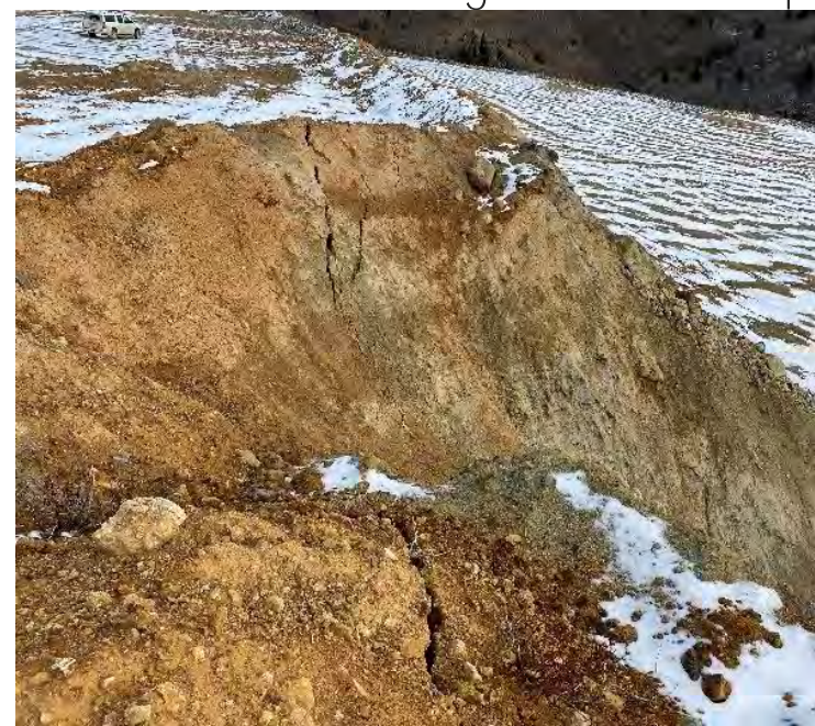
North-South Embankment Crest Cracking (2019)
