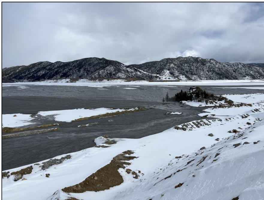
PHOTO 4 – March 13, 2024 – Discharge from West Embankment (looking south)
