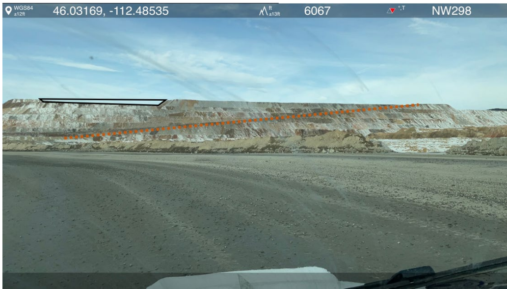
Photo 5- Only a portion of the crest has not been constructed to this elevation, near the juncture between N-S and E-W Embankments (outlined in black). The primary haul route now follows along the ramp constructed on the N-S Embankment (orange dashes).
