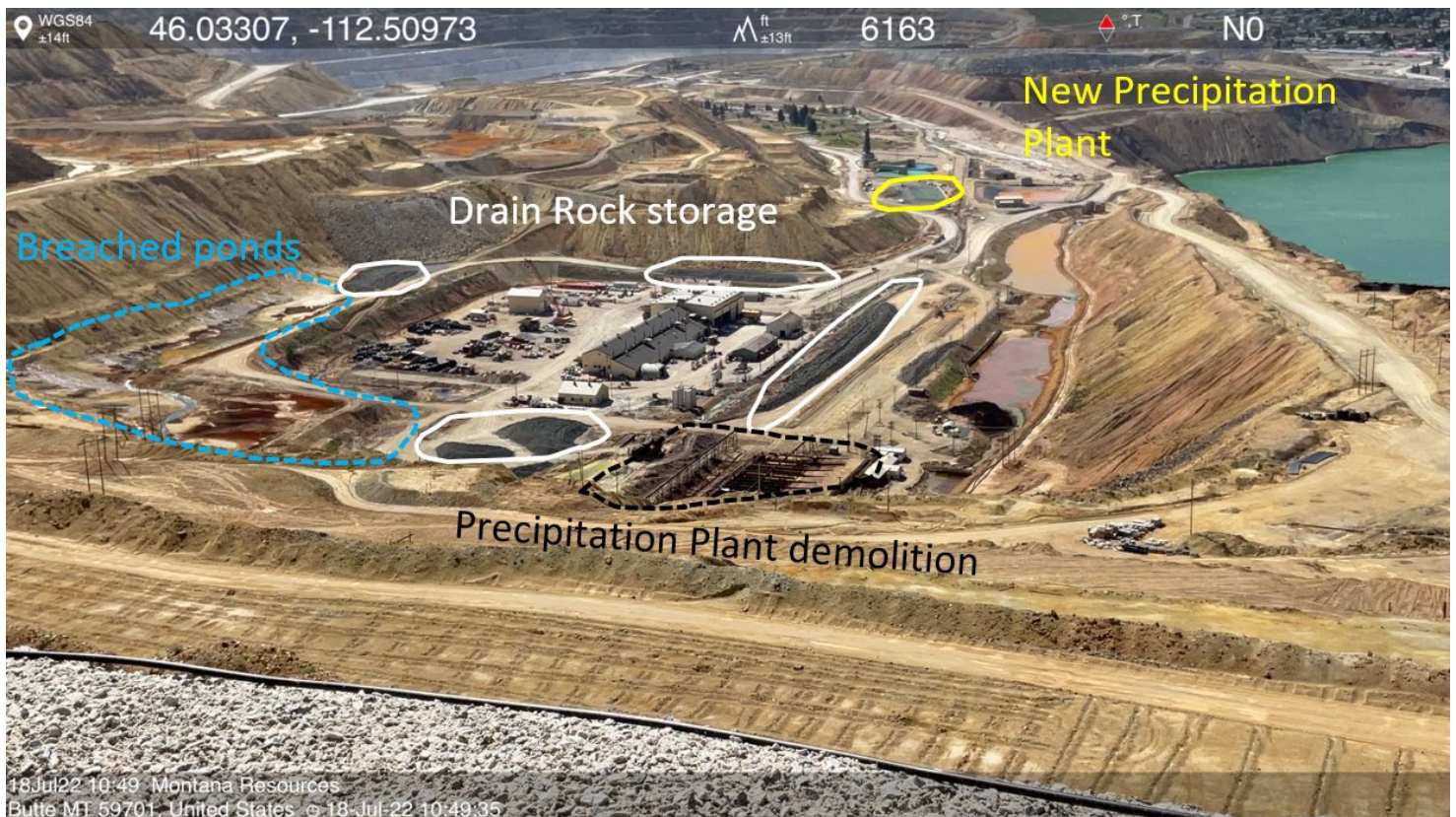
Photo 1- Looking south over the HSB area: the former Precipitation Plant is being demolished (lower center, black); water collection ponds at the toe of adjacent leach pads have been breached and drained (left, blue); drain rock from Pipestone Quarry has been placed in stockpiles around the area (white); the construction of the new Precipitation Plant near the HSB Water Treatment Plant (yellow); Berkeley Pit to the distant right.
