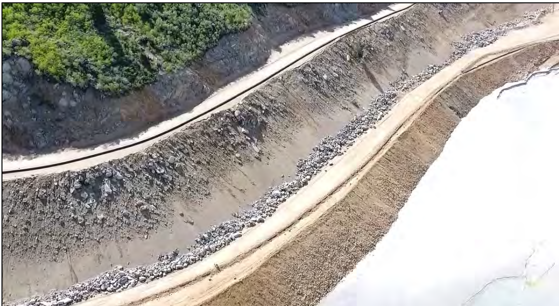
PHOTO 8 – Relocated reclaim water pipeline along the EL. 6,500 ft road.
