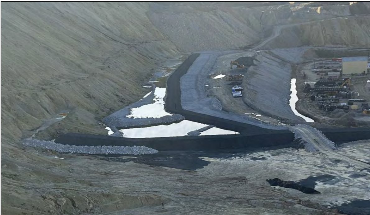
PHOTO 56 – UF – Foundation Layer material placement adjacent to rock drain D6 in the HsB Area, facing southeast.
