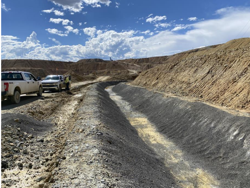
PHOTO 27 – Seep 10 – SWD#10 STA 0+500 ft looking west – 3/8" minus material placed along side slopes
