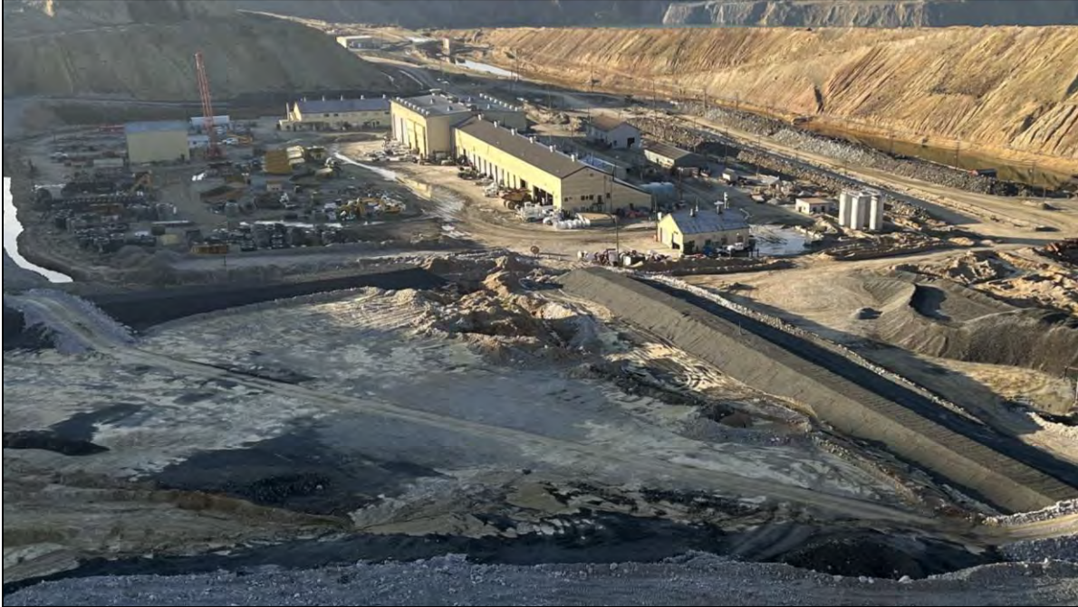
PHOTO 59 – Rock drains D4 and D7 construction progress, facing south from Number 10 Seep Bench.
