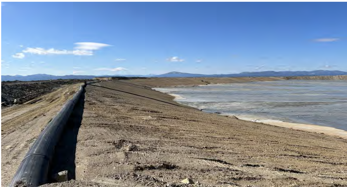
PHOTO 38 – North-South Embankment upstream side along EL. 6,450 ft tailings discharge corridor near Section 28+00N looking towards Central Pedestal Area, facing southwest.
