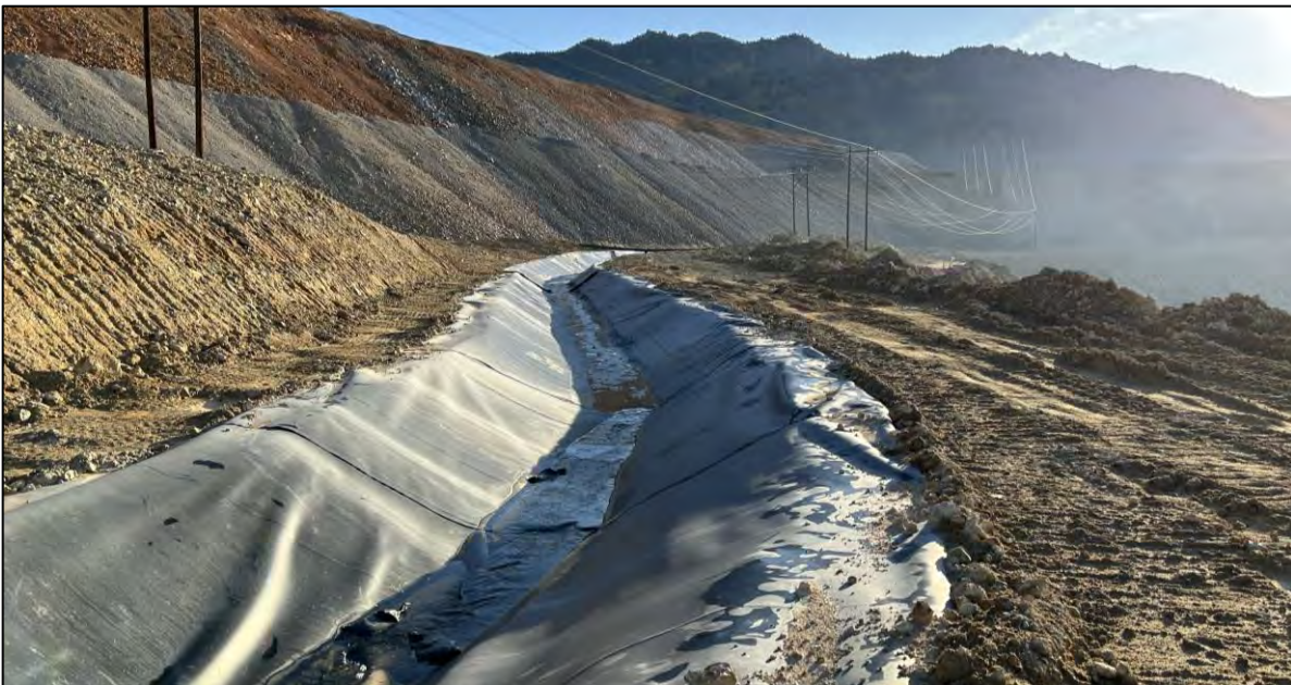
PHOTO 76 – Seep 10 bench SWD #10 conditions near Station 0+700, facing northeast.
