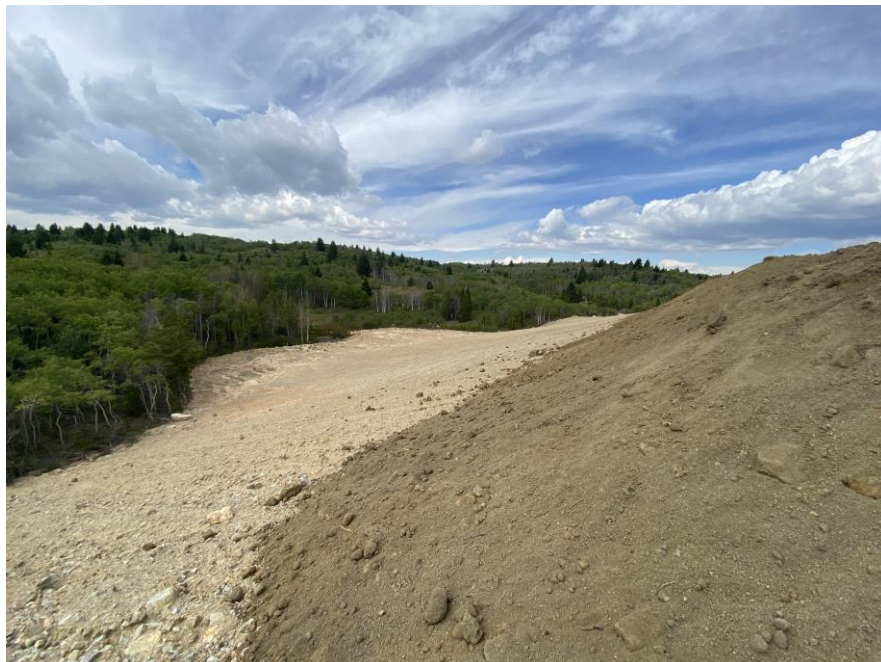
PHOTO 2 – West Embankment – Downstream face of dam receiving topsoil for reclaiming and revegetating surface
