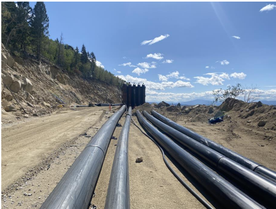
PHOTO 18 – Reclaim Road - Looking South at 5 reclaim pipes coming from the two reclaim barges
