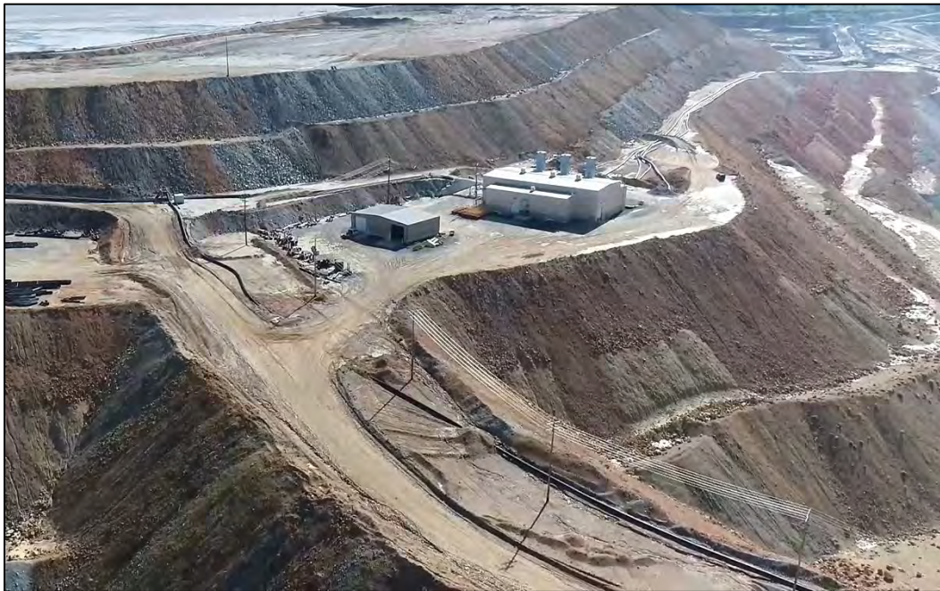
PHOTO 14 – EL. 6,450 ft lift placement complete, No. 3 Booster Pump House, and East-West pipeline ramp in Central Pedestal Area of the East West Embankment, facing east.
