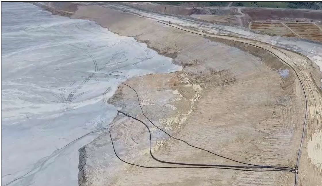
PHOTO 4 – North-South Embankment upstream regrading and alluvium facing completed up to approximately Section 28+00N, facing northeast.
