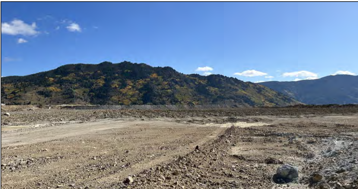
PHOTO 40 – Central Pedestal Area final grading lift progress, looking towards Section 0+00, facing east.
