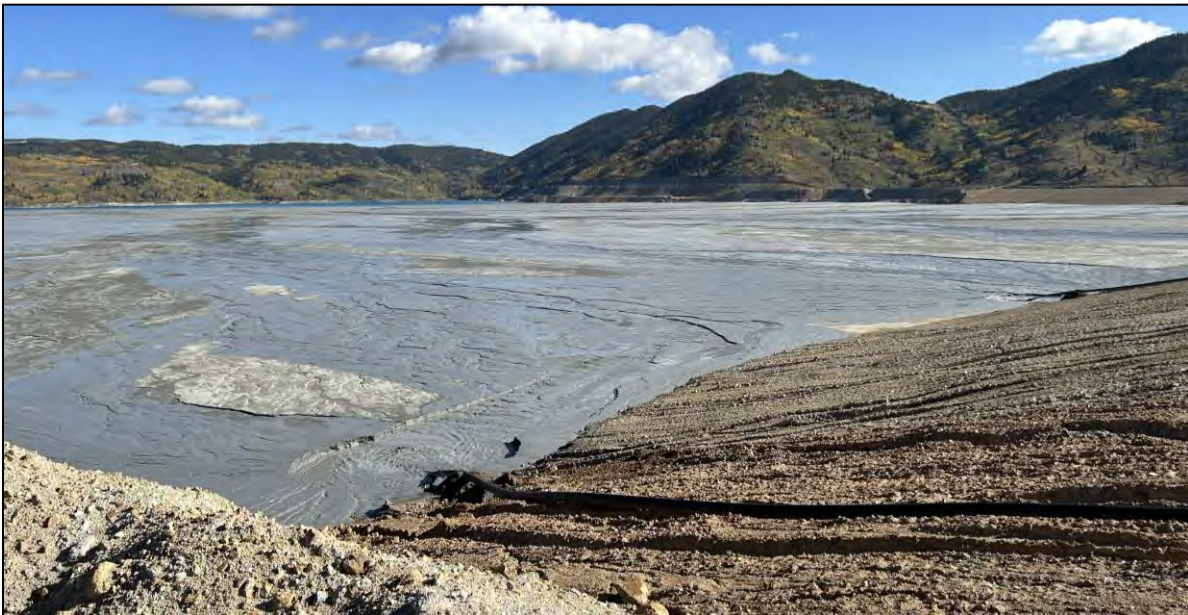
PHOTO 42 – East-West Embankment limit of upstream regrading and alluvium facing completed in Central Pedestal Area, facing northeast at Section 23+00NW.
