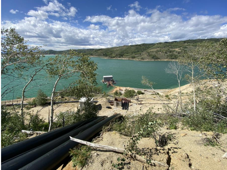
PHOTO 19 – Old reclaim barge – Outlet pipes now routed up to 6,450 ft reclaim road
