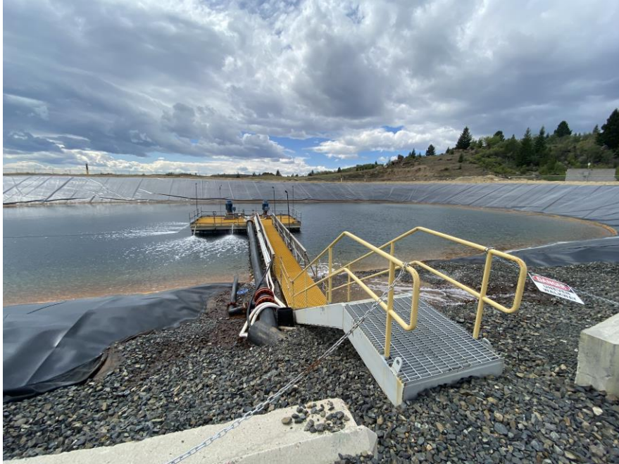
PHOTO 7 – Extraction Pond – Pumping system operating as normal
