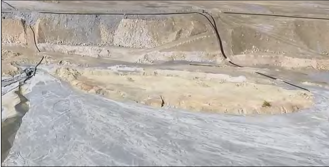
PHOTO 21 –West Embankment upstream interface near Rocky Knob, with view of discharge location RK-1 and an adjacent 12-inch discharge, facing south.
