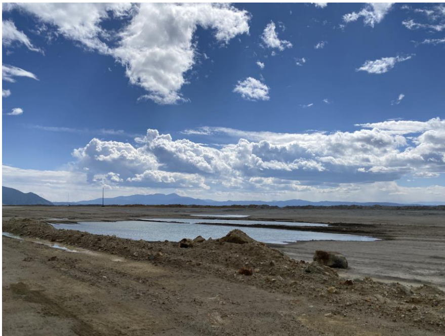
PHOTO 8 – East-West Embankment - Undulations/depressions visible along surface grade of the embankment crest due to settlement – Puddling formed after storm event
