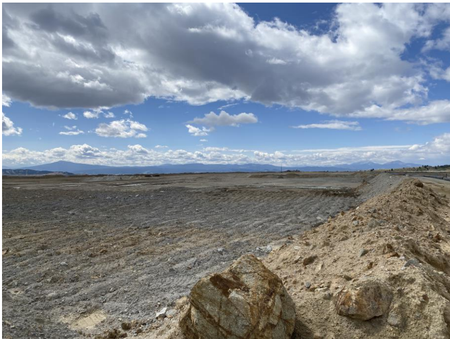
PHOTO 12 – East-West Embankment – Ripping of embankment crest for placement of material for regrading
