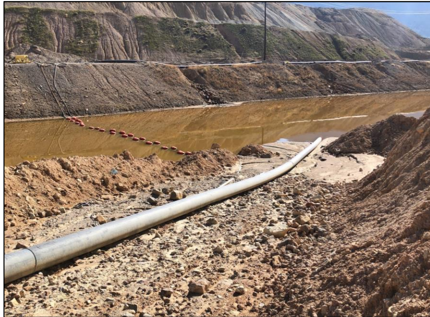
Photo 2.7 Pipeline 1 Discharge into HsB Pond
