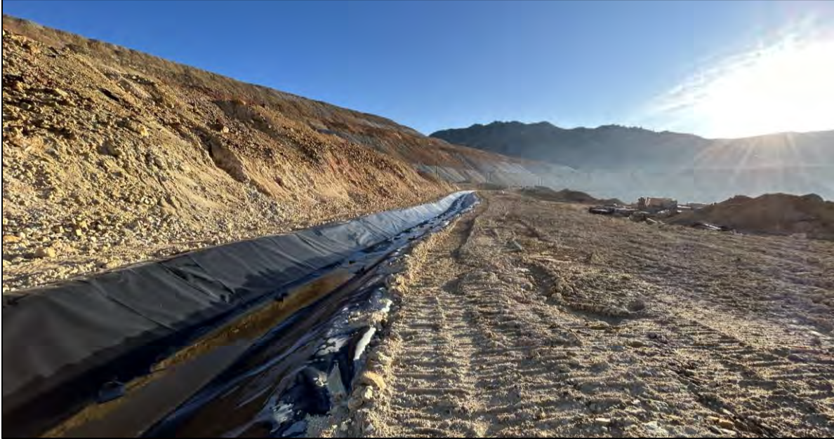
PHOTO 75 – Seep 10 bench SWD #10 conditions near Station 1+400, facing northeast.
