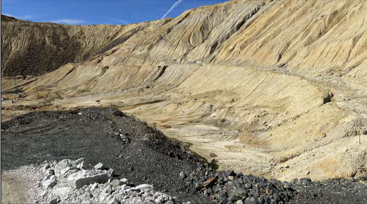
PHOTO 61 – HsB area along downstream toe of East-West Embankment, facing west from recently construction rock drain D4
