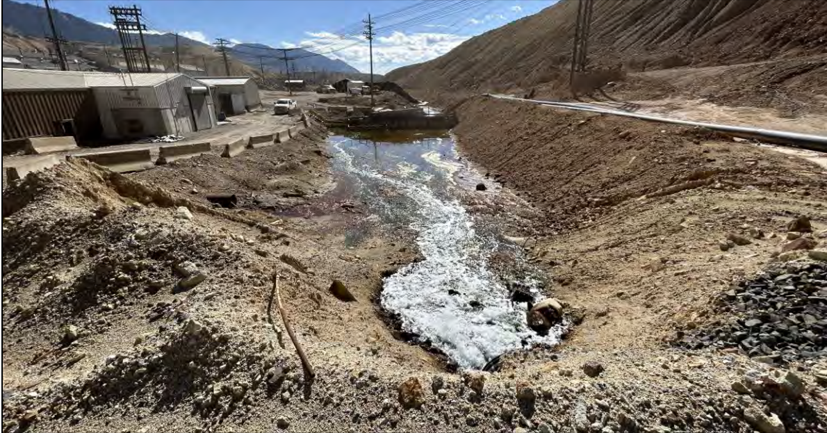
PHOTO 67 – HsB area below upper pond prior to demolition, salvage and pond breaching activities, facing south.
