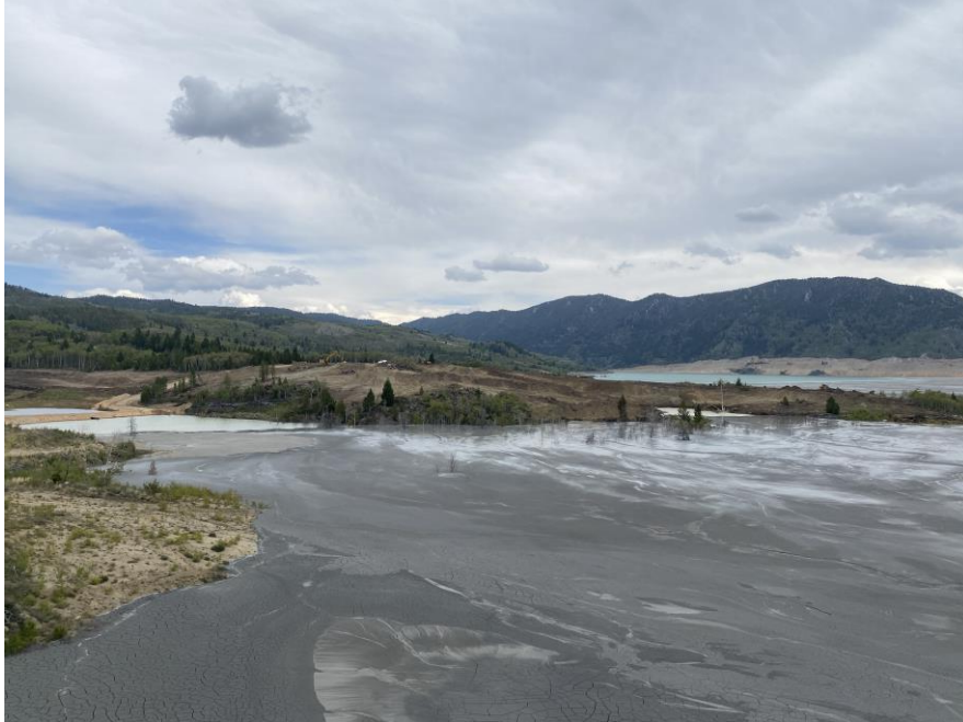
PHOTO 5 – West Embankment – Clearing and grubbing of area east of the north abutment
