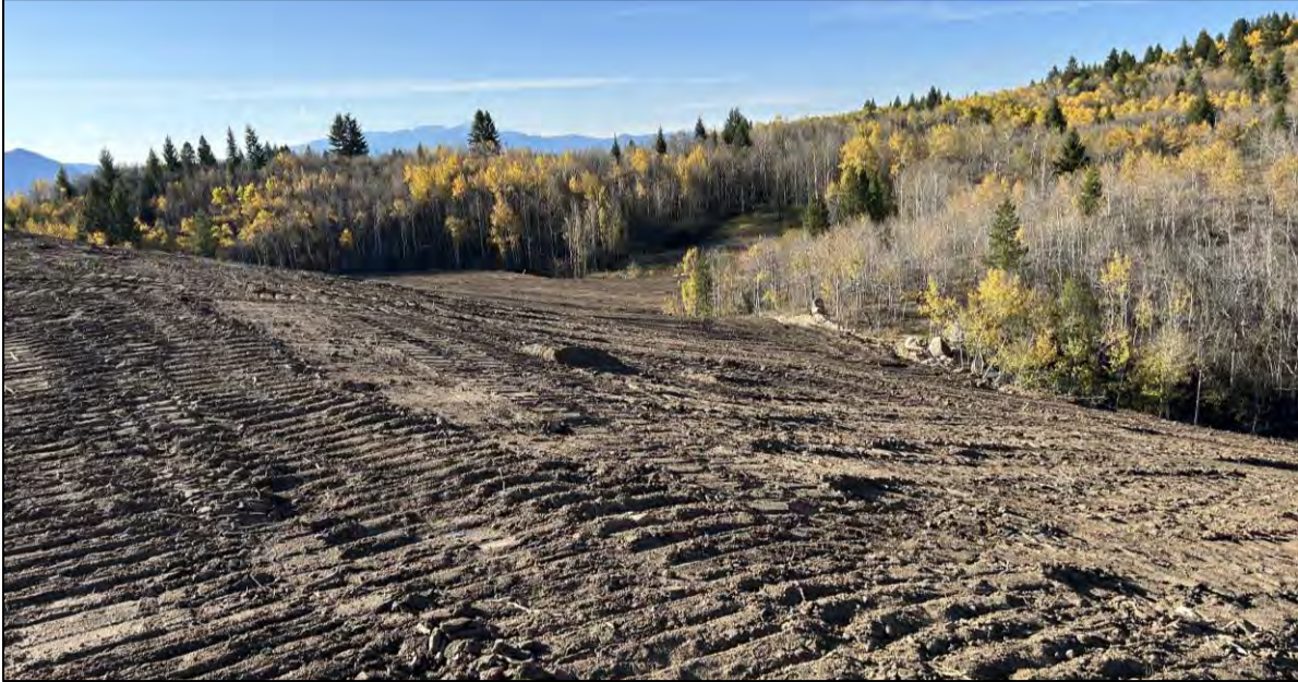
PHOTO 47 – Downstream side of West Embankment near Section 70+00W. Final grading and trimming to 3H:1V slope angle with topsoil placement completed, facing southwest.
