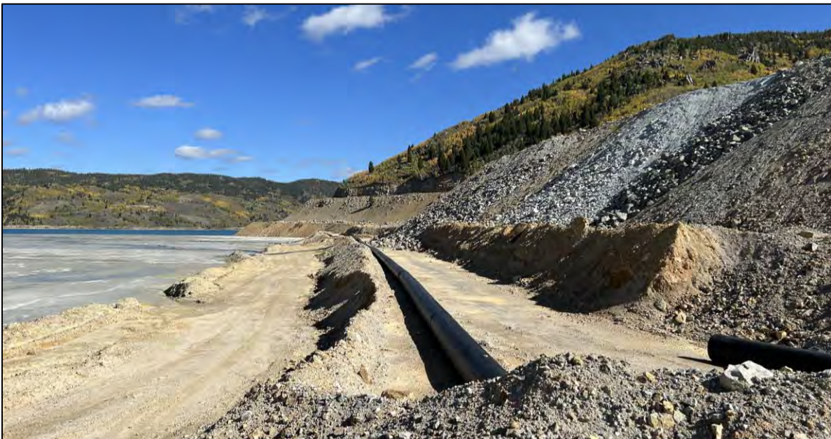
PHOTO 36 – North-South Embankment upstream side along EL. 6,400 ft tailings discharge corridor and EL. 6,450 ft lift placement near Discharge 3-4, facing northeast.
