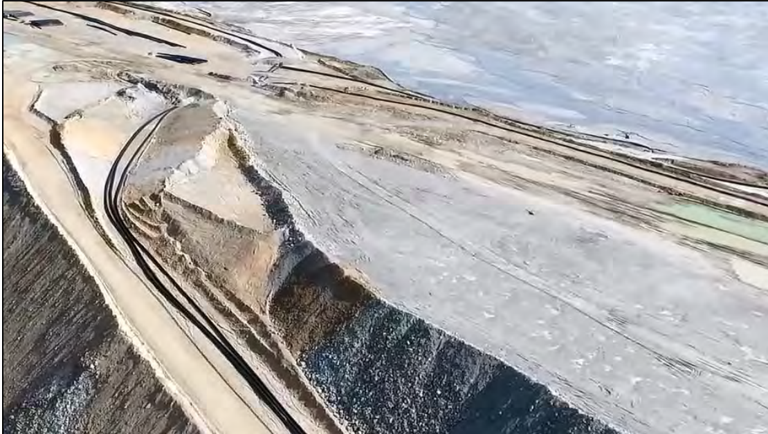
PHOTO 19 – East-West Embankment EL. 6,450 ft lift and surcharge zone, with view of adjacent tailings beach and Line 3, recently routed over the EL. 6,450 ft lift.
