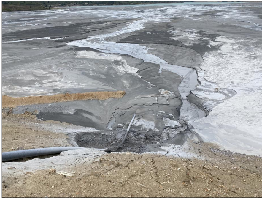
Photo 2.1 EL. 6,450 ft West Embankment Discharge Spigot 1-2B 12" Valve Leaking
