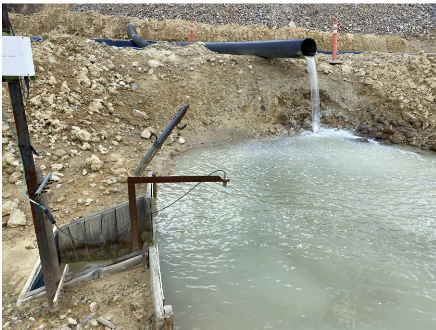
PHOTO 24 – Seep 10 – Pond inflows
