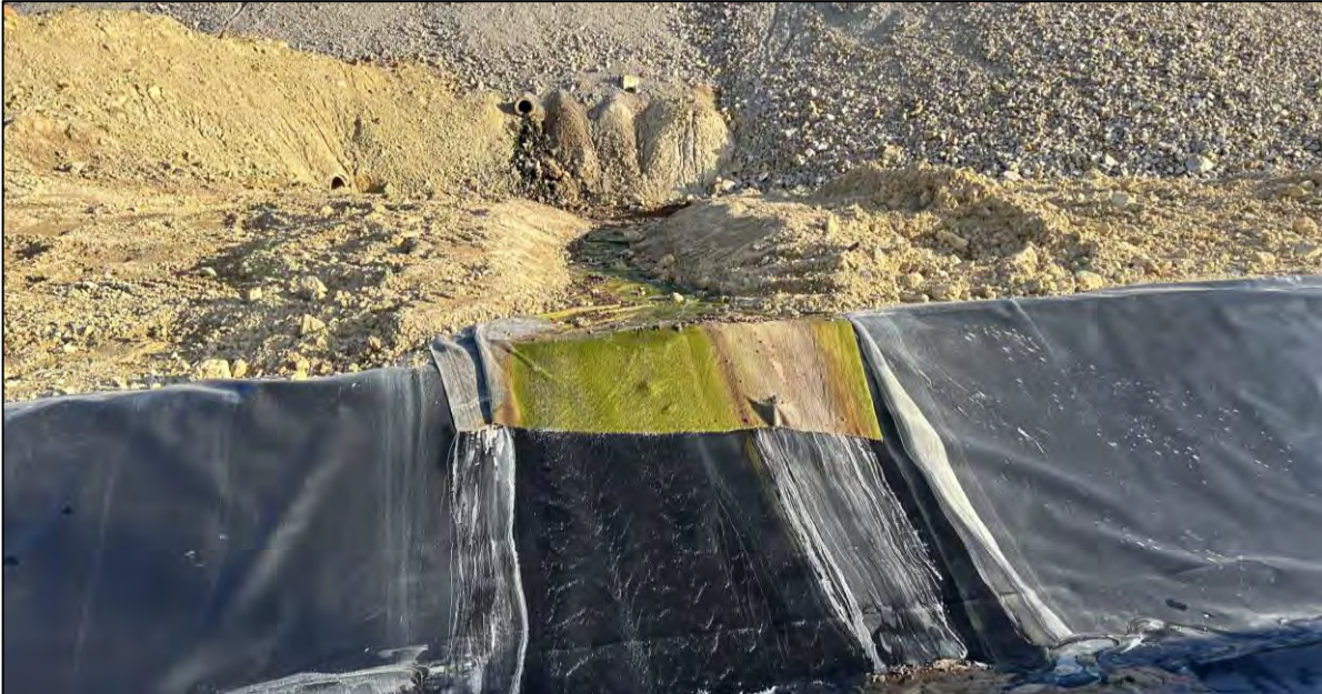
PHOTO 77 – Seep 10 bench SWD #10 conditions near Station 0+300 at Seep 10 inflow, facing north.
