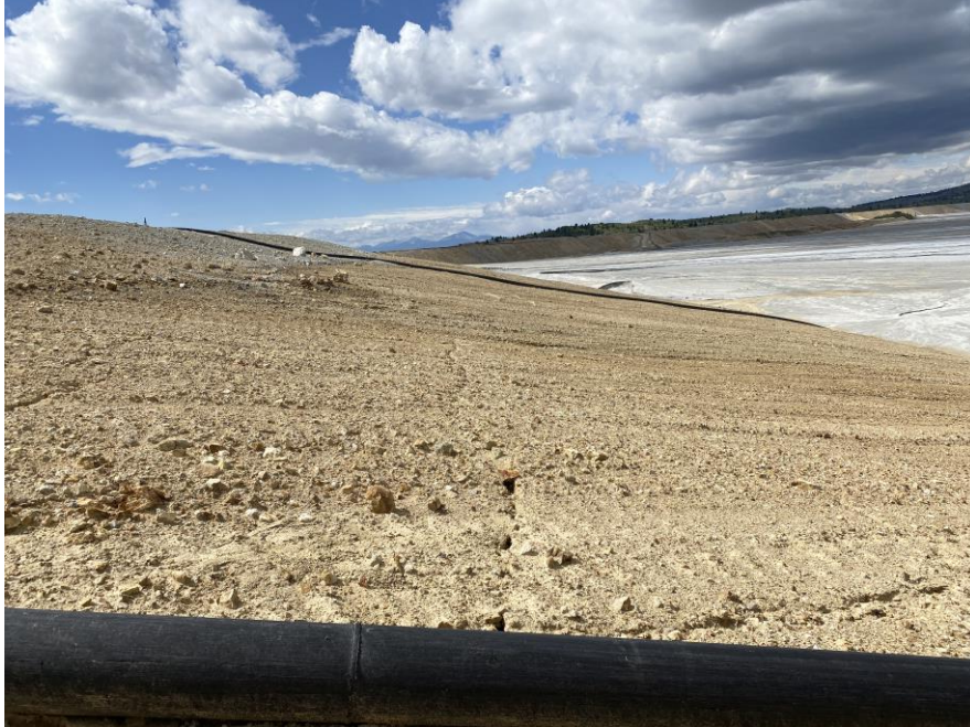
PHOTO 9 – East-West Embankment – Settling cracks noticed within the upstream face with the Zone F facing
