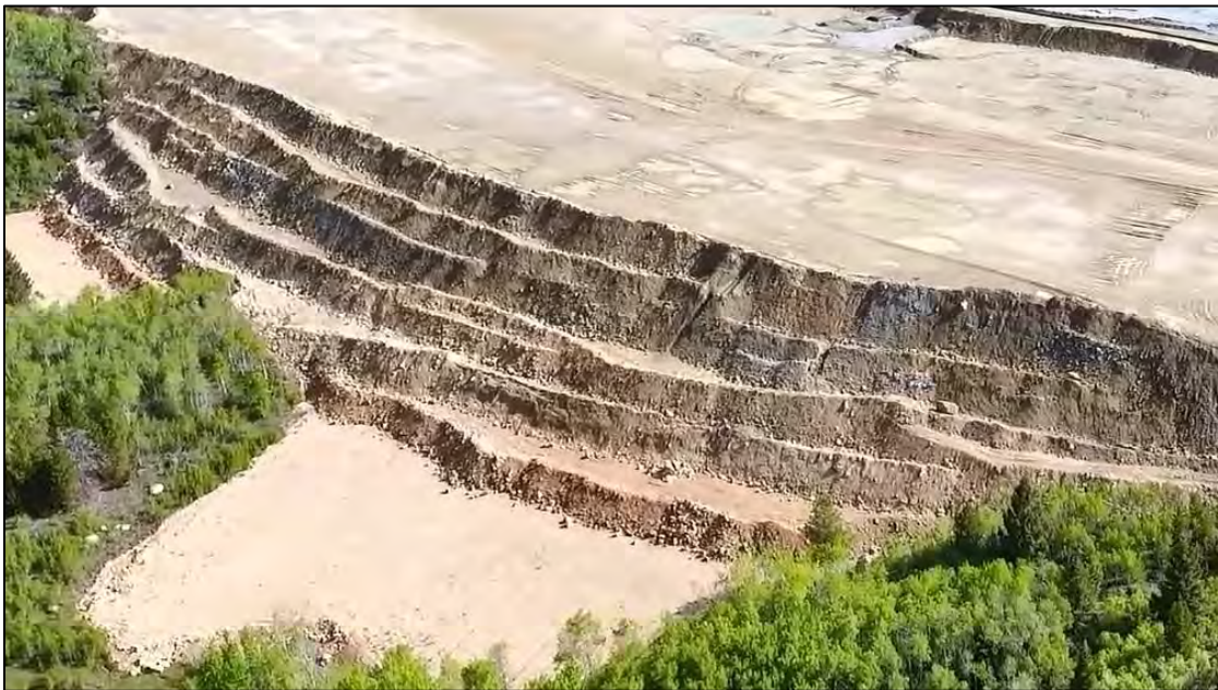
PHOTO 26 – West Embankment downstream shell before final grading and trimming, northwest of Rocky Knob and Extraction Pond, looking northeast.
