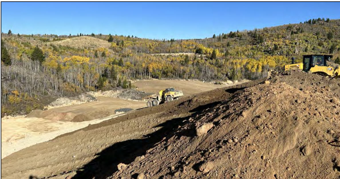
PHOTO 50 – Downstream side of West Embankment near Section 105+00W. Final grading and trimming to 3H:1V slope angle completed with topsoil placement in progress, facing westnorth.
