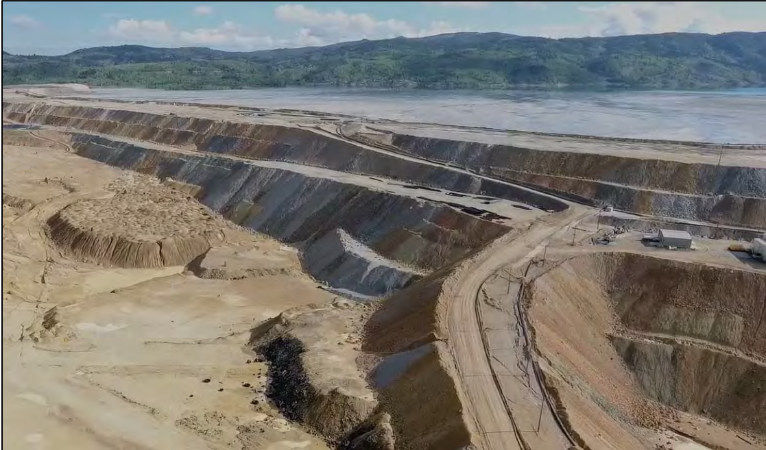
PHOTO 15 – East-West Embankment downstream side along northwest trending limb with No. 3 Booster Pump House on right hand side, looking north.
