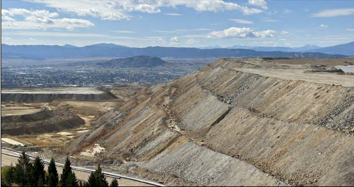
PHOTO 35 – North-South Embankment downstream slope with visible North RDS fill placement for the Mega Ramp, facing southwest.
