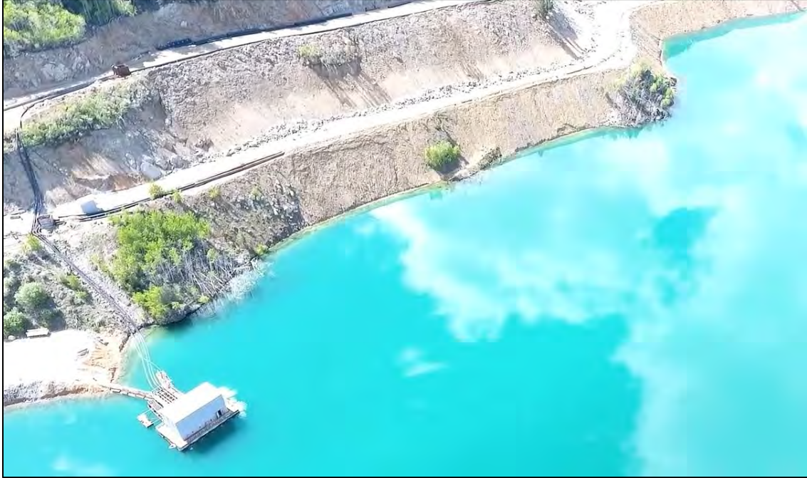
PHOTO 7 – Older Reclaim Barge connected to reclaim pipeline along the EL. 6,500 ft road.
