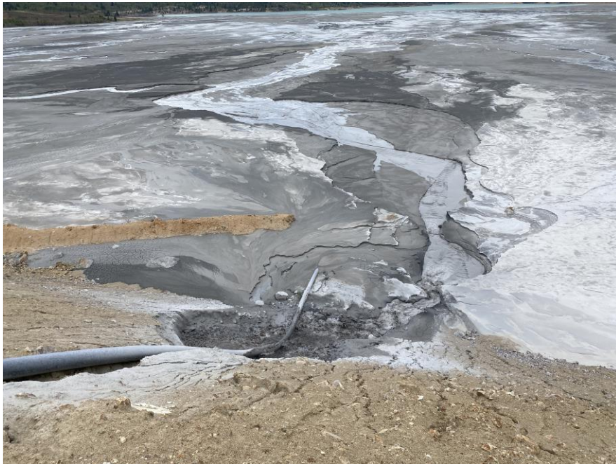
PHOTO 6 – West Embankment – Upstream face discharge 1-2B causing erosion to the embankment due to eroded discharge pipe.
