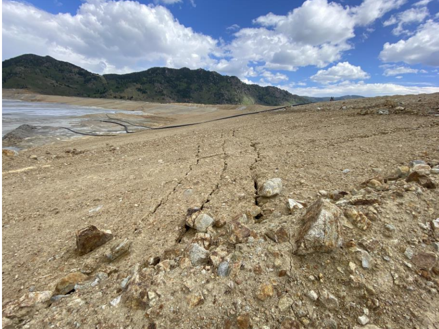
PHOTO 11 – East-West Embankment – Settling cracks noticed within the upstream face with the Zone F facing
