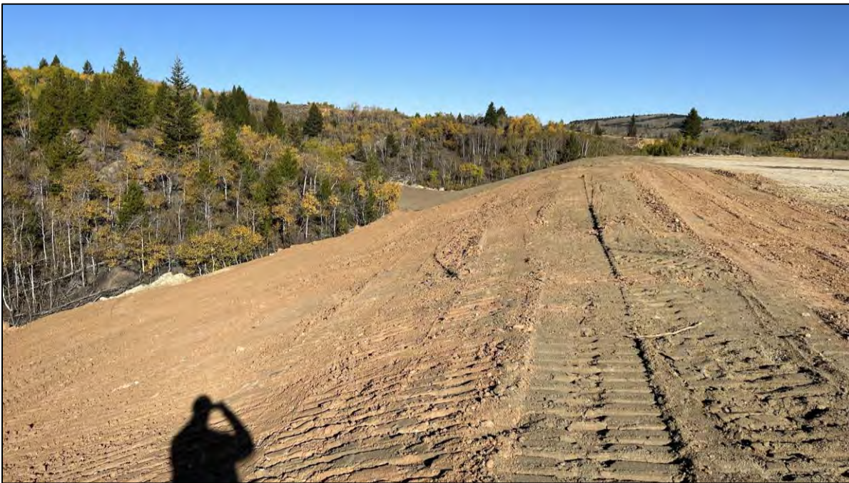
PHOTO 48 – Downstream side of West Embankment near Section 83+00W. Final grading and trimming to 3H:1V slope angle with topsoil placement completed, facing north.
