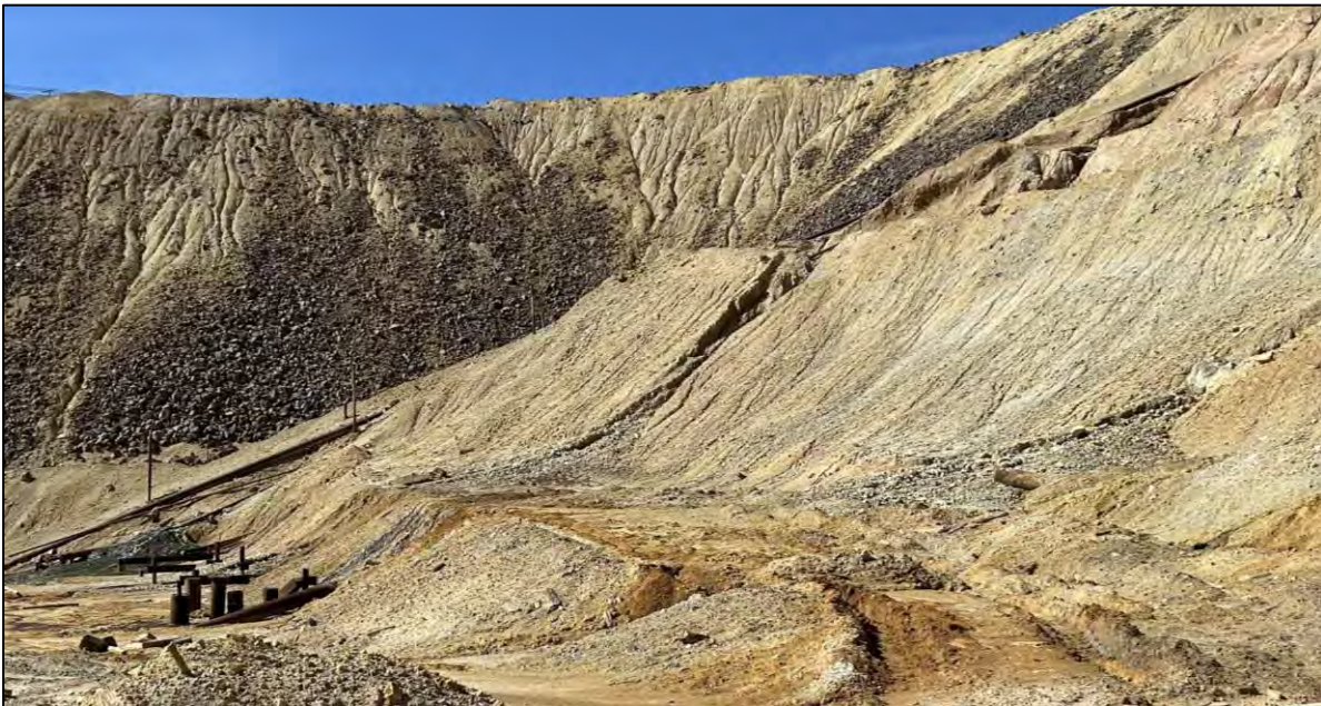
PHOTO 64 – Downstream embankment shell in the HsB area, facing west towards Section 8+00W prior to rock drain construction.
