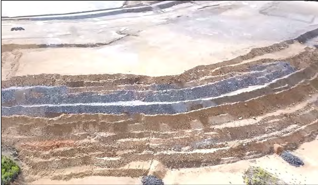
PHOTO 25 – West Embankment crest and downstream shell before final grading and trimming at northern end of West Embankment, facing east.
