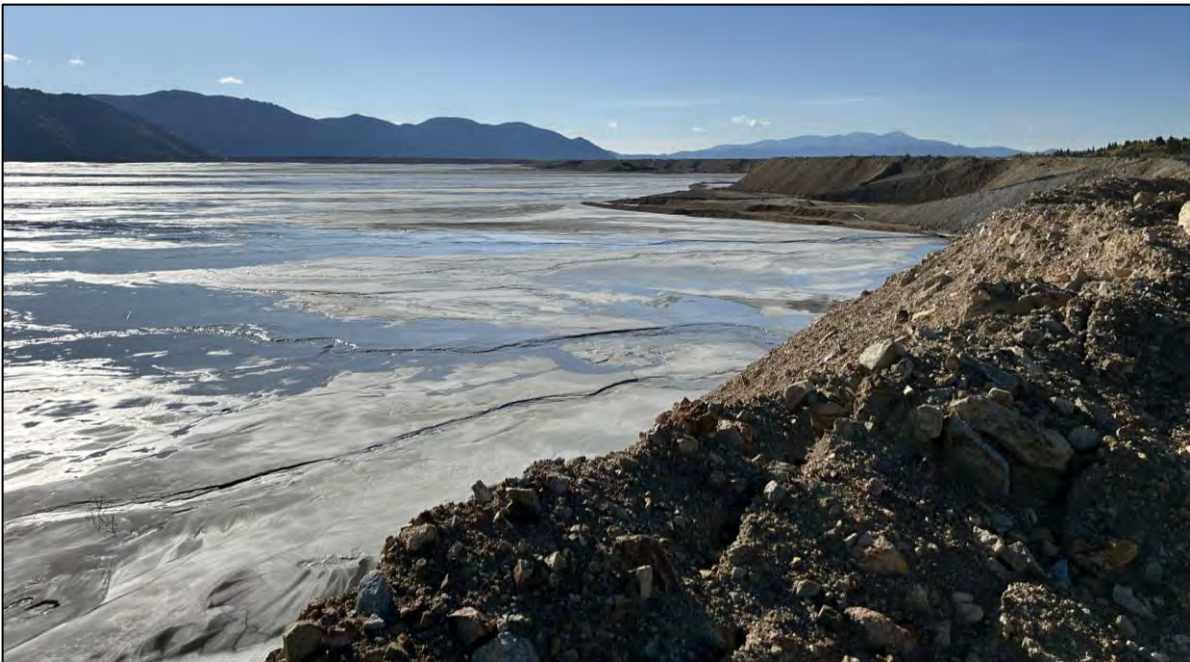
PHOTO 52 – West Embankment upstream shell (right) and tailings beach (left) by tailings discharge location RK-3, facing southeast from EL. 6,450 ft.
