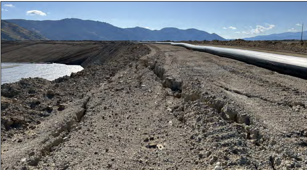
PHOTO 44 – East-West Embankment upstream side near limit of upstream regrading work at Section 23+00NW. Differential settlement cracking observed along tailings discharge corridor from Section 23+00NW to 33+00NW, facing southeast.
