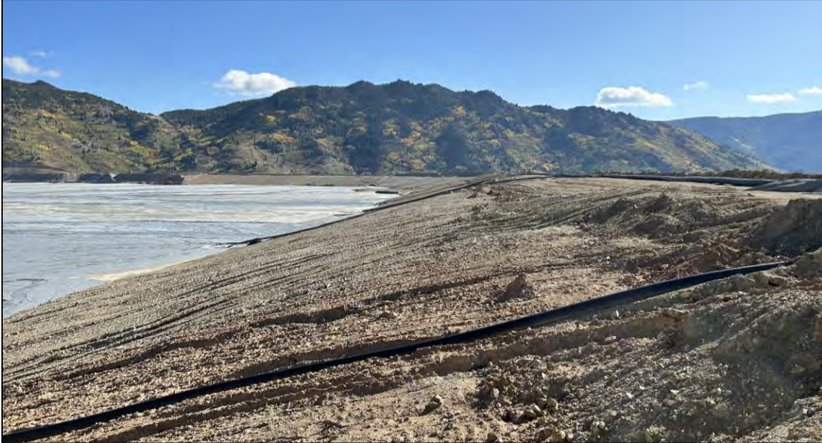
PHOTO 41 – East-West Embankment upstream regrading and alluvium facing completed in Central Pedestal Area, facing east from Section 23+00NW.
