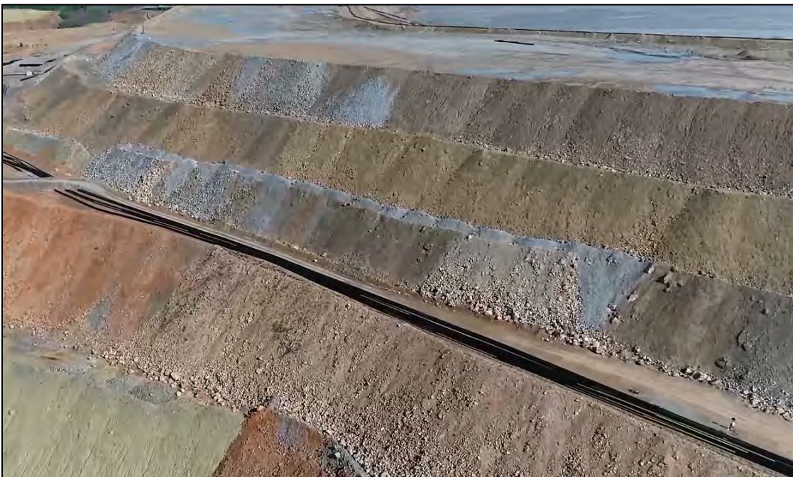
PHOTO 16 – East-West Embankment pipeline ramp with EL. 6,450 ft lift and surcharge zone placement complete, facing northwest from east of No. 3 Booster Pump House.
