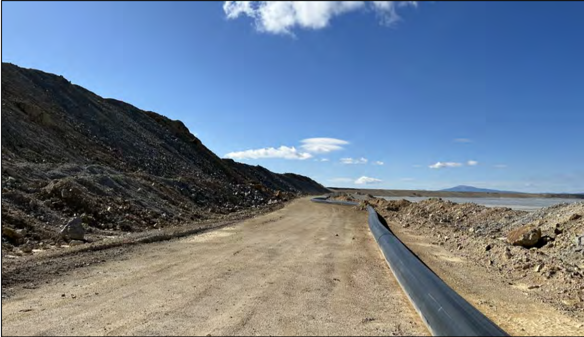
PHOTO 37 – North-South Embankment upstream side along EL. 6,400 ft tailings discharge corridor and EL. 6,450 ft lift placement near Discharge 3-4, facing southwest.
