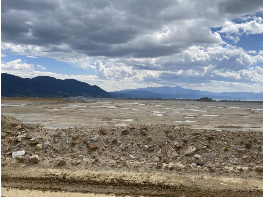
PHOTO 13 – East-West Embankment - Undulations/depressions visible along crest
