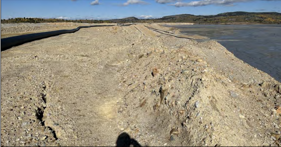
PHOTO 43 – East-West Embankment end of upstream regrading and alluvium facing completed in Central Pedestal Area, facing northwest at Section 23+00NW.
