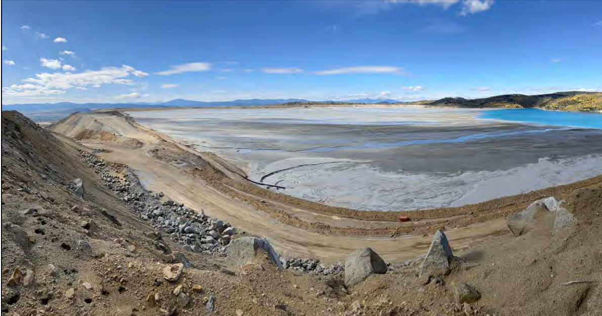
PHOTO 33 – North-South Embankment and beach, looking west from the new reclaim water pipeline road.
