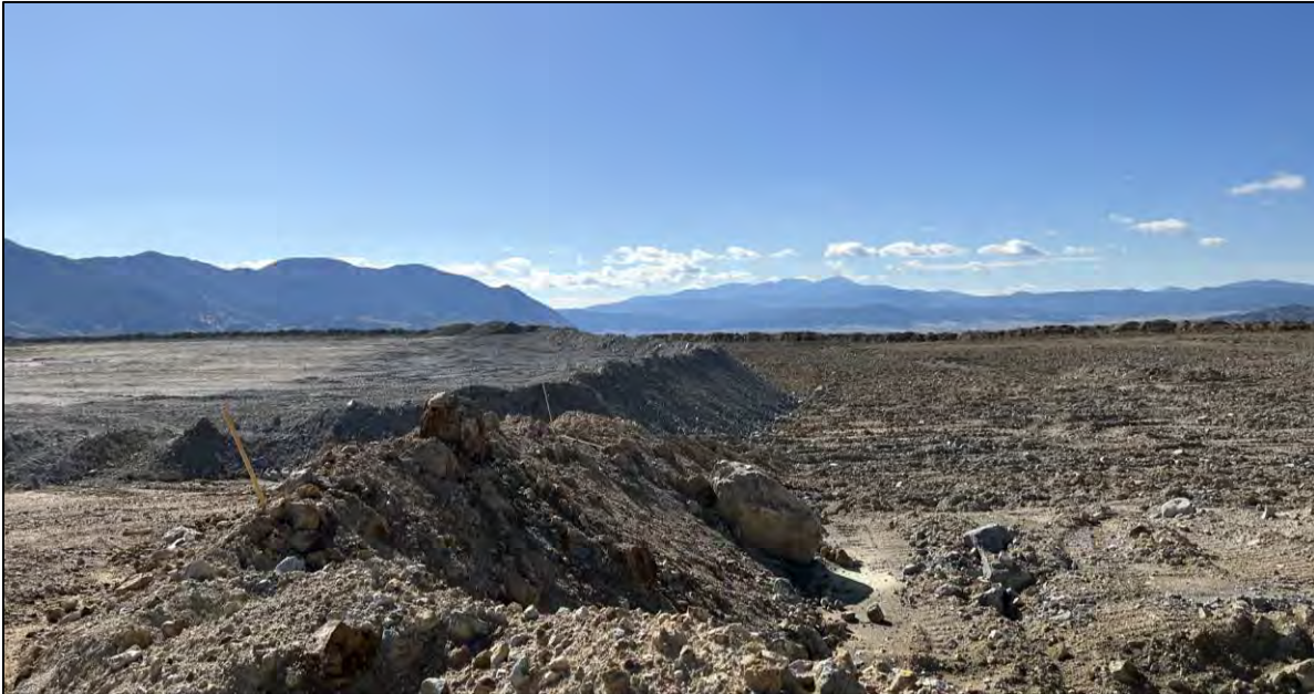
PHOTO 39 – Central Pedestal Area final grading lift progress to the east of Section 0+00, facing south. Cross ripped area on right side of image was where transverse cracking was remediated. No crack re-expression observed.
