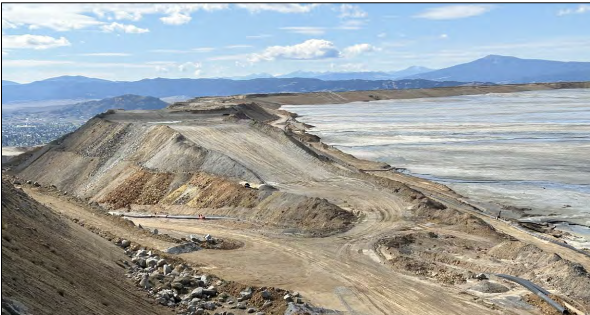
PHOTO 34 – North-South Embankment northern abutment at deferred fill placement area, looking southwest from the new reclaim pipeline road.
