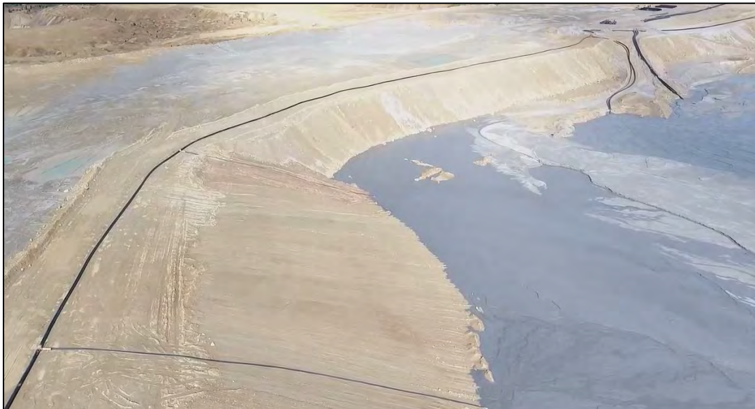
PHOTO 10 – East-West Embankment upstream side near limit of upstream regrading work at Section 23+00NW. Differential settlement cracking observed along tailings discharge corridor from Section 23+00NW to 33+00NW near the tailings discharge point (at top right corner).
