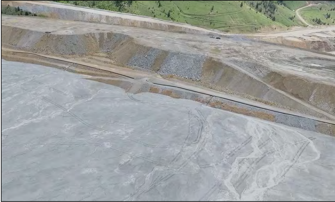
PHOTO 5 – North-South Embankment upstream regrading remains to be completed beyond approximately Section 28+00N, facing east.
