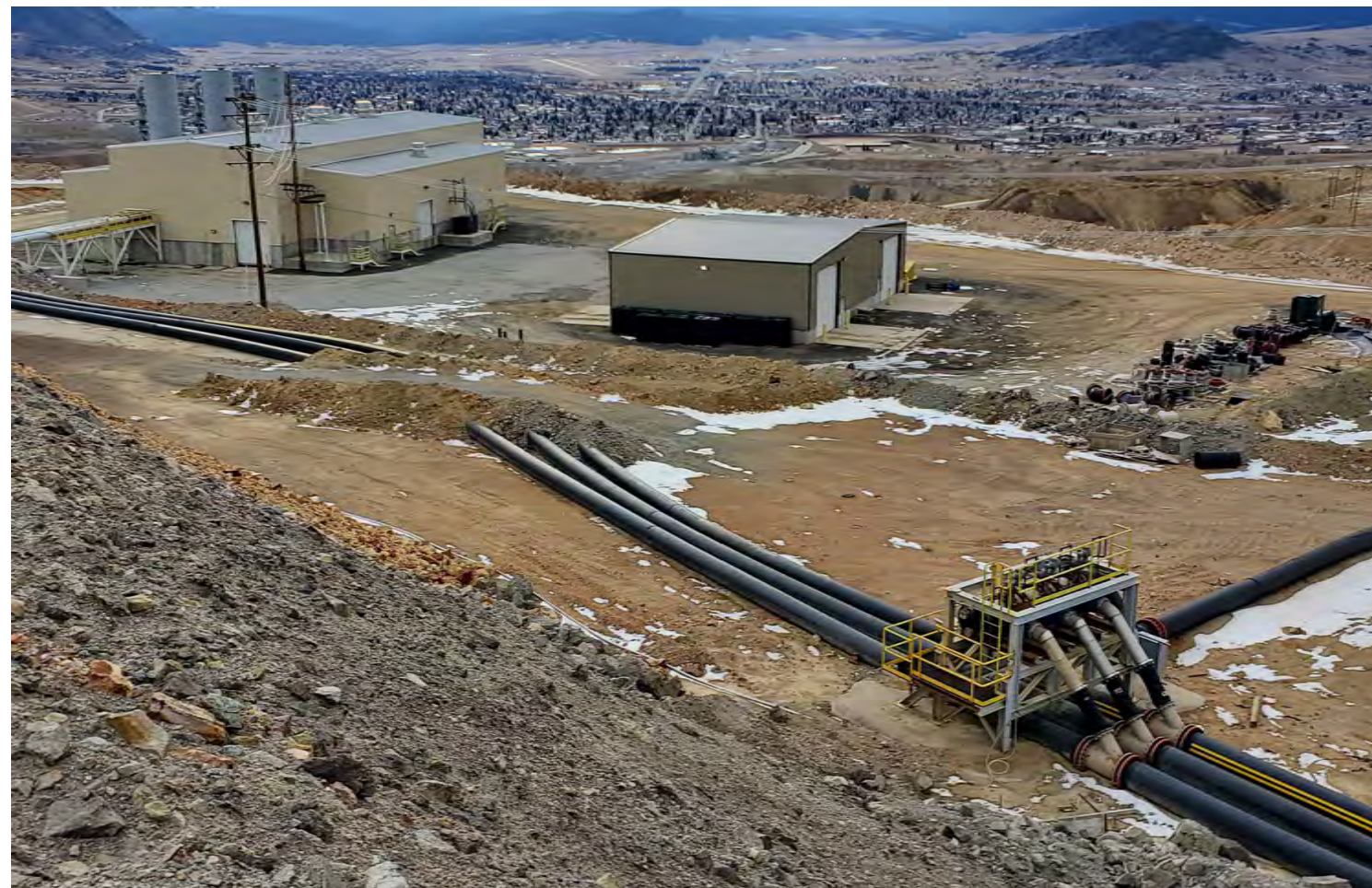
BOOSTER 3 PUMPHOUSE AND HsBCS MANIFOLD
