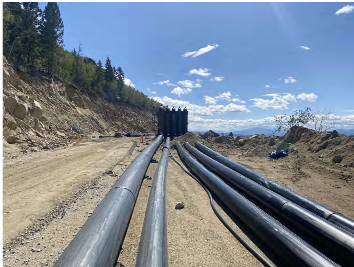
RECLAIM WATER JUNCTION BOX
