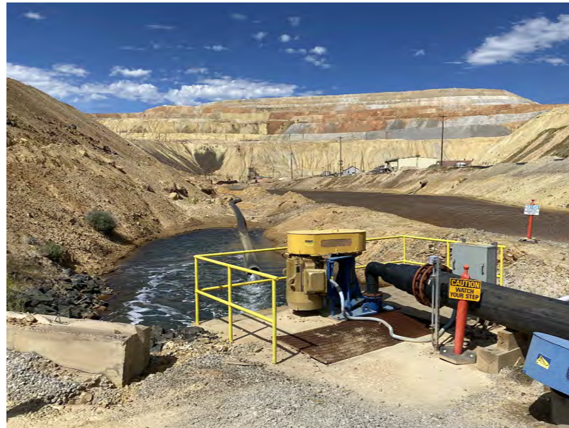
HsBCS TRANSFER POND AND PUMP
