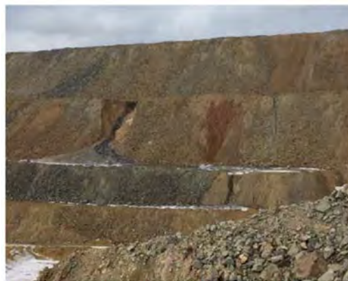
Photo 2. Seepage incident on North-South Embankment reported in 2016 KP EOR report.
