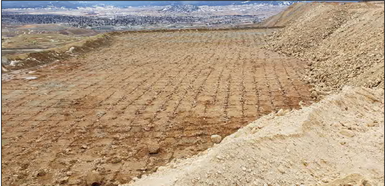
PHOTO 3 – North-South Embankment – Southern extent of 6,350 ft lift surface scarified prior to advancement of the 6,400 ft lift. (March 30, 2020)
