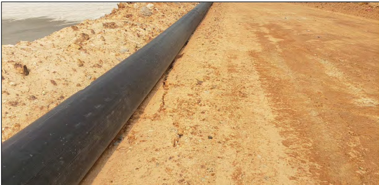
PHOTO 4 – North-South Embankment – Example of cracking along the upstream edge of the tailings discharge corridor
