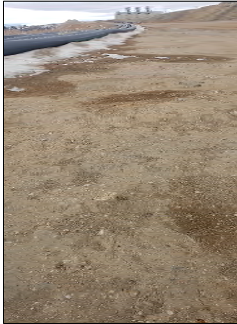
PHOTO 5 – East-West Embankment – Example of settlement cracking along the downstream edge of the tailings pipeline ramp
