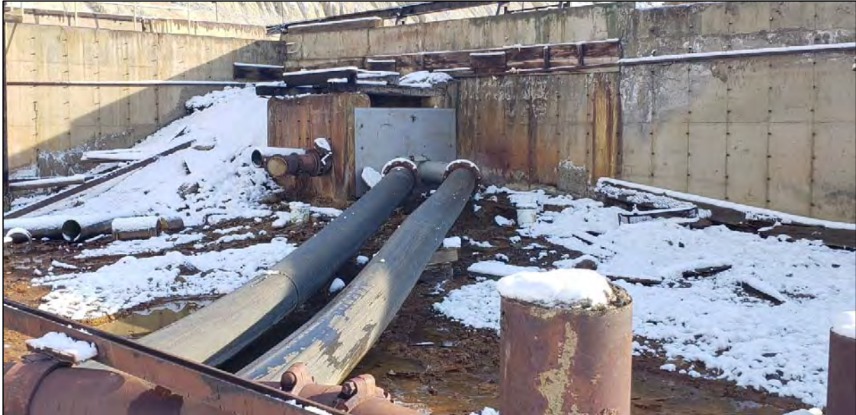
PHOTO 19 – HsB Area – Repair work done to discharge pipe bulkhead exiting #5 and #6 Cells of Precipitation Plant.
