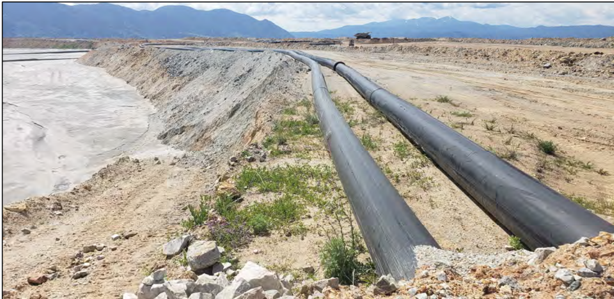
PHOTO 6 – East-West Embankment – Over steepened cut slopes on Terramac access ramp. (June 26, 2020)
