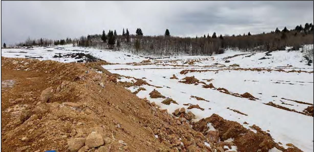
PHOTO 9 – West Embankment – Area above Temporary Extraction Pond filled in with U material, D1 5 ft lifts are planned to be placed in Q2. (March 30, 2020)
