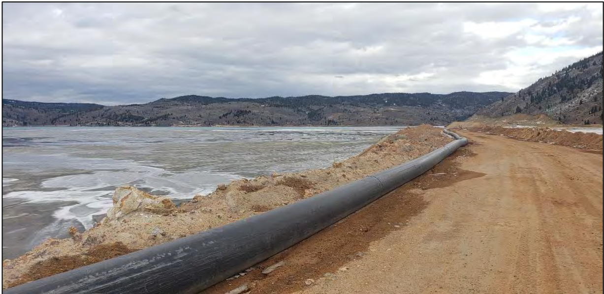
PHOTO 2 – North-South Embankment – Example of minor settlement cracking along the upstream edge of the tailings discharge corridor
