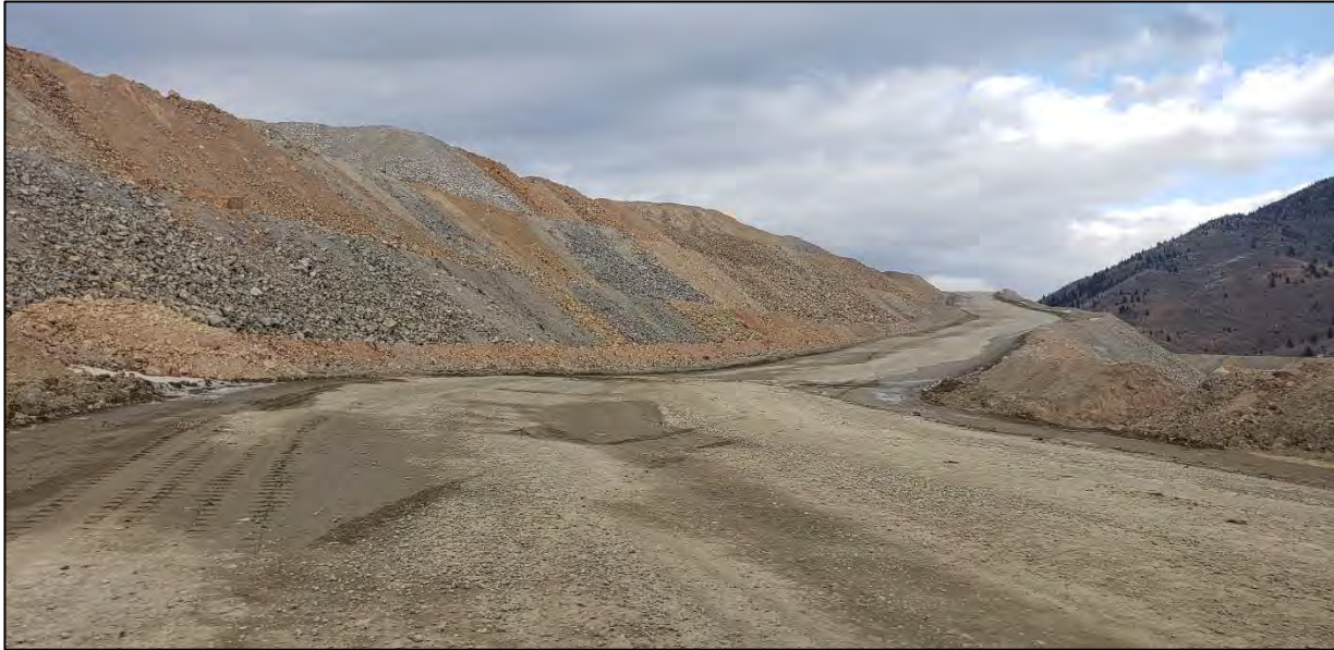
PHOTO 3 – North-South Embankment – Minor depressions in the access ramp
