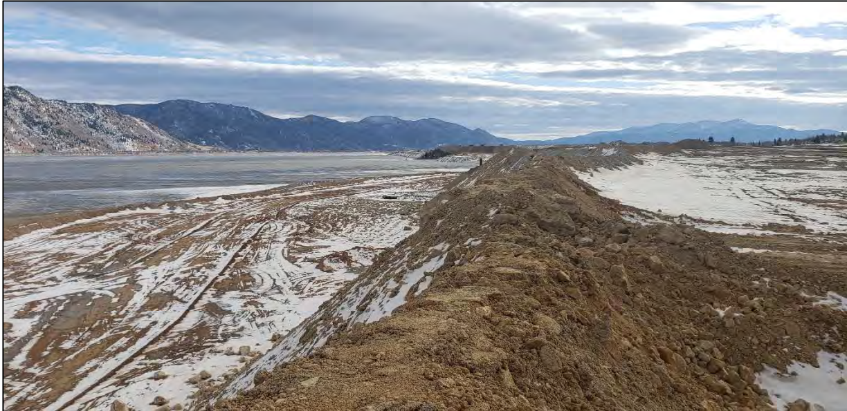
PHOTO 9 West Embankment – El. 6,450 ft construction progress, looking south from the northern end of the embankment
