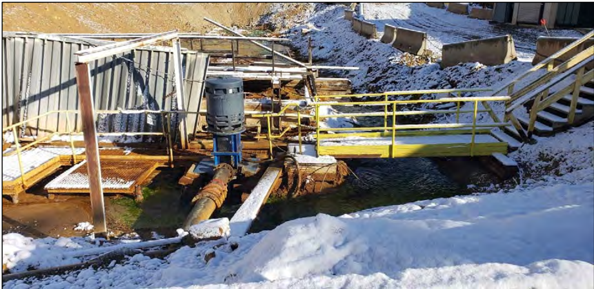
PHOTO 20 – HsB Area – Cell #10 Pump, new pump handling incoming flows, no overflowing water to HsB Lower Pond.
