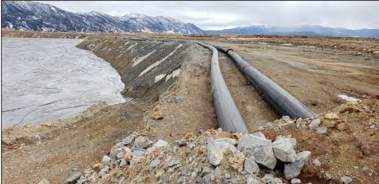
PHOTO 7 – East-West Embankment – Over steepened cut slopes on Terramac access ramp. (March 30, 2020)
