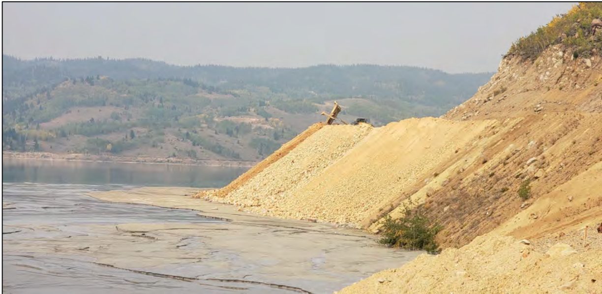
PHOTO 3 – North-South Embankment – Road widening to accommodate realignment of the Reclaim Water Pipeline
