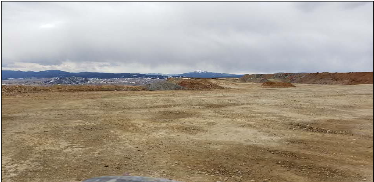
PHOTO 2 – North-South Embankment – Construction of the 6,400 ft lift nearly complete near the southern extent. (March 30, 2020)
