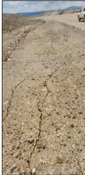
PHOTO 3 – North-South Embankment – Cracking along the downstream edge of the EL. 6,400 ft lift. (June 26, 2020)
