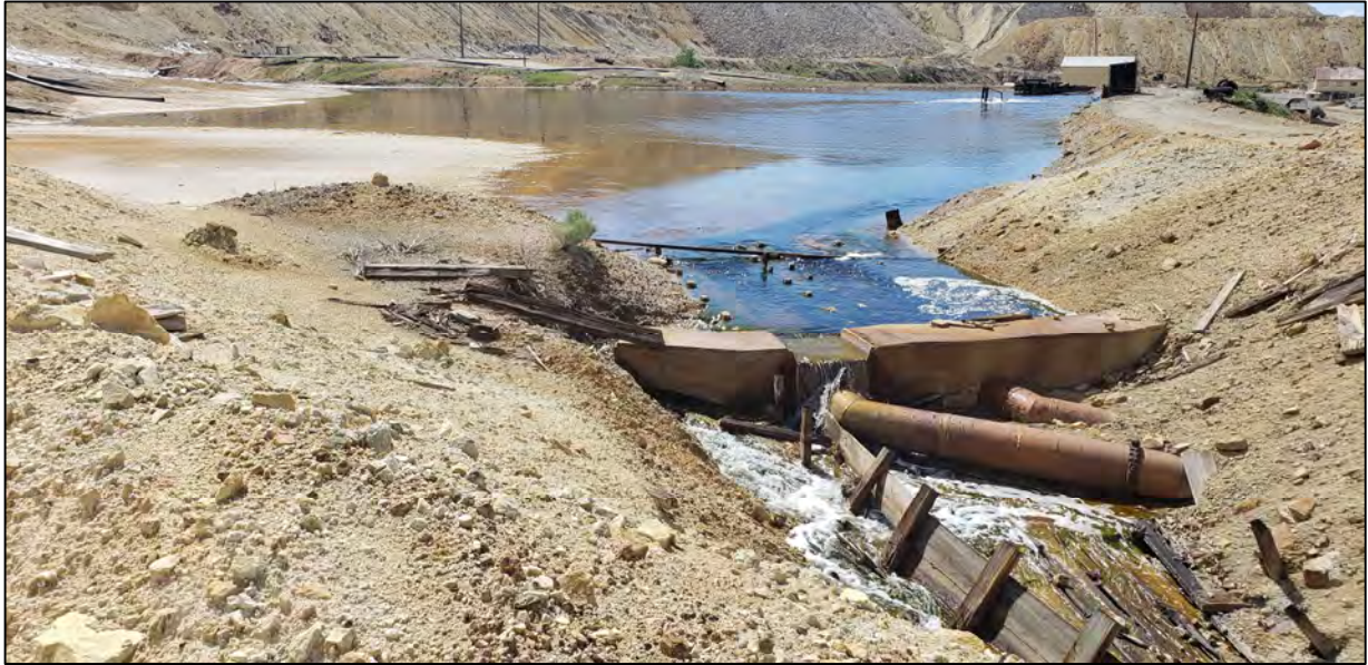
PHOTO 19 – HsB Area – Surge Pond overflow. (June 26, 2020)
