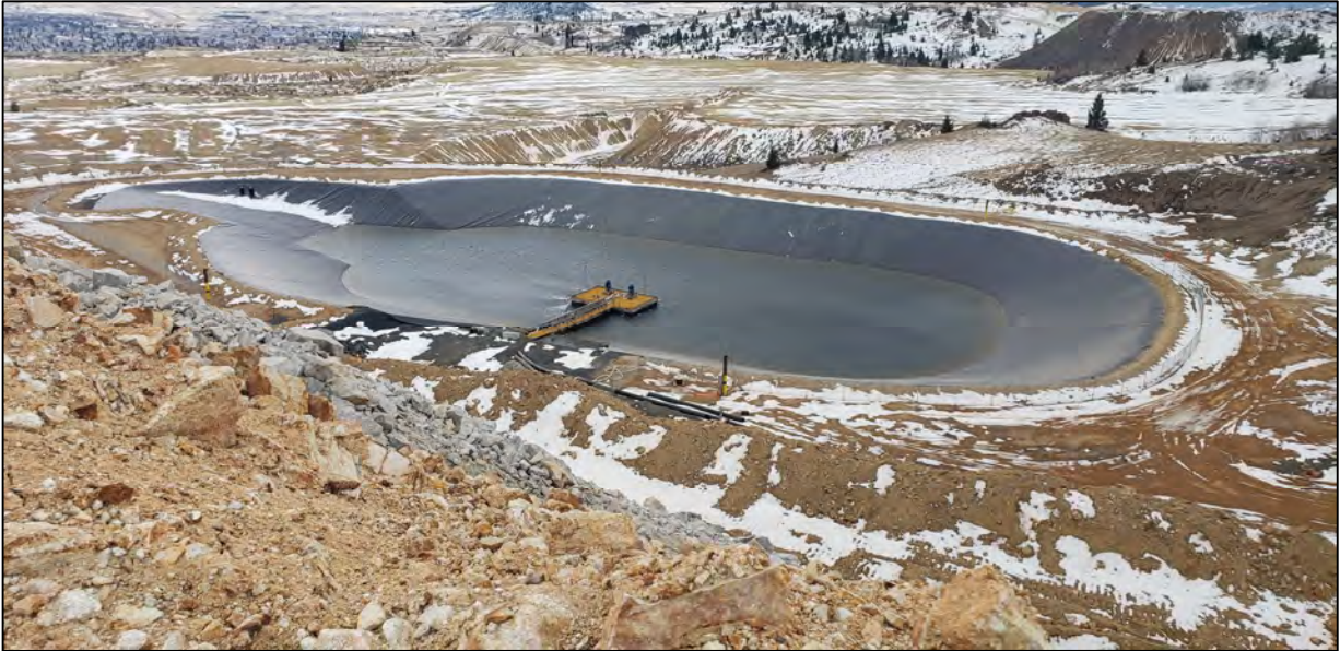
PHOTO 7 – Dec 9, 2020 – WED Extraction Pond and Dewatering System.
