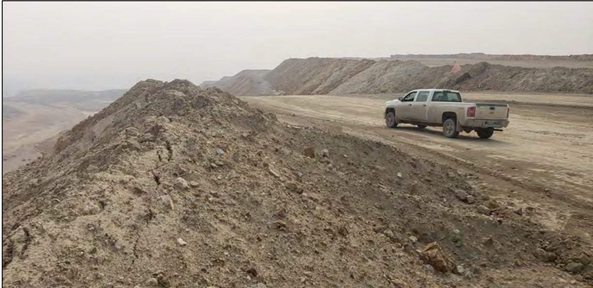
PHOTO 5 – North-South Embankment – Downstream edge of Haul Ramp showing minor settlement cracking along EL 6,400 lift
