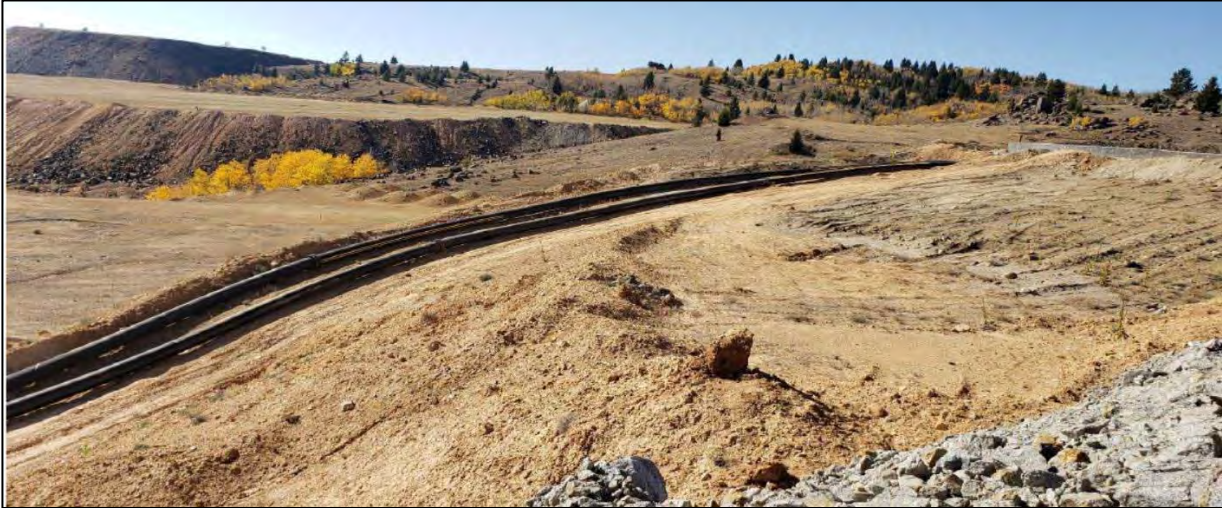
PHOTO 11 – West Embankment – Extraction Pond emergency overflow pipes fused
