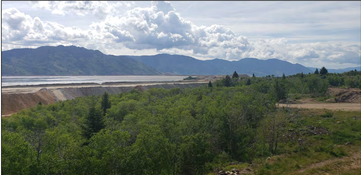
PHOTO 9 – West Embankment – Overview from the West Ridge Topsoil Stockpile showing EL. 6,450 ft. construction progress. (June 26, 2020)
