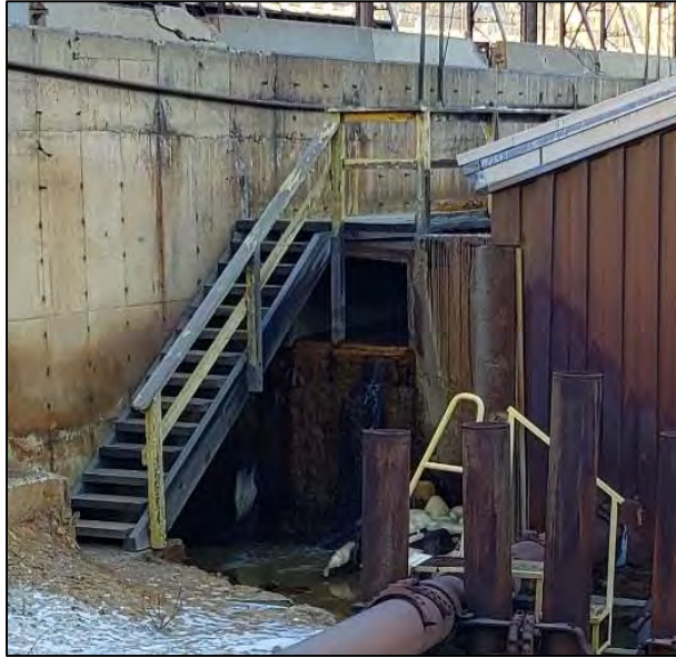
PHOTO 5 – Dec 10, 2020 – Close-up of overflowing head tank at the Precipitation Plant Recirculation Pump House.
