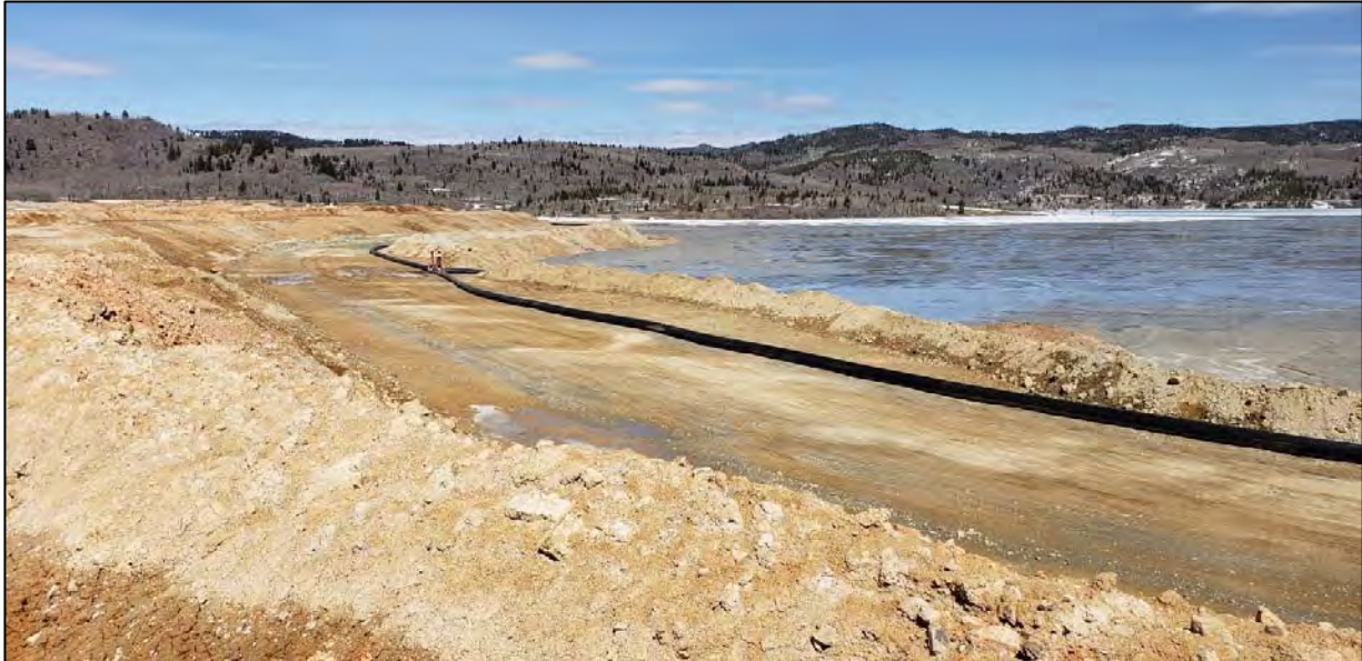
PHOTO 13 – West Embankment – Completed Pipe Bench Raise of Tailings Line #1 and Discharge Point RK-2 in use. (April 10, 2020)
