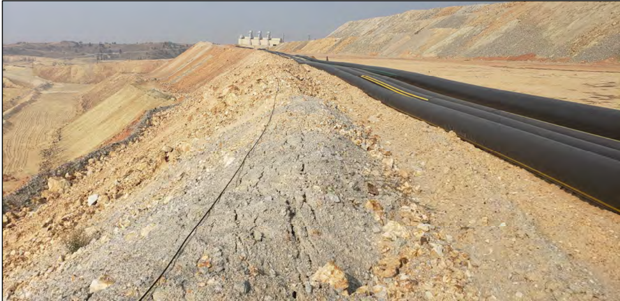
PHOTO 7 – East-West Embankment – Downstream edge of pipeline ramp showing minor settlement cracking
