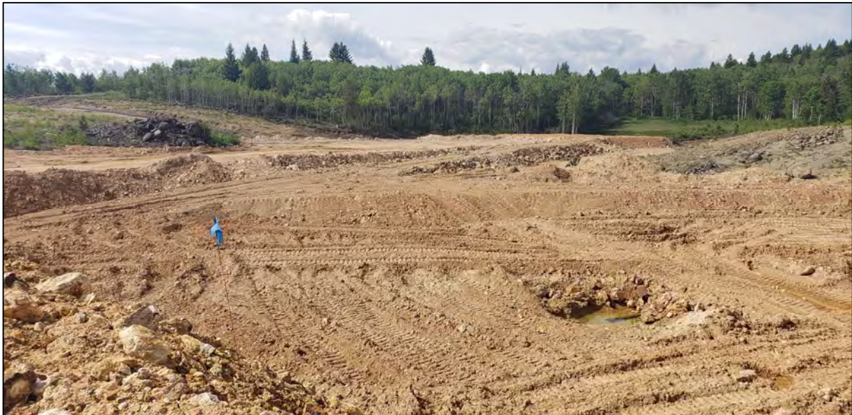
PHOTO 10 – West Embankment – EL. 6,405 ft. Zone D1 Material near Temporary Extraction Pond. (June 26, 2020)
