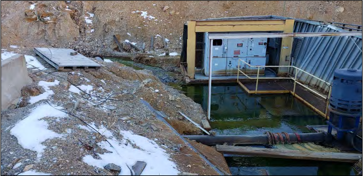
PHOTO 15 – Cell #10 Pump – Overflow to HsB Pond
