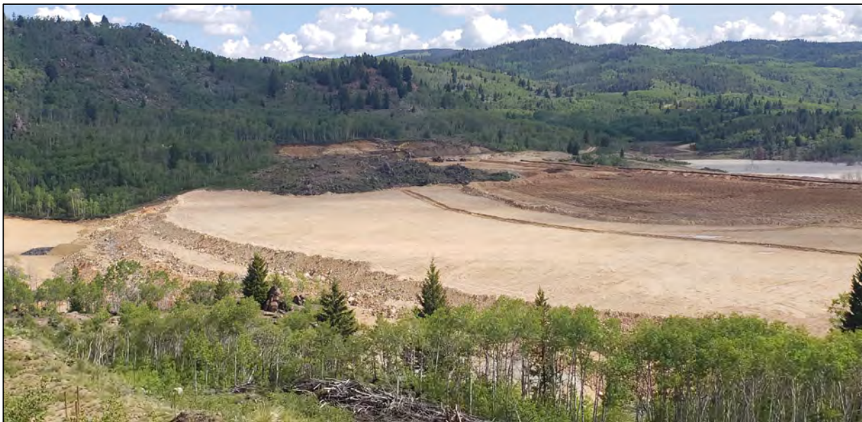
PHOTO 8 – West Embankment – Surface preparation of the EL. 6,400 ft. lift in advance of EL. 6,450 ft. construction.(June 26, 2020)
