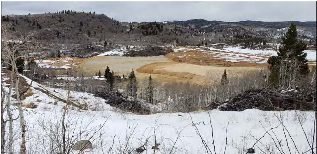
PHOTO 10 – West Embankment – Placement of the 6395 lift of Zone D1 Material near Drain Pod 1 (Bumtown). (March 30, 2020)
