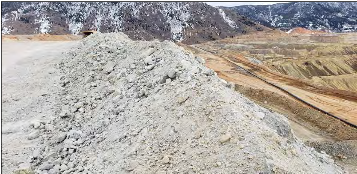
PHOTO 6 – East-West Embankment – New pipe bench and one tailings line moved beyond projected EL. 6,450 ft embankment toe. Additional dozer work needed above Booster Station #2 before remaining pipelines are relocated. (March 30, 2020)
