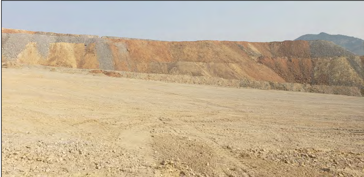
PHOTO 9 – East-West Embankment – Corner to be completed between East-West and North-South Embankments viewed from the haul road
