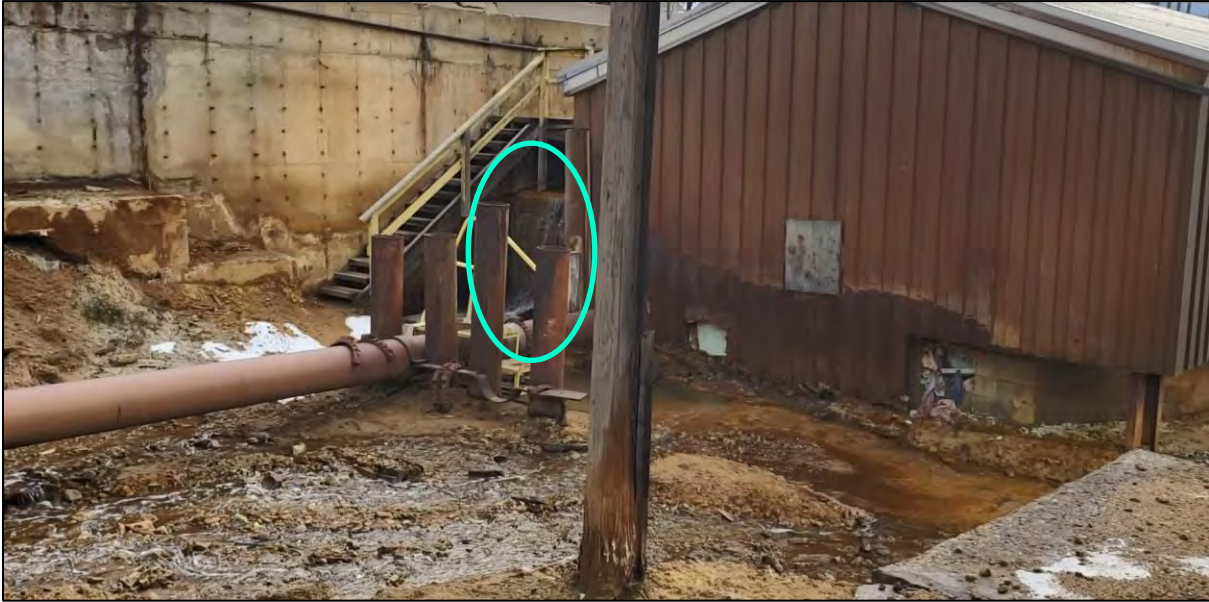
PHOTO 5 – Oct 30, 2020 – Precipitation Plant Recirculation Pump House. Water is overflowing from the head tank under the stairs.
