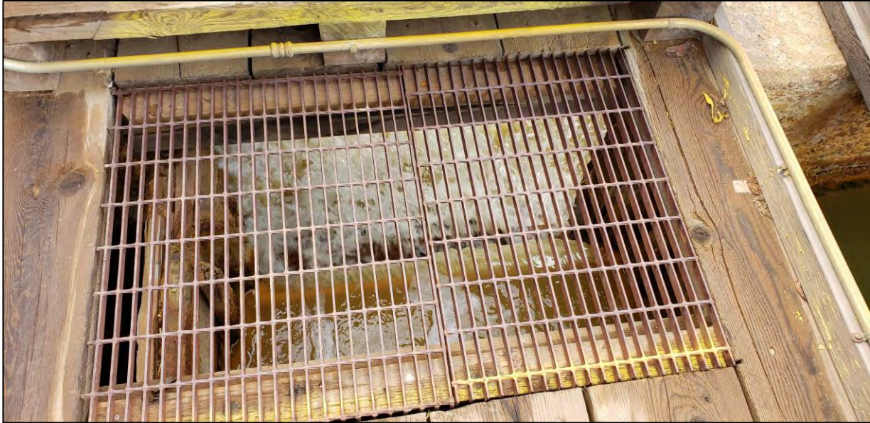
PHOTO 7 – Oct 30, 2020 – Flow through Precipitation Plant overflow weir.
