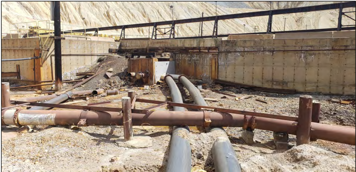
PHOTO 22 – HsB Area – Discharge pipe bulkhead exiting #5 and #6 Cells of Precipitation Plant. (June 26, 2020)
