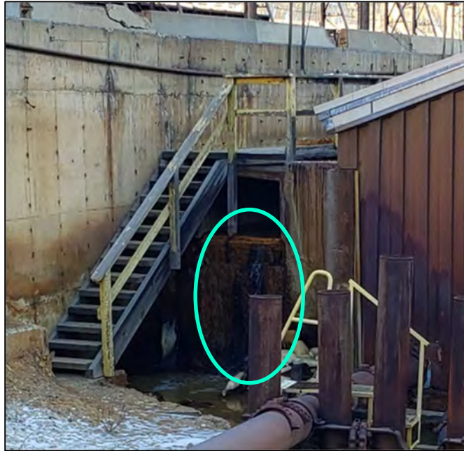
Photo 7.2 Precipitation Plant Recirculation Pump House - water is overflowing from the head tank under the stairs (Dec 10, 2020).
