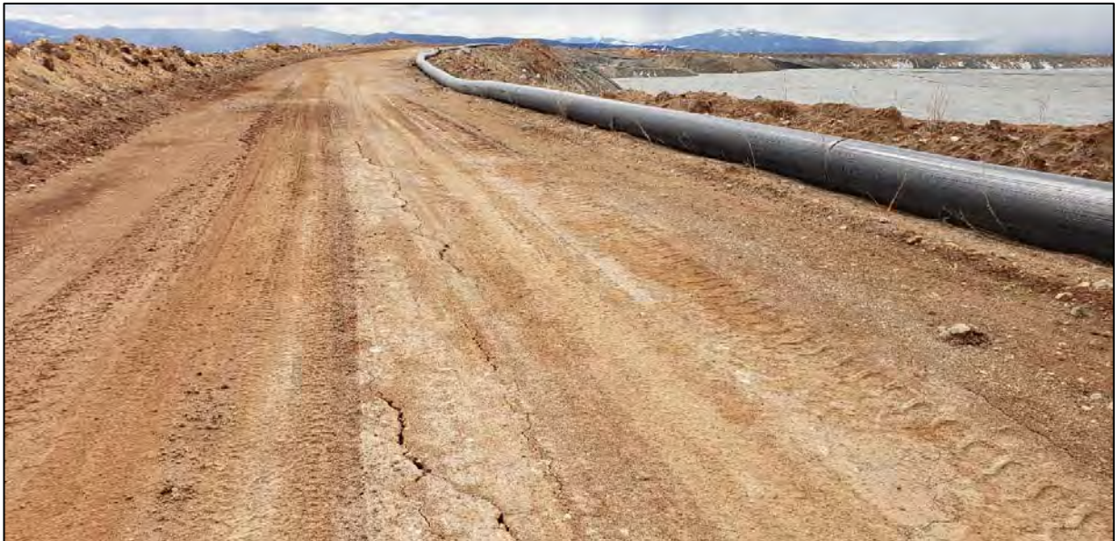
PHOTO 4 – North-South Embankment – Dormant cracking along the upstream pipe corridor near the NS-2 discharge location. (March 30, 2020)
