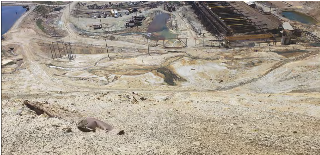
PHOTO 18 – HsB Area – Seeps along toe of East-West Embankment viewed from Seep 10 bench. (June 26, 2020)
