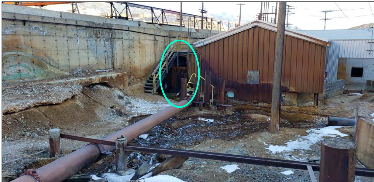
PHOTO 4 – Dec 10, 2020 – Precipitation Plant Recirculation Pump House. Water is overflowing from the head tank under the stairs.
