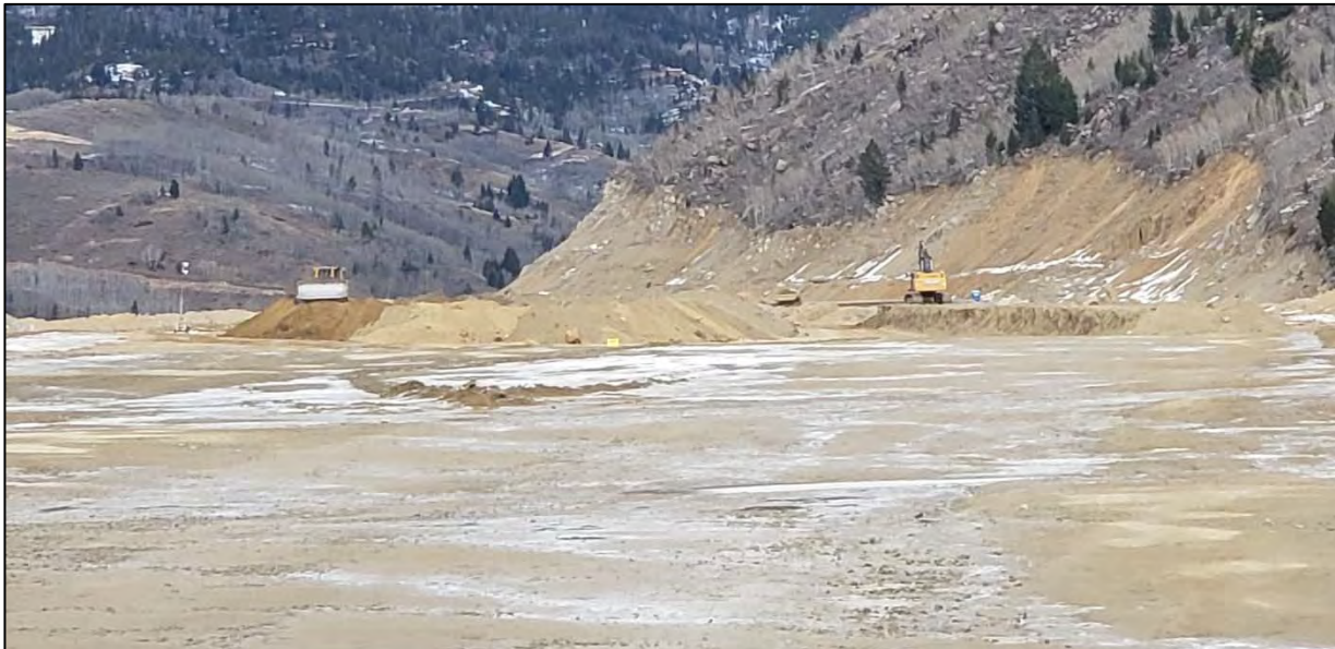
PHOTO 4 – North-South Embankment – Road widening to accommodate realignment of the Reclaim Water Pipeline
