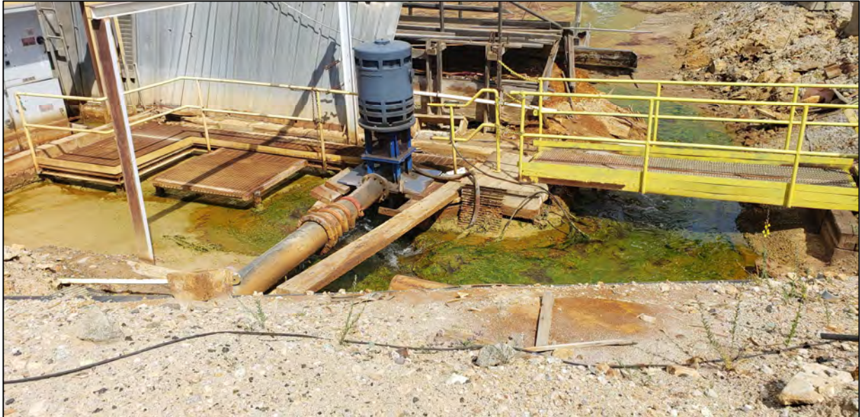
PHOTO 21 – HsB Area – Cell #10 Pump, no overflowing water to HsB Lower Pond. (June 26, 2020)
