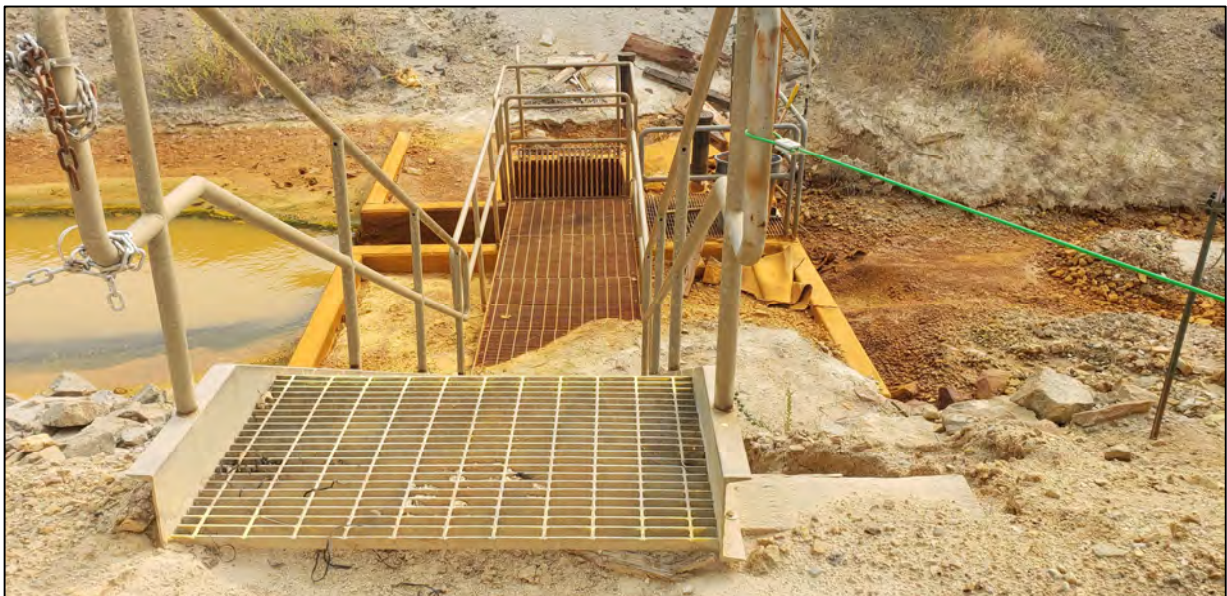
PHOTO 28 – HsB Area – Equalization Basin Intake
