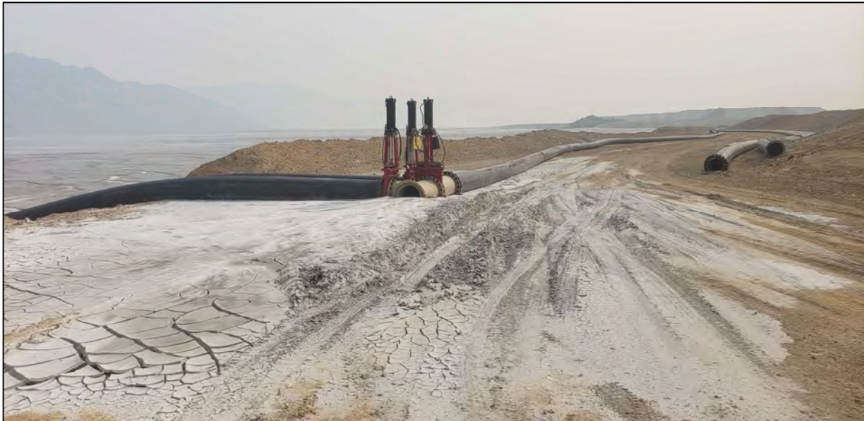
PHOTO 15 – West Embankment – Line 1, Valve 3 disconnected from RK-4 at RK-3 discharge location
