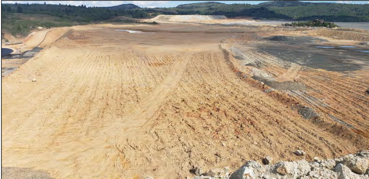
PHOTO 7 – West Embankment – EL. 6,400 ft surface scarified prior to EL. 6,450 ft lift placement (June 26, 2020)
