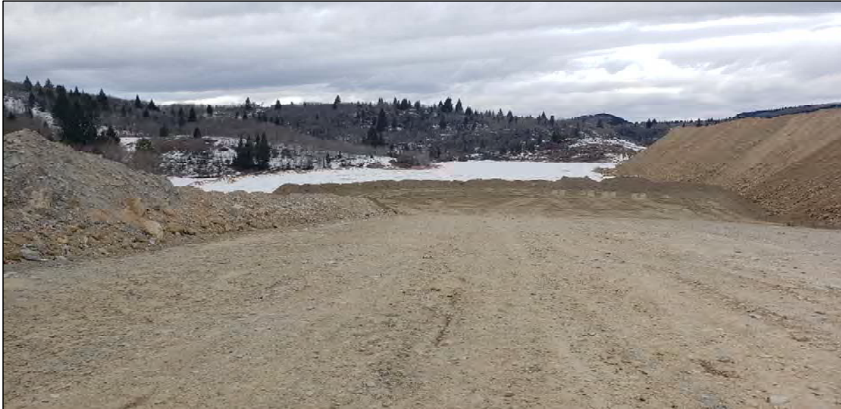
PHOTO 7 – West Embankment – Zone D1 construction west of the Temporary Extraction Pond location
