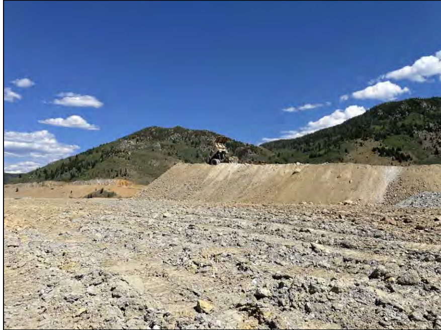
PHOTO 9 – North-South Embankment – EL. 6,450 ft lift subgrade preparation and U material placement, looking northeast
