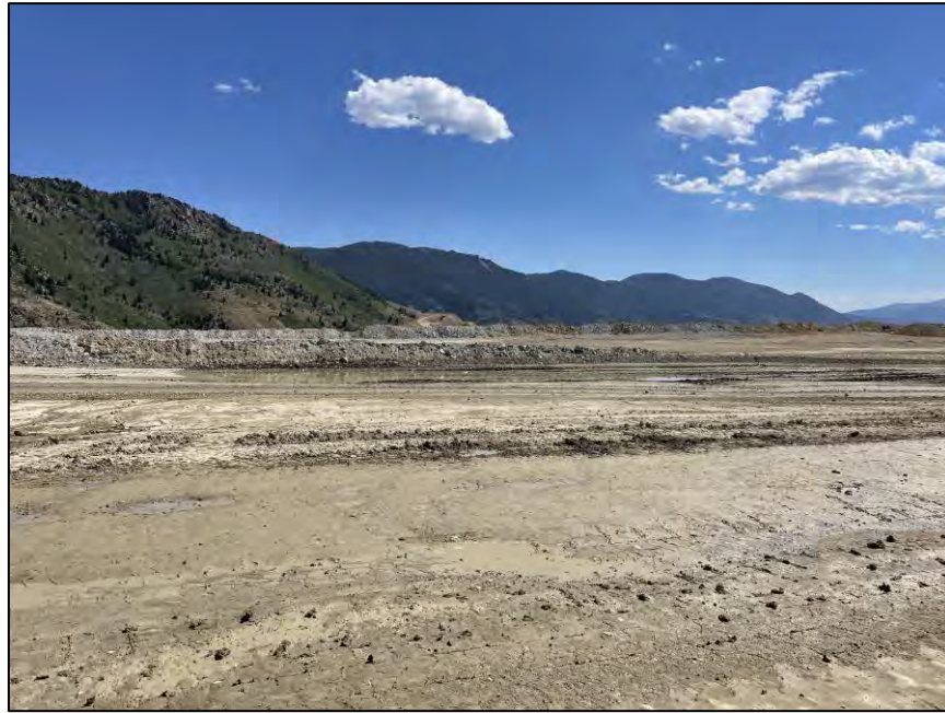
Photo 3.6 EL. 6,450 ft North-South Embankment Crest Depression and Ponding
