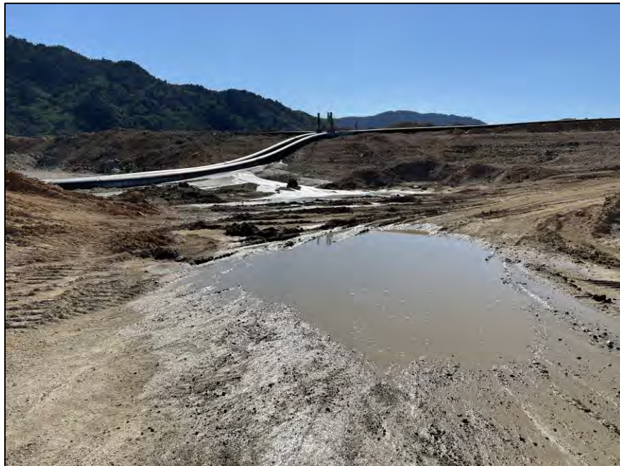
PHOTO 6 – East-West Embankment – Tailings Discharge 3-2 valve leak and pooling
