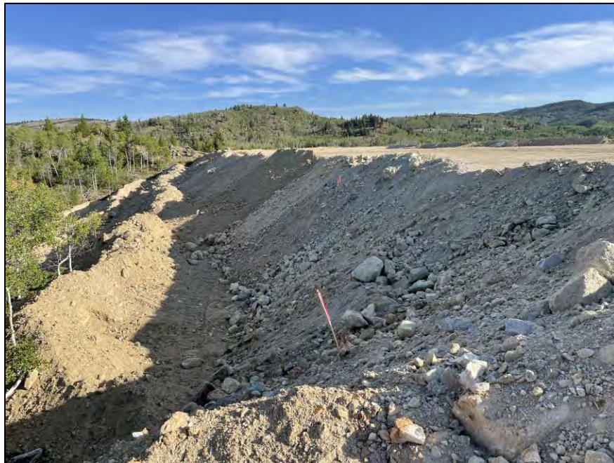
PHOTO 2 – West Embankment – Completed Zone D1 (EL. 6,450 ft) construction north of the Ridge Road
