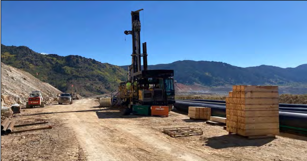
PHOTO 43 – Drill rig for 2022 site investigation program along the East-West Embankment tailings pipeline ramp in the Central Pedestal Area, facing east.
