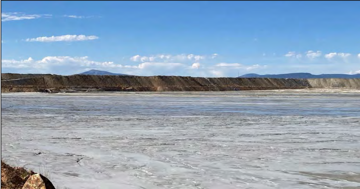
PHOTO 41 – East-West Embankment EL. 6,450 ft surcharge zone upstream shell and adjacent tailings beach in between tailings discharge locations EW-1 and EW-2, facing south from the North-South Embankment.
