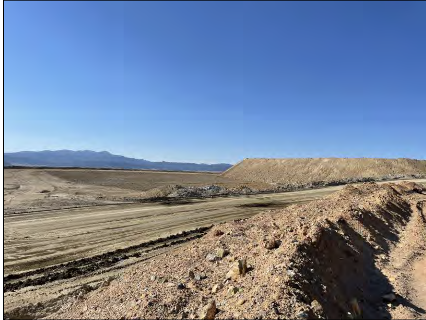
PHOTO 7 – East-West Embankment – EL. 6,450 ft subgrade preparation and U material placement, looking south
