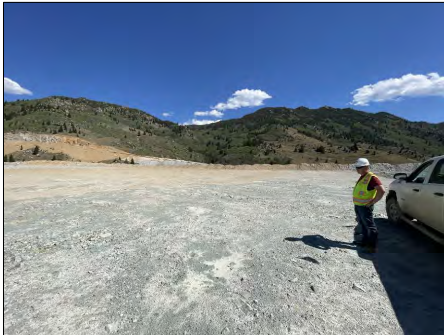
PHOTO 8 – North-South Embankment – EL. 6,400 ft crest in area that underwent CAP recommended re-grading, looking northeast
