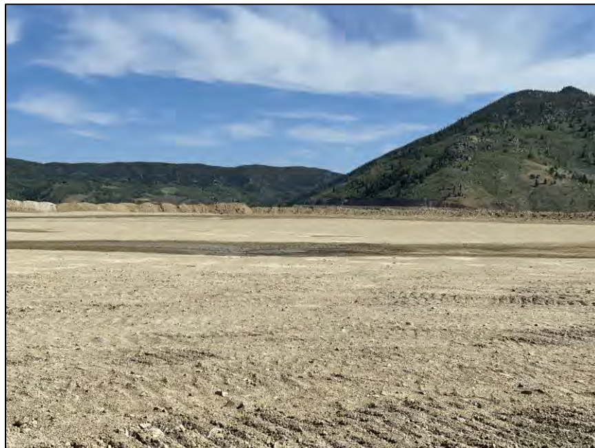
Photo 3.4 EL. 6,450 ft East-West Embankment Crest Depression and Ponding
