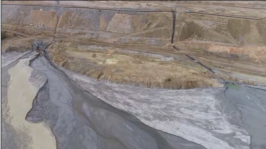
PHOTO 21 –West Embankment upstream interface near Rocky Knob, with view of discharge location RK-1 and an adjacent, recently installed 12” discharge, facing south.
