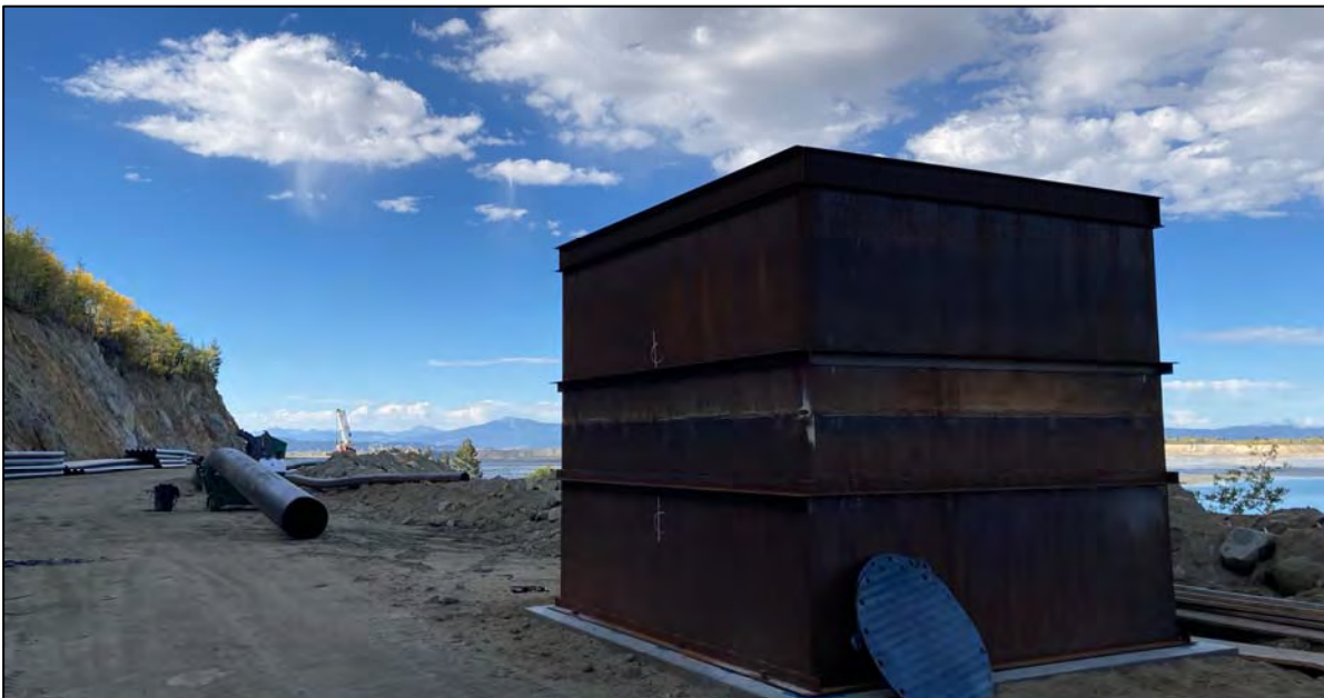
PHOTO 30 – Reclaim Water Pipeline construction, facing south from the New Reclaim Water Pipeline road.
