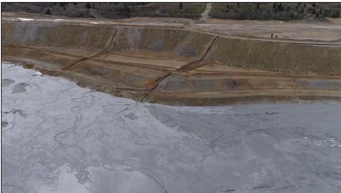
PHOTO 22 – West Embankment upstream interface with view of recently installed 12” discharges between discharge locations RK-2 and RK-3, facing west.
