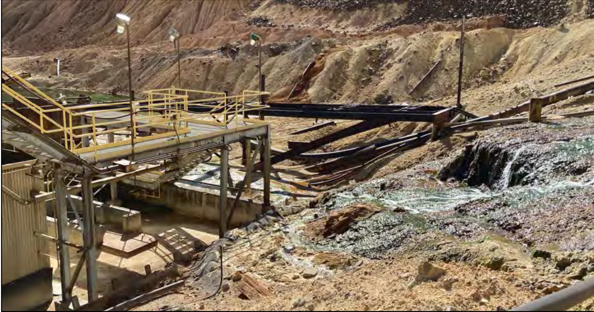
PHOTO 65 – Embankment toe seepage (right) flowing into Upper HsB Pond, facing west.
