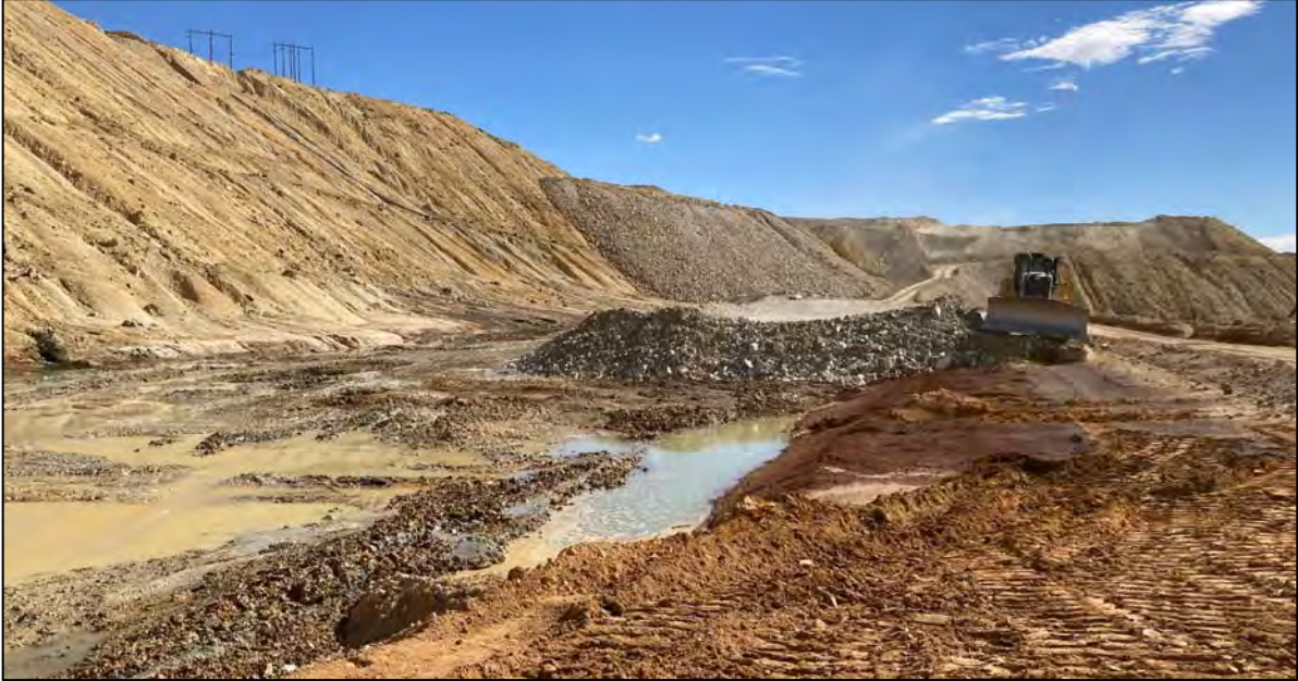
PHOTO 57 – UF – Foundation Layer material placement over the Holding Pond in the HsB Area, facing south.
