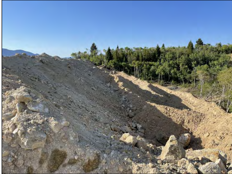
PHOTO 3 – West Embankment – Completed Zone D1 (EL. 6,450 ft) construction south of the Ridge Road
