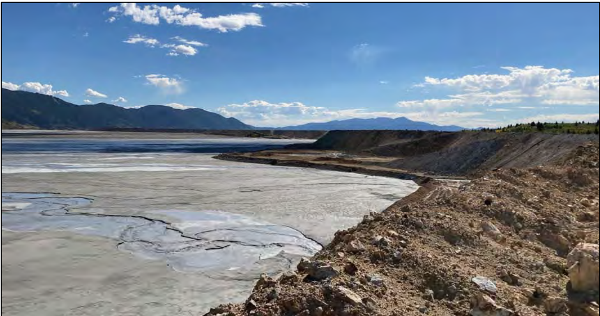
PHOTO 52 – West Embankment upstream shell (right) and tailings beach (left) by tailings discharge location RK-3, facing southeast from EL. 6,450 ft.
