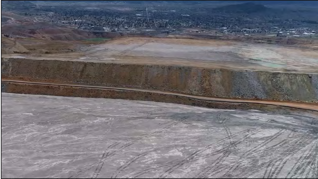
PHOTO 15 – Upstream interface of East-West Embankment, in between NS-1 and EW-1, and EL. 6,450 ft lift and rockfill surcharge placement progress, looking south.
