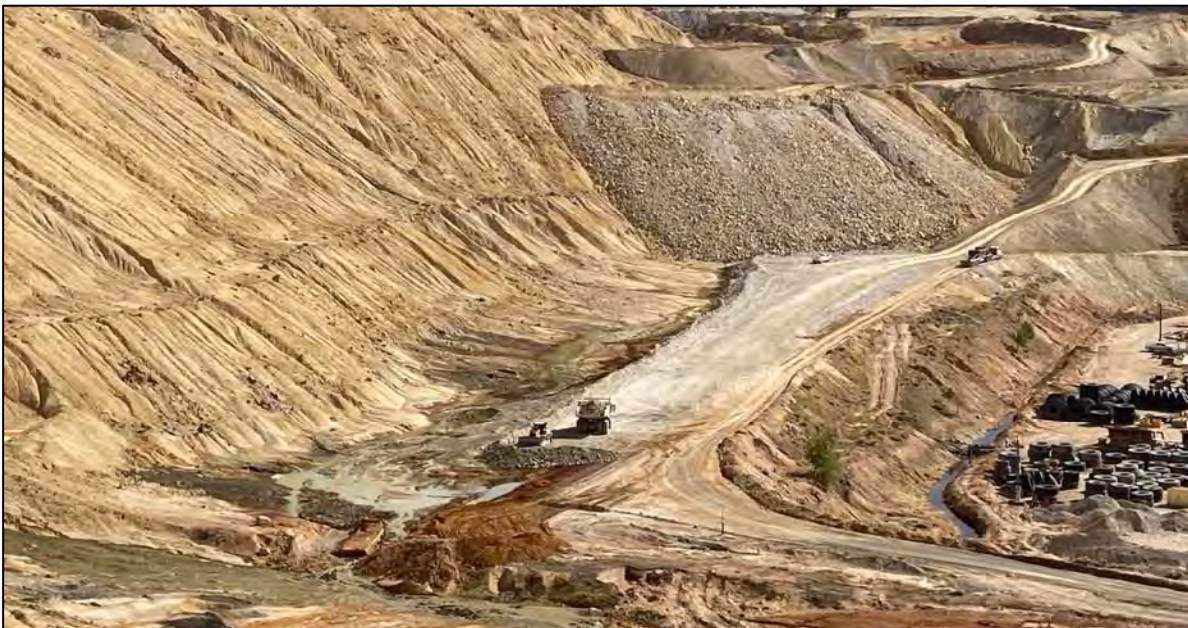
PHOTO 56 – UF – Foundation Layer material placement over the Holding Pond in the HsB Area, facing southeast.
