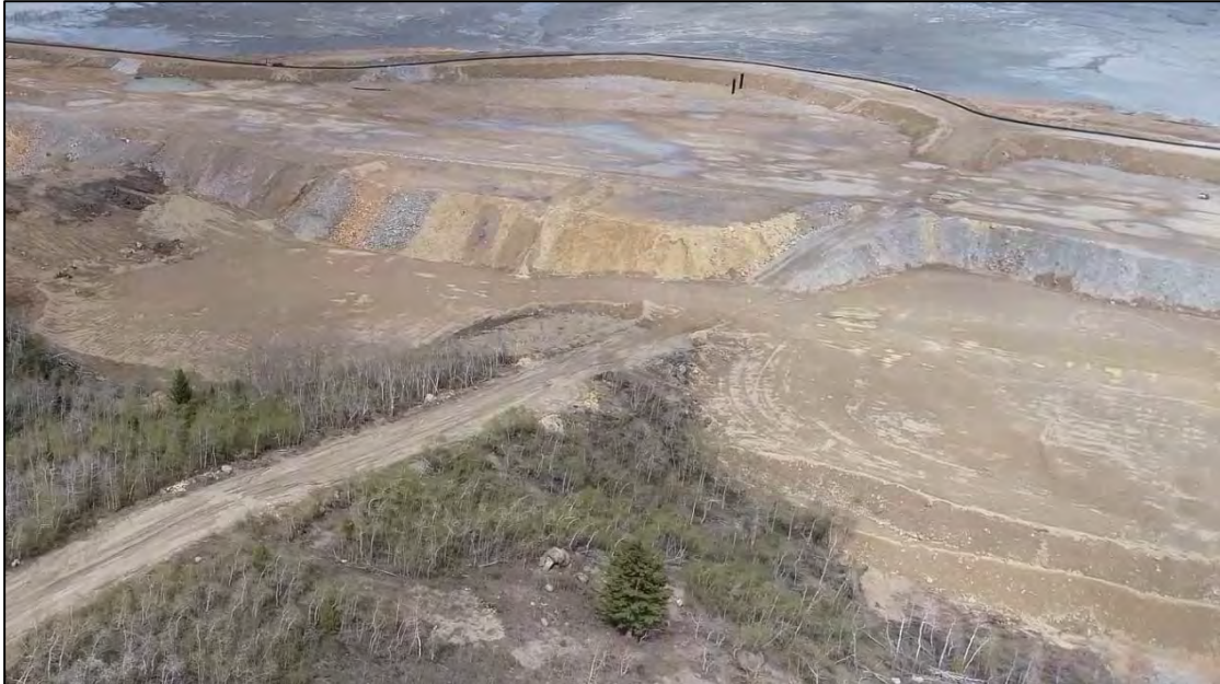
PHOTO 27 – West Embankment D1 – Rockfill material placement progress by Ridge Road, facing east.
