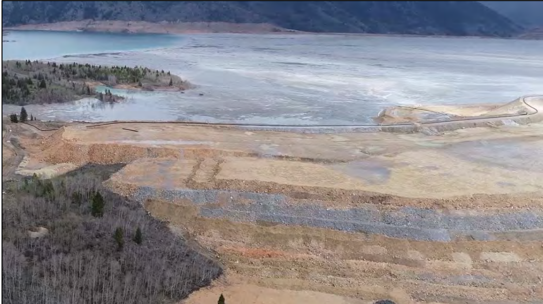
PHOTO 25 – West Embankment crest and downstream shell at northern end of West Embankment, facing east.
