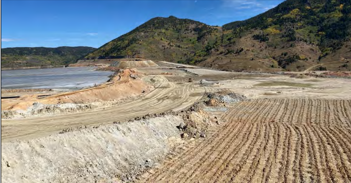
PHOTO 35 – North-South Embankment crest and EL. 6,450 ft lift subgrade preparation, looking north from the North-South Embankment and East-West Embankment tie-in area.
