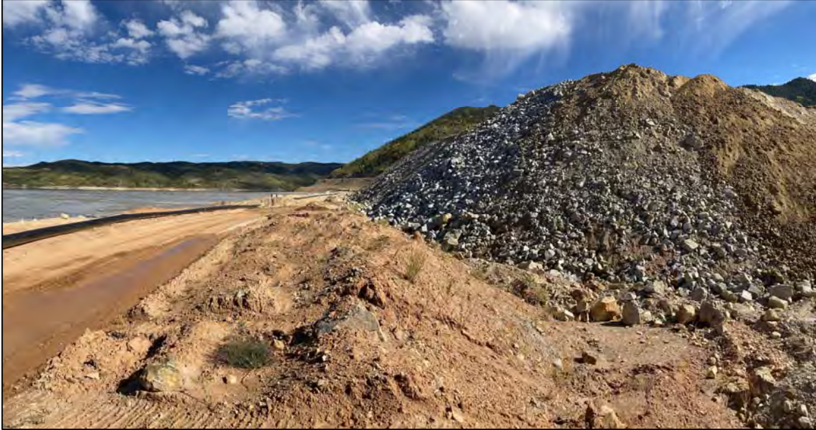
PHOTO 37 – North-South Embankment tailings discharge corridor (left) and EL. 6,450 ft lift placement progress (right), facing north.
