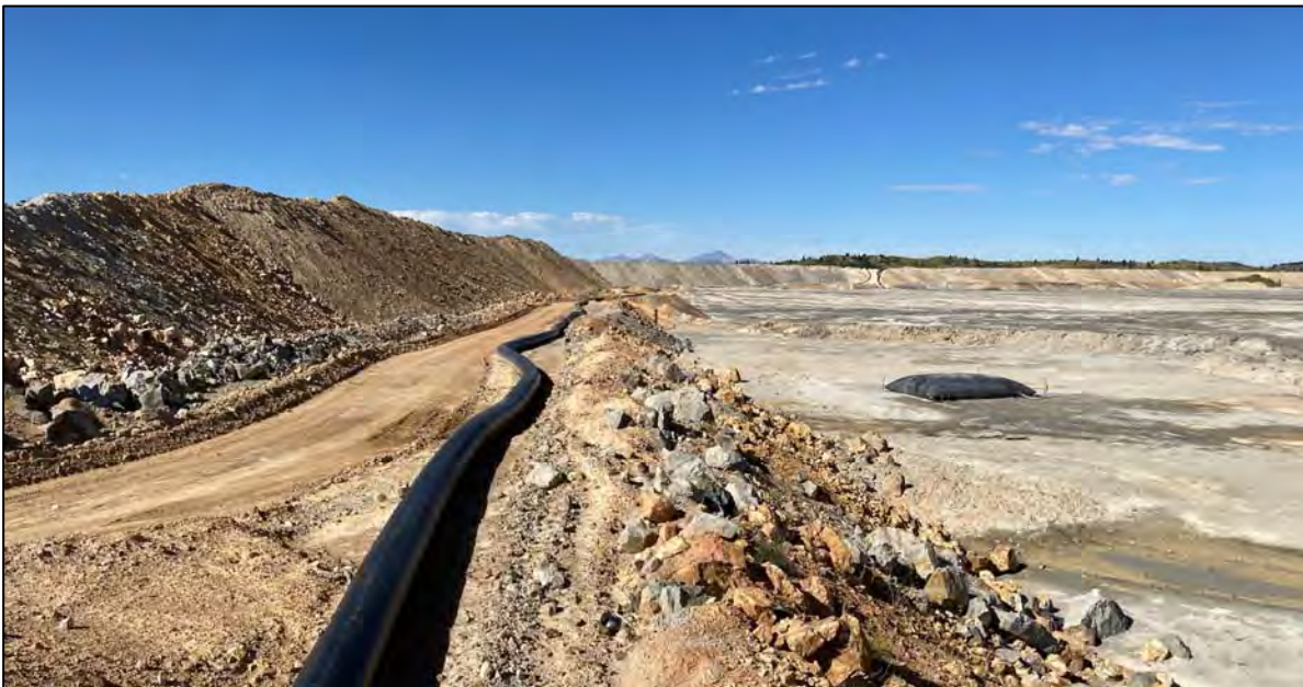
PHOTO 42 – East-West Embankment EL. 6,450 surcharge zone (left), tailings pipeline (middle), and tailings beach (right), facing west from tailings discharge location NS-1 towards EW-2.
