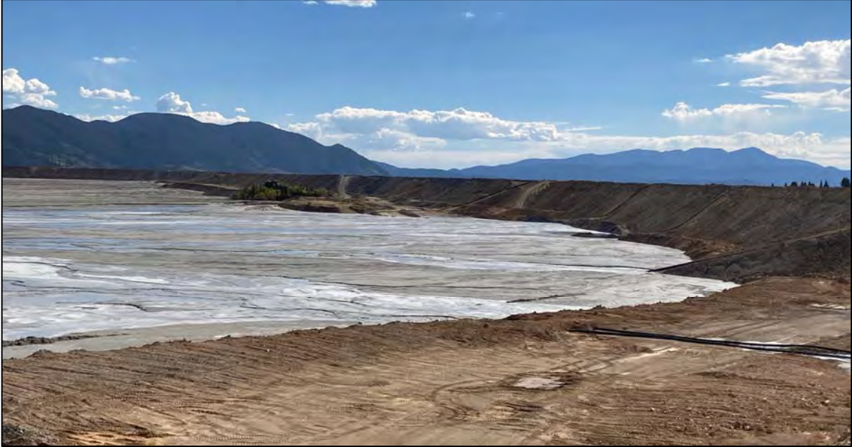
PHOTO 51 – West Embankment upstream shell (right) and tailings beach (left) north of Rocky Knob, facing southeast from EL. 6,450 ft.
