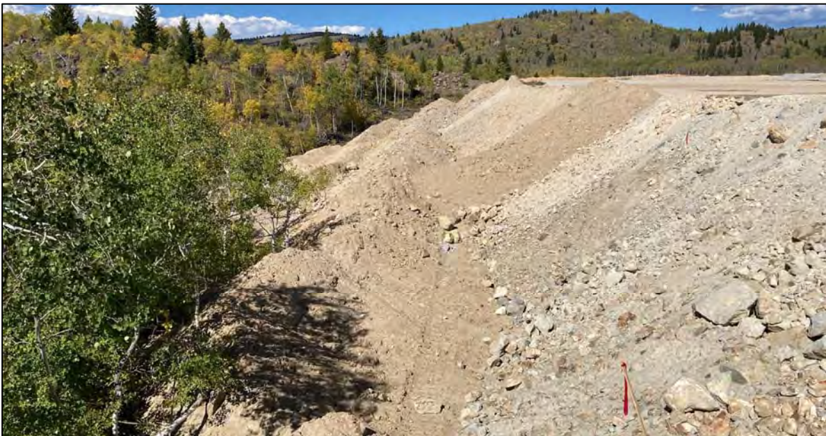
PHOTO 48 – Downstream side of West Embankment south of the Ridge Road. Completed D1 material placement in benches pending final grading and trimming to 3H:1V slope angle, facing north.
