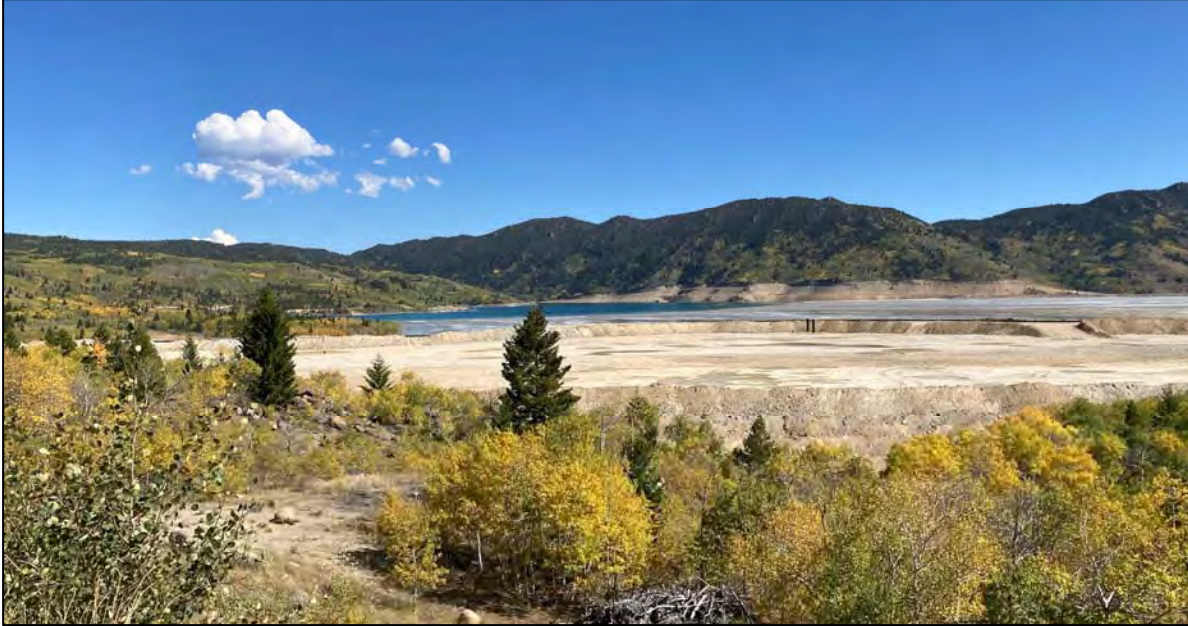
PHOTO 47 – Downstream side of the West Embankment including completed Zone D1 of the downstream shell, facing east from West Ridge topsoil stockpile.
