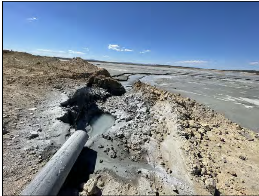
Photo 4.1 Erosion Along Tailings Discharge Corridor Near Section 58+00 N
