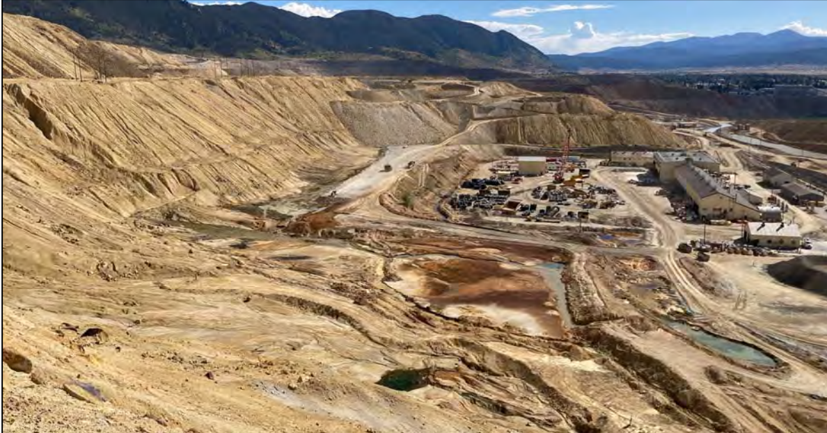
PHOTO 55 – Zone UF construction progress, Holding Pond, and Surge Pond in the HsB Area, facing south from Number 10 Seep Bench.
