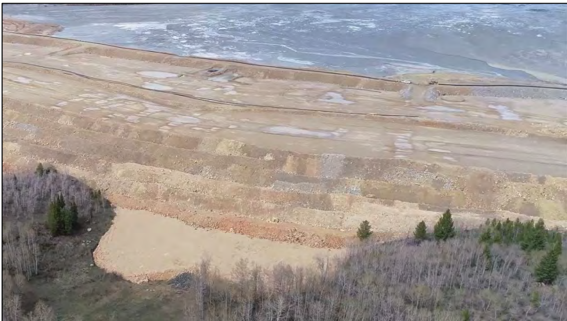
PHOTO 26 – West Embankment downstream shell, northwest of Rocky Knob and Extraction Pond, looking northeast.
