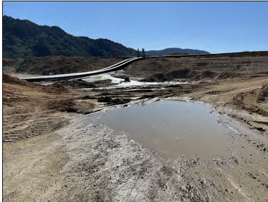
Photo 4.2 Discharge 3-2 Valve Leak and Minor Ponding
