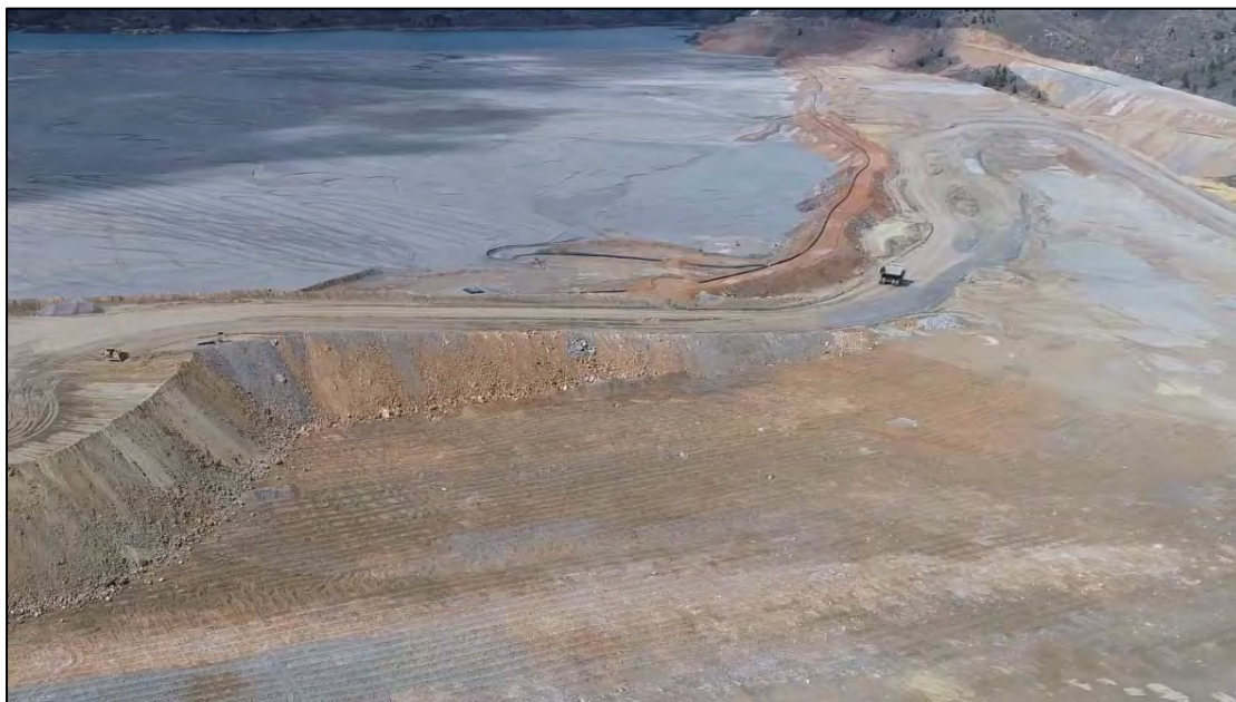
PHOTO 10 – Tailings beach (left), EL. 6,450 ft rockfill surcharge placement progress (left), North-South Embankment crest (right), and subgrade preparation at the North-South Embankment and East-West Embankment tie-in area, facing north.
