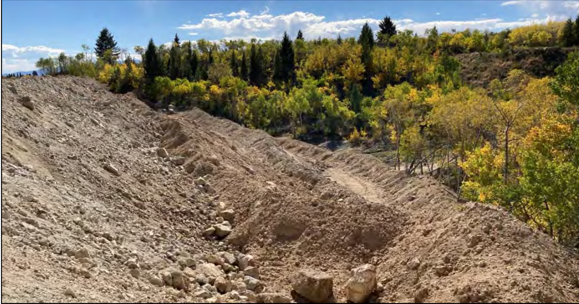
PHOTO 49 – Downstream side of West Embankment south of the Ridge Road. Completed D1 material placement in benches pending final grading and trimming to 3H:1V slope angle, facing north.
