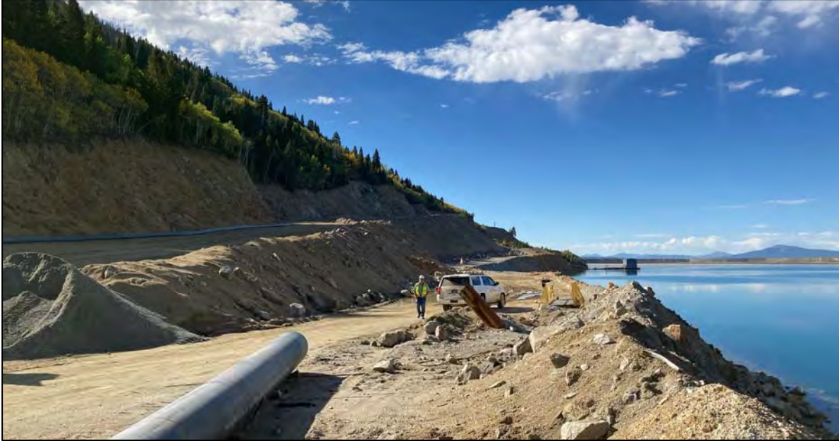
PHOTO 31 – Completed New Reclaim Pipeline road (left) and YDTI supernatant pond (right), facing south.
