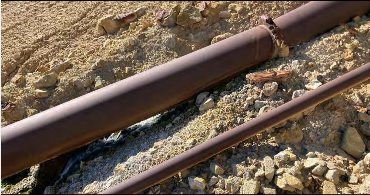
PHOTO 75 – Seep 10 pipeline with observed leak, facing west.
