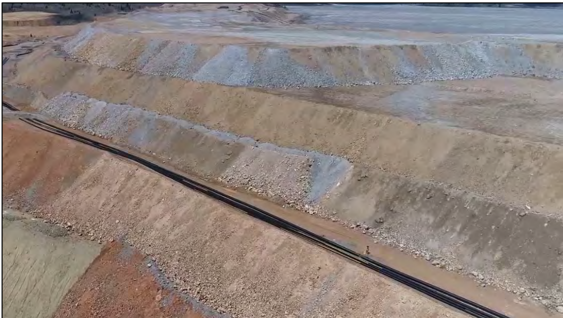
PHOTO 16 – East-West Embankment pipeline ramp and EL. 6,450 ft lift and surcharge zone placement progress, facing northwest from east of No. 3 Booster Pump House.
