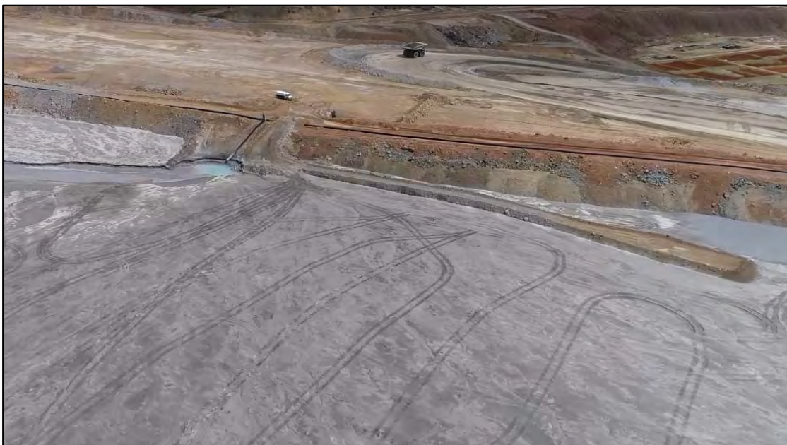
PHOTO 8 – Upstream side of the North-South Embankment by tailings discharge location NS-2, facing east.
