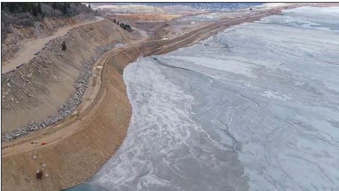
PHOTO 6 – New Reclaim Water Pipeline road, North-South Embankment Crest, and tailings beach, facing south.
