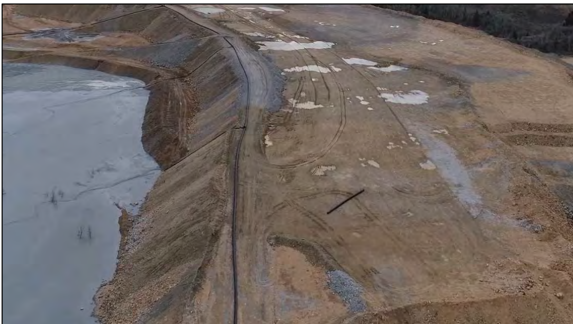
PHOTO 24 – Northern end of West Embankment with view of upstream interface and EL. 6,450 ft crest, facing south near discharge location RK-4.
