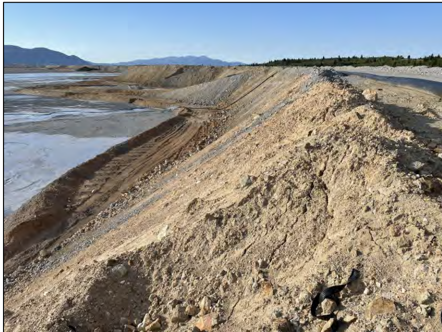
PHOTO 4 – West Embankment – Tailings discharge corridor loosely placed berm cracking
