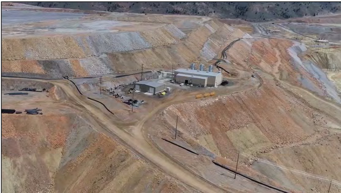
PHOTO 14 – EL. 6,450 ft lift placement progress, No. 3 Booster Pump House, and East-West pipeline ramp in Central Pedestal Area of the East West Embankment, facing east.
