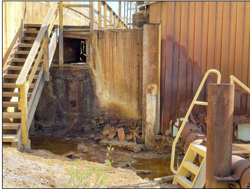
Photo 3.9 Recirculation Pumphouse Head Tank
