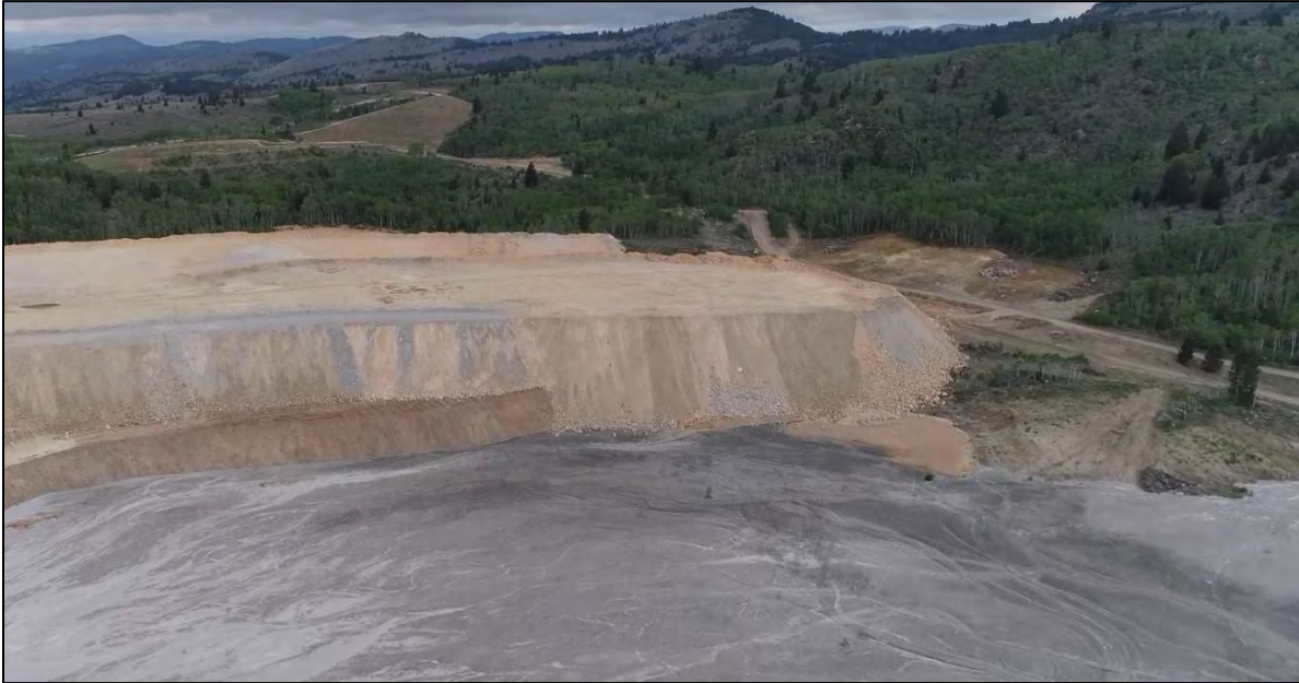
PHOTO 23 – Northern end of West Embankment, upstream interface, looking northwest near decommissioned discharge location RK-4.
