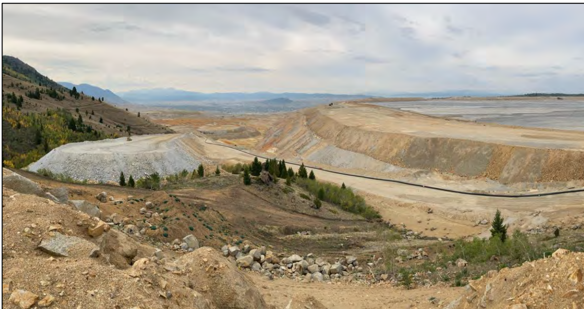
PHOTO 28 – New Reclaim Water Pipeline Ramp (left) and North-South Embankment (right), facing south from New Reclaim Water Pipeline hillside cut.
