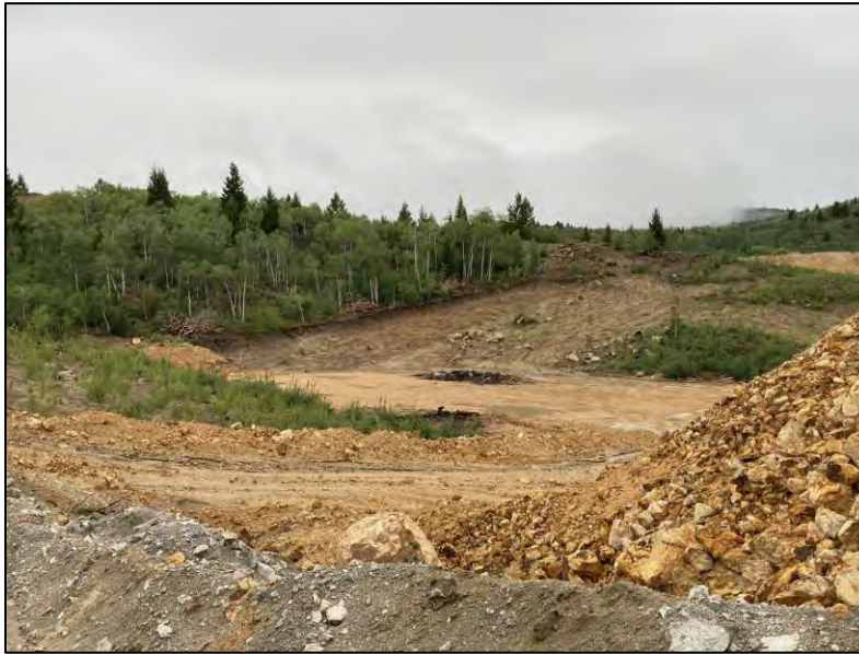
Photo 3.4 Incomplete D1 material placement at Ridge Road facing North
