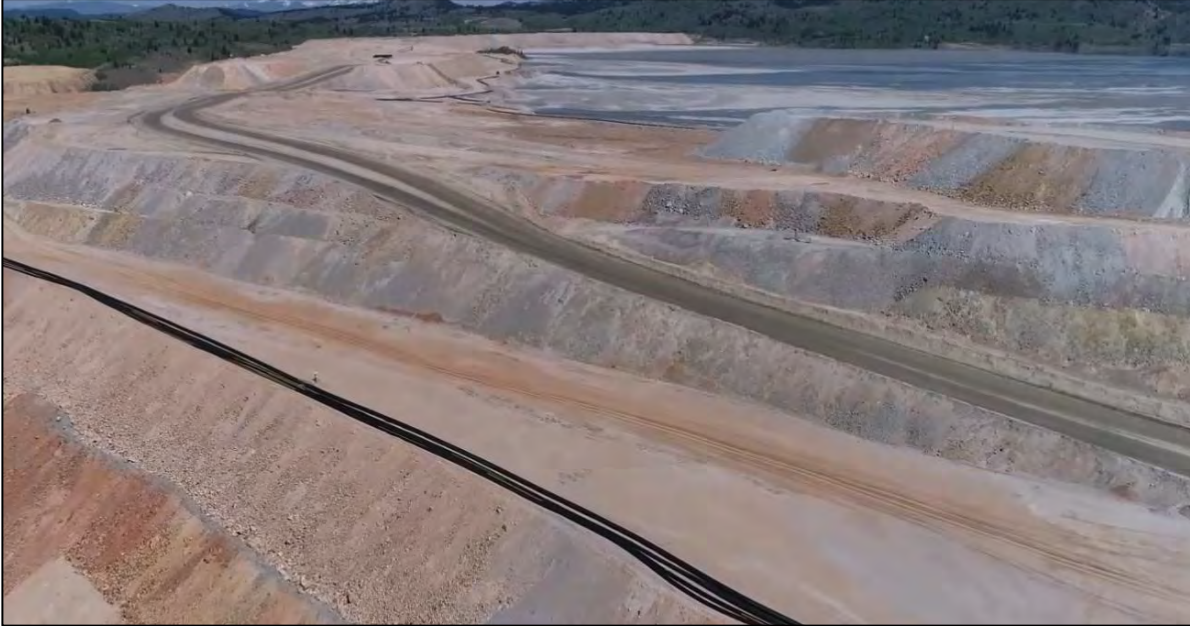
PHOTO 15 – East-West pipeline ramp, decommissioned East-West haul road, EL. 6,450 ft lift (left) and EL. 6,450 surcharge (right), looking north from east of Booster Station #3.
