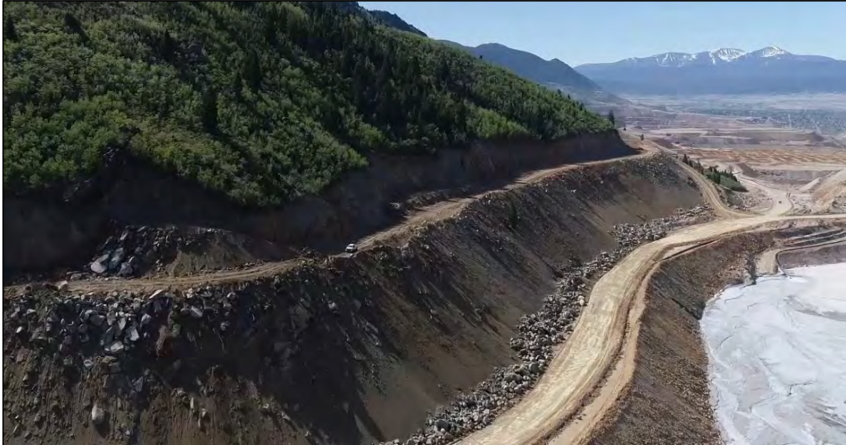
PHOTO 5 – Reclaim water pipeline road and New Reclaim Water Pipeline Ramp cut construction progress, looking south.
