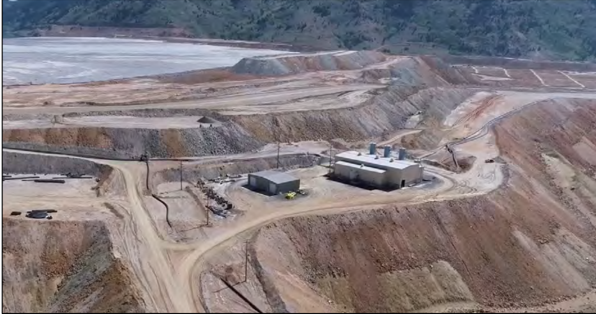
PHOTO 13 – Booster Station #3, East-West pipeline ramp, and EL. 6,450 ft rockfill surcharge in Central Pedestal Area of the East West Embankment, looking northeast.
