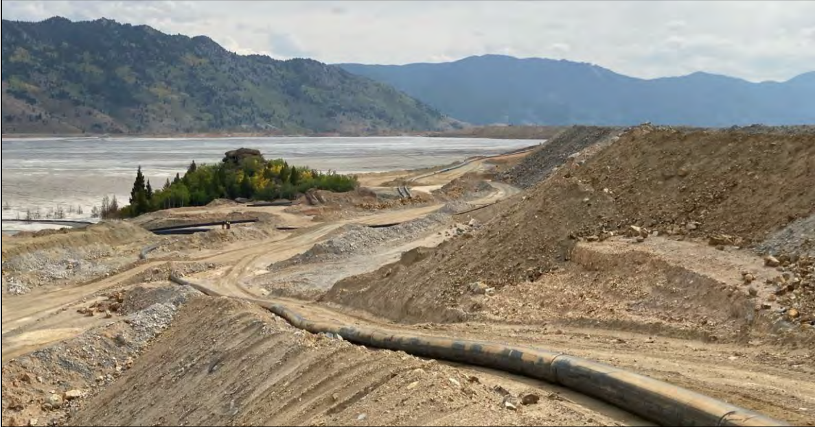
PHOTO 49 – West Embankment upstream side – Tailings discharge location RK-1 by Rocky Knob (left) and EL. 6,450 ft lift (right), facing southeast.
