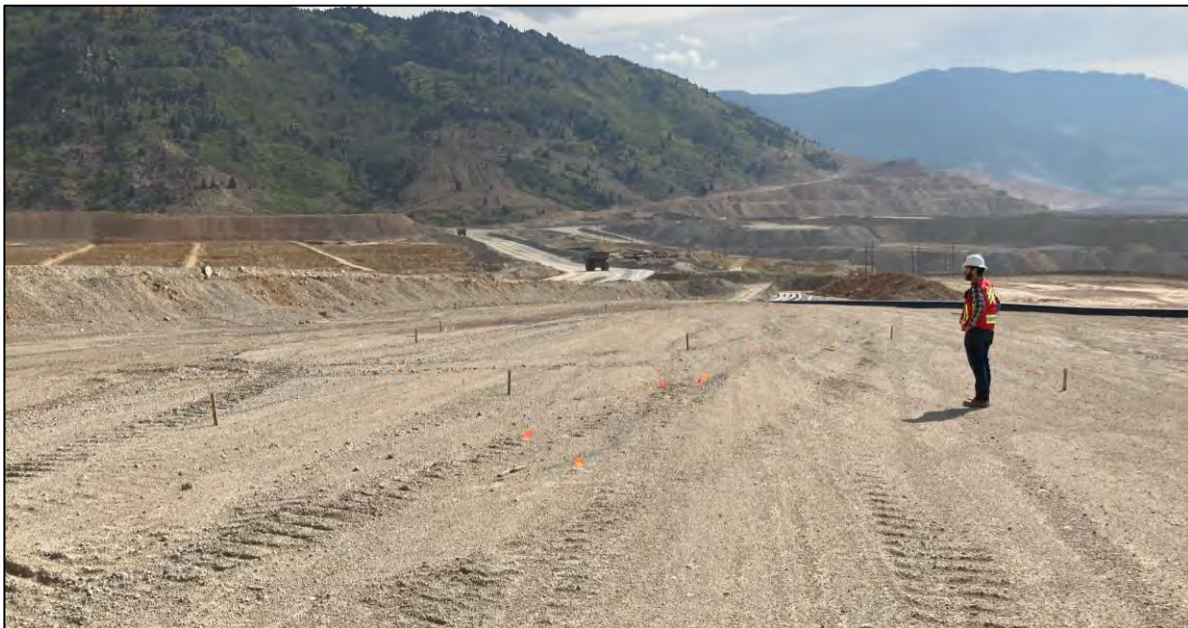
PHOTO 42 – Cracks monitored along the upstream side of the East-West pipeline ramp by the eastern toe of the EL. 6,250 ft lift, facing east.
