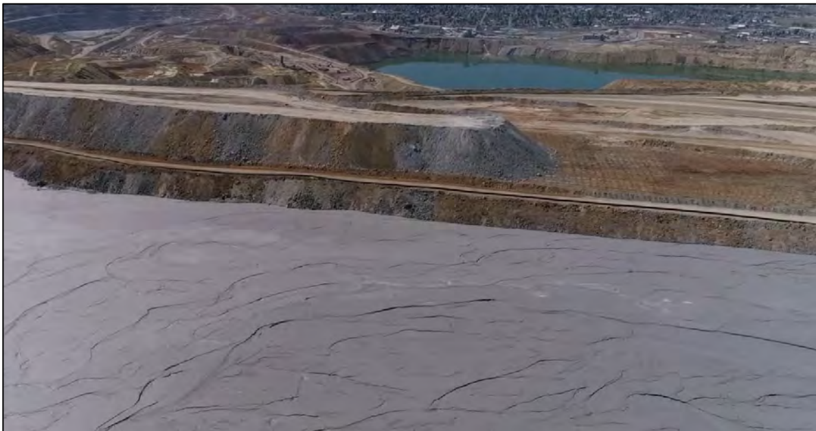
PHOTO 14 – Upstream interface of East-West Embankment, in between NS-1 and EW-1, and EL. 6,450 ft rockfill surcharge construction progress, looking south.
