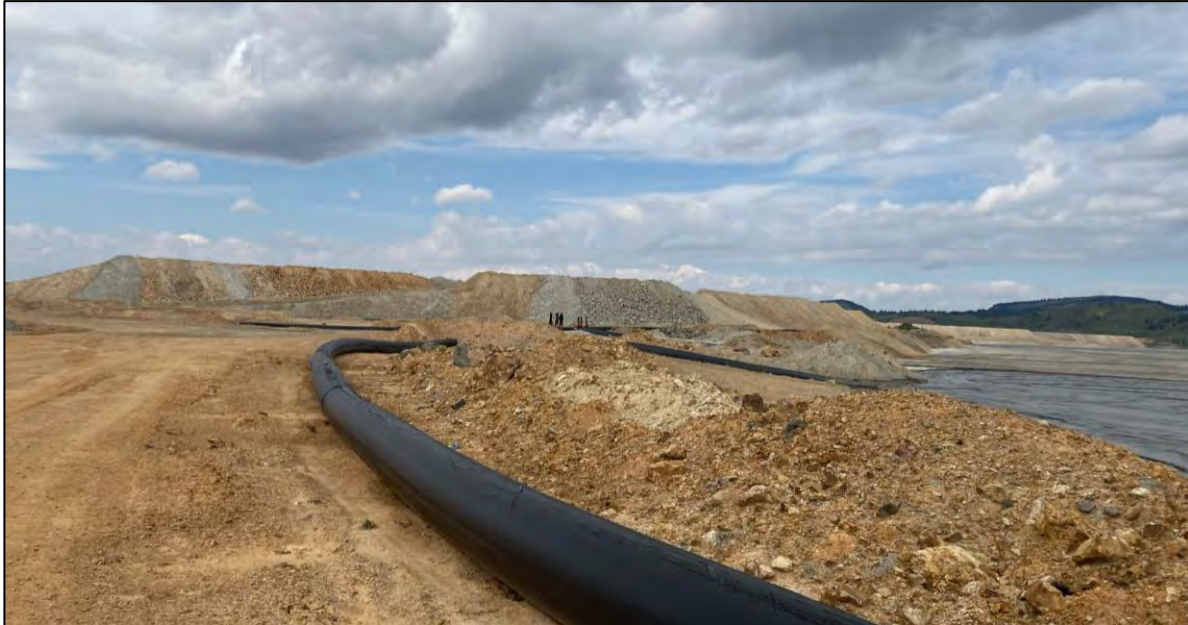
PHOTO 33 – Tailings discharge pipelines, tailings discharge location NS-1, and East-West Embankment EL. 6,450 ft surcharge zone, facing west.
