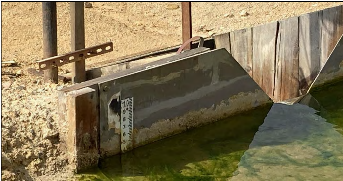
PHOTO 72 – Number 10 Seep V-notch weir staff gauge reading slightly below 0.4.
