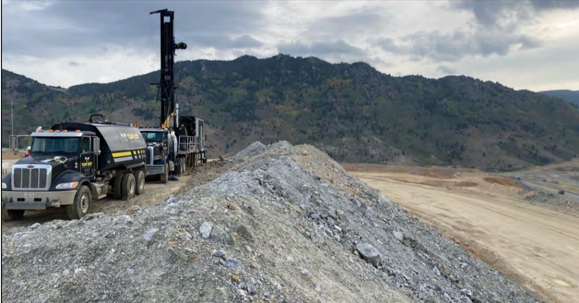
PHOTO 37 – 2021 Embankment SI drill rig on the EL. 6,450 ft surcharge zone (left). E-W Embankment EL. 6,400 ft lift (right), facing east.
