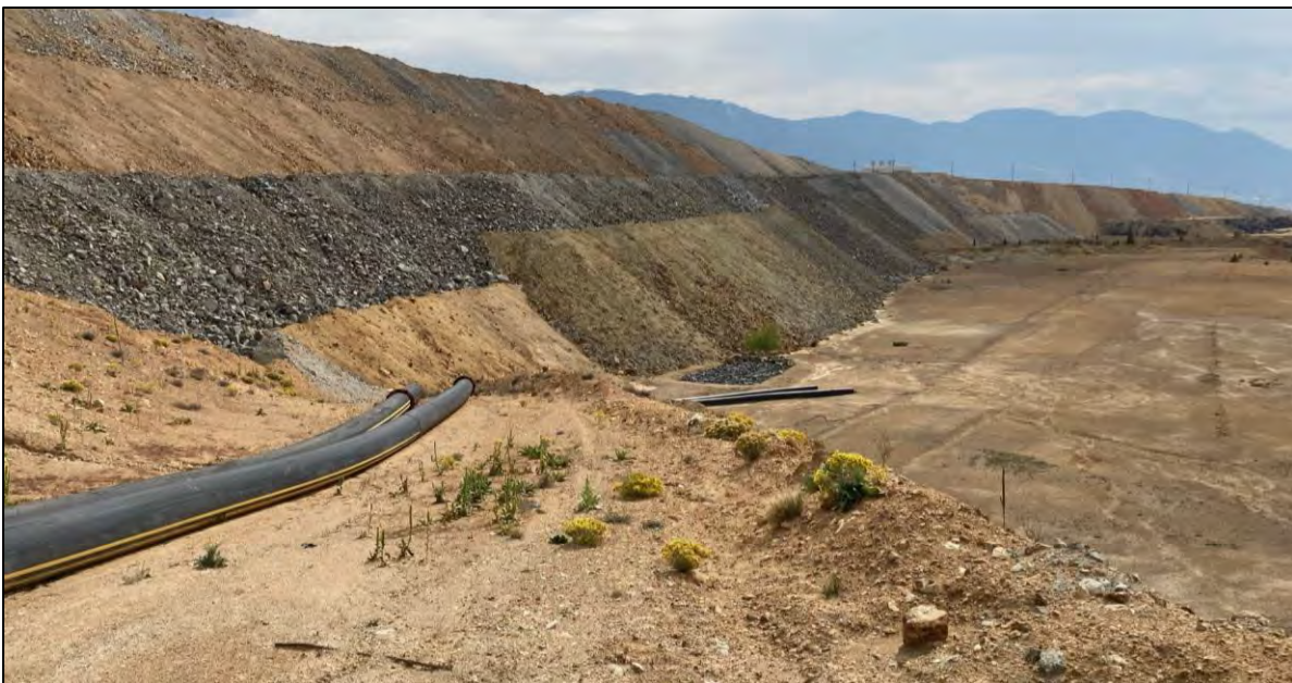
PHOTO 44 – East-West Embankment downstream slopes and WED Extraction Pond emergency overflow pipelines, west of Booster Station #3, facing southeast near Extraction Pond. Boulders for energy dissipation and final alignment of pipeline discharge remains to be completed.
