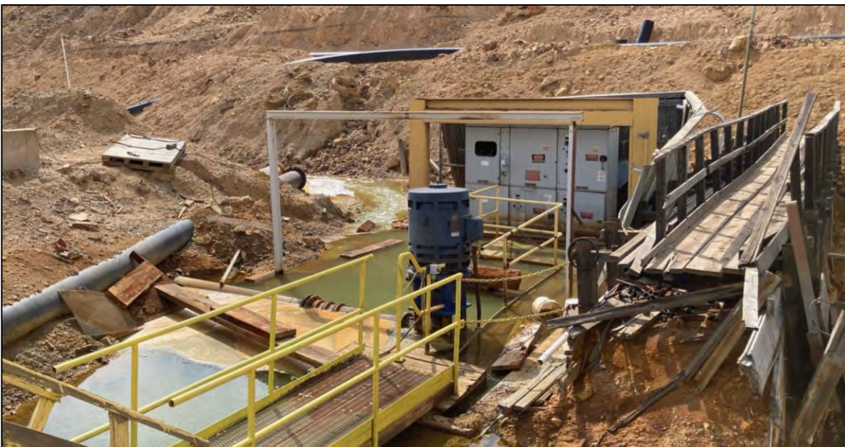
PHOTO 66 – Cell 10 Pump with overflow to the HsB Pond.
