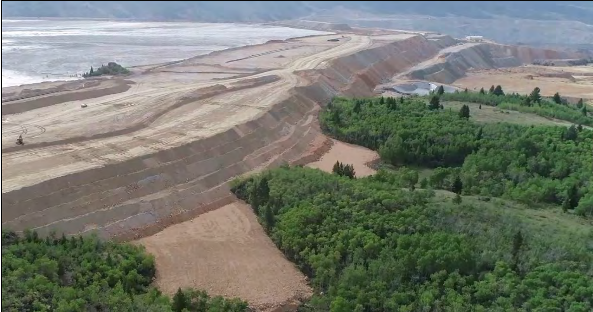
PHOTO 25 – West Embankment downstream shell, north of Rocky Knob and Extraction Pond, looking southeast.
