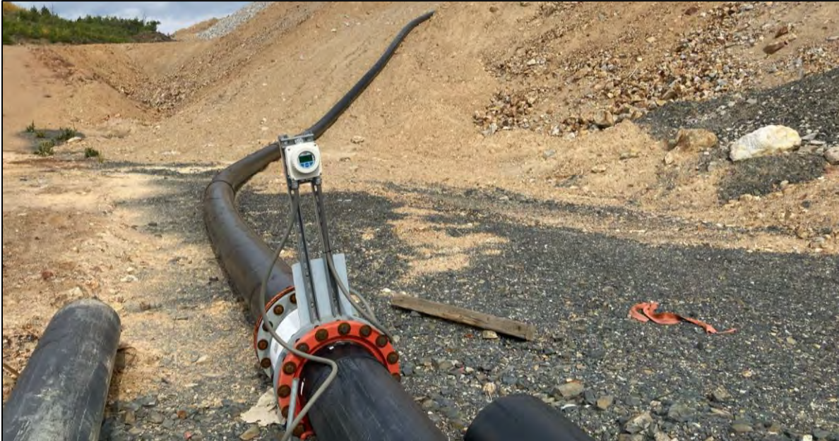
PHOTO 47 – WED Extraction Pond flowmeter on pipeline conveying recovered flow to tailings discharge location RK-1, facing north.
