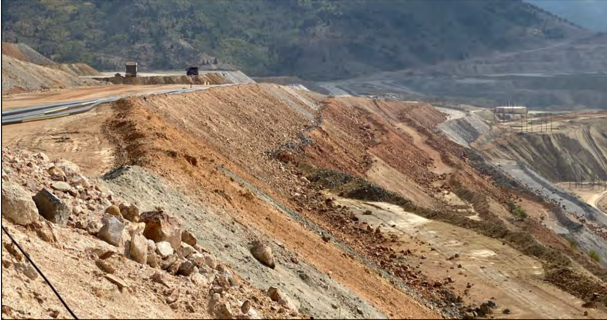
PHOTO 41 – East-West Embankment Central Pedestal Area, including East-West pipeline ramp and EL. 6,300 ft lift construction, facing east near Booster Station #3.
