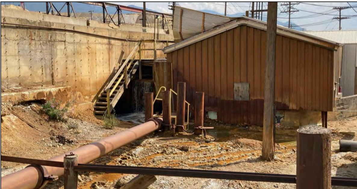
PHOTO 62 – Precipitation Plant Recirculation Pump House. There is overflow seen at the head tank under the stairs.
