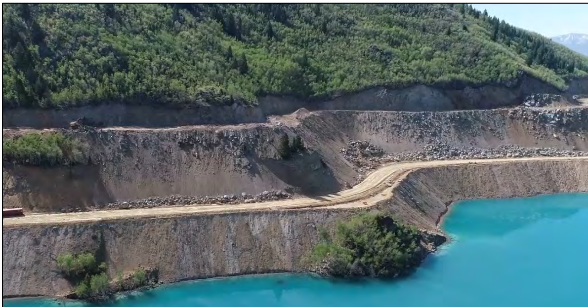
PHOTO 4 – Reclaim water pipeline road and New Reclaim Water Pipeline Ramp cut construction progress.
