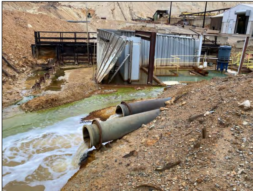
PHOTO 2 – Cell #10 Pump and Cell #5 Pipelines – Overflow to HsB Pond
