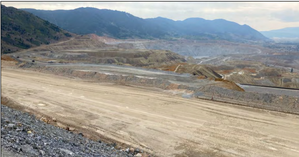
PHOTO 38 – EL. 6,400 ft lift and EL. 6,300 ft lift construction progress, facing southeast from the EL. 6,450 ft surcharge zone.
