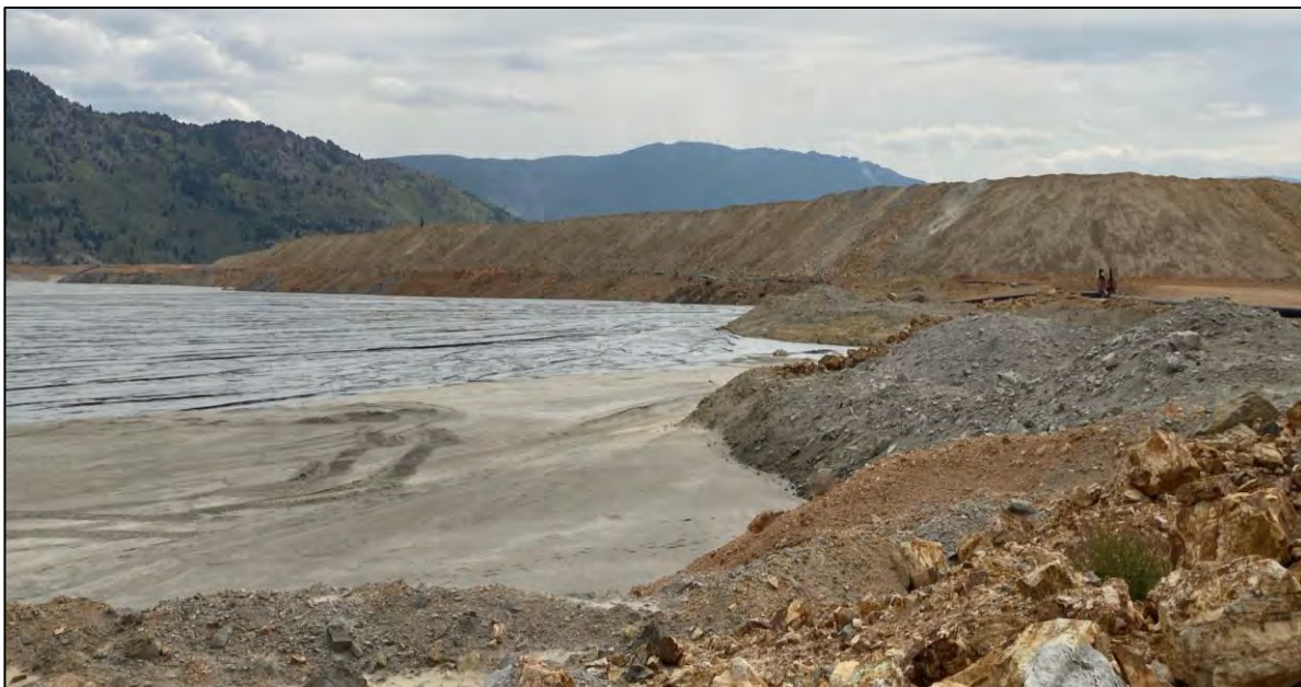
PHOTO 36 – Upstream interface of East-West Embankment – Tailings discharge location EW-1, tailings beach, and East-West Embankment EL. 6,450 ft surcharge zone.
