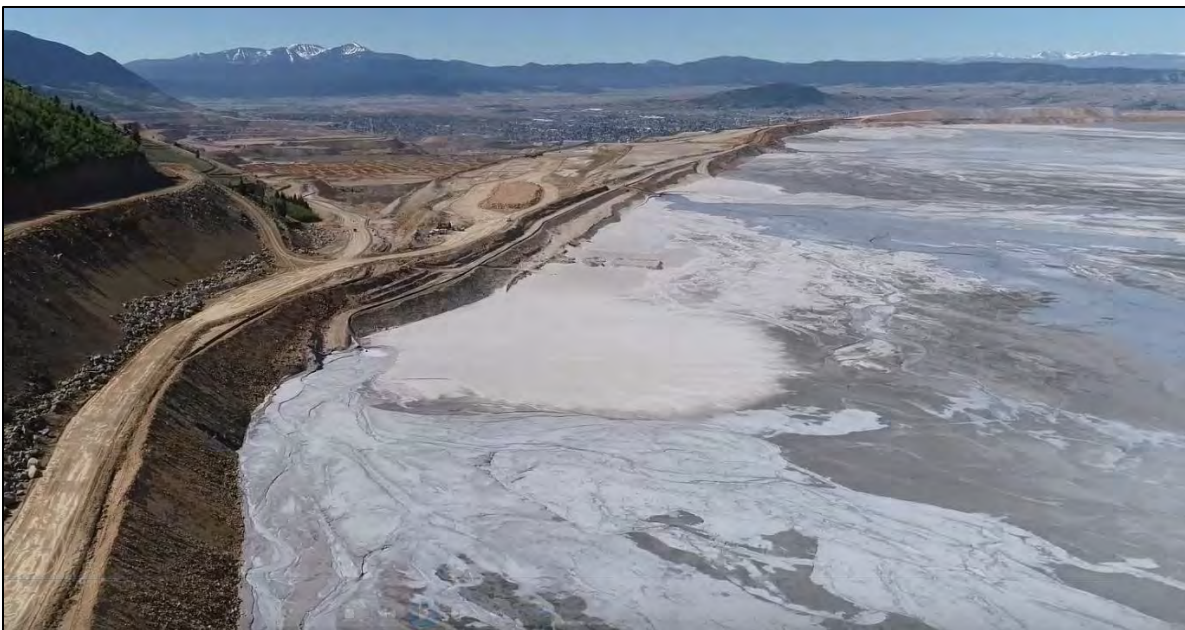
PHOTO 6 – Tailings beach beyond the northern end of the North-South Embankment near NS-4, looking south.
