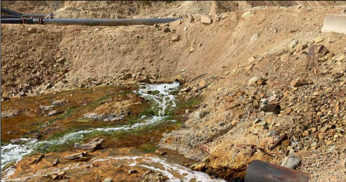
PHOTO 65 – Culvert and seepage discharging flow from Upper HsB Area to Cell 10 pump area.
