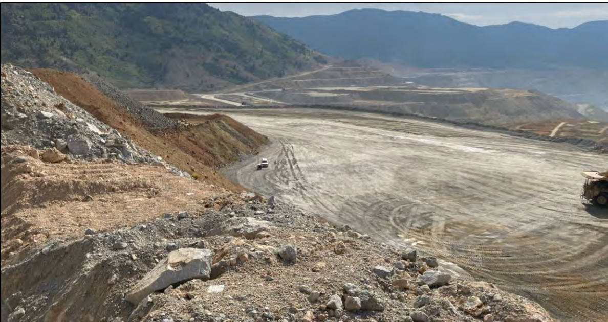
PHOTO 40 – East-West Embankment EL. 6,300 ft lift construction progress, facing southeast from EL. 6,400 ft lift crest in Central Pedestal Area.
