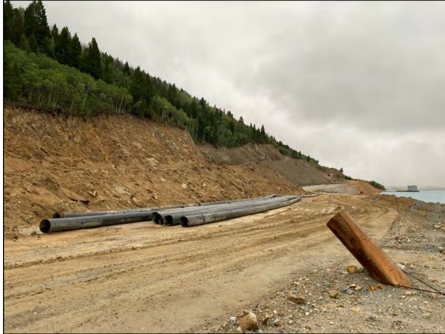
PHOTO 15 – Reclaim Pipeline Access Road – Construction progress, viewed from the north end of the existing reclaim access road
