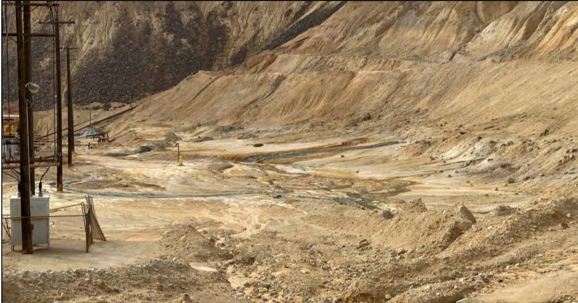
PHOTO 59 – Overview of daylighting seeps along the YDTI downstream toe in the HsB Area, facing west.
