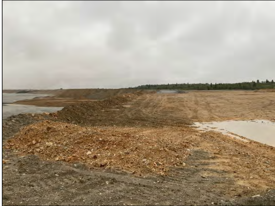
PHOTO 11 – West Embankment – EL. 6,450 ft crest, viewed from the north end of the embankment, looking South
