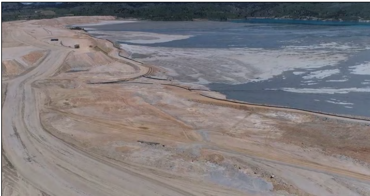
PHOTO 18 – East-West Embankment EL. 6,450 ft lift (left) and EL. 6,450 ft rockfill surcharge subgrade preparation (right) with view of beach adjacent to discharge locations EW-1 and EW-2, looking north.
