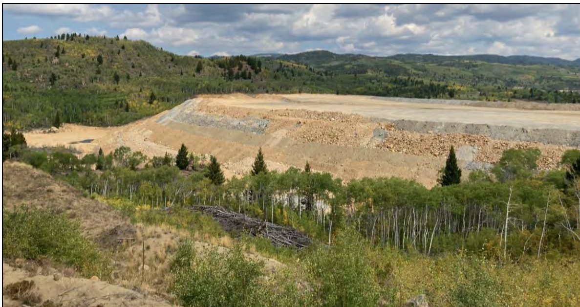
PHOTO 52 – Downstream side of northern end of West Embankment, 5 ft lifts of D1 material placed downstream of U material. Facing north from West Ridge topsoil stockpile.
