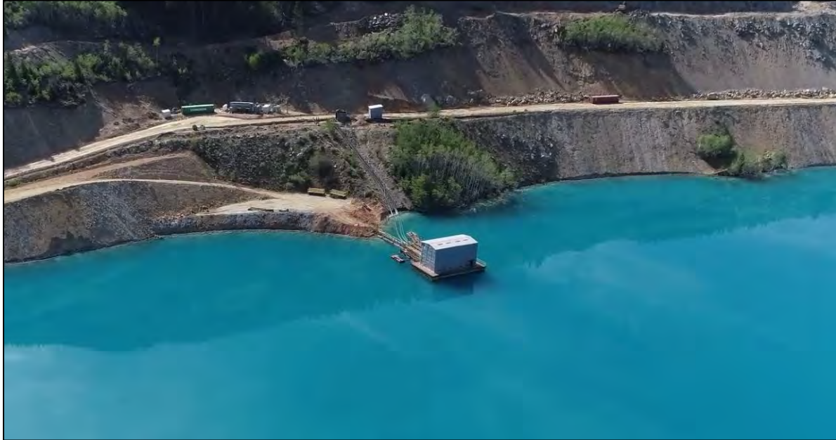
PHOTO 3 – Old Reclaim Barge and New Reclaim Water Pipeline Ramp cut construction progress.
