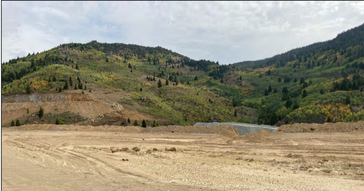
PHOTO 29 – New Reclaim Water Pipeline Ramp hillside cut (left) and ramp (right) tie-in area, facing east from North-South Embankment EL. 6,400.
