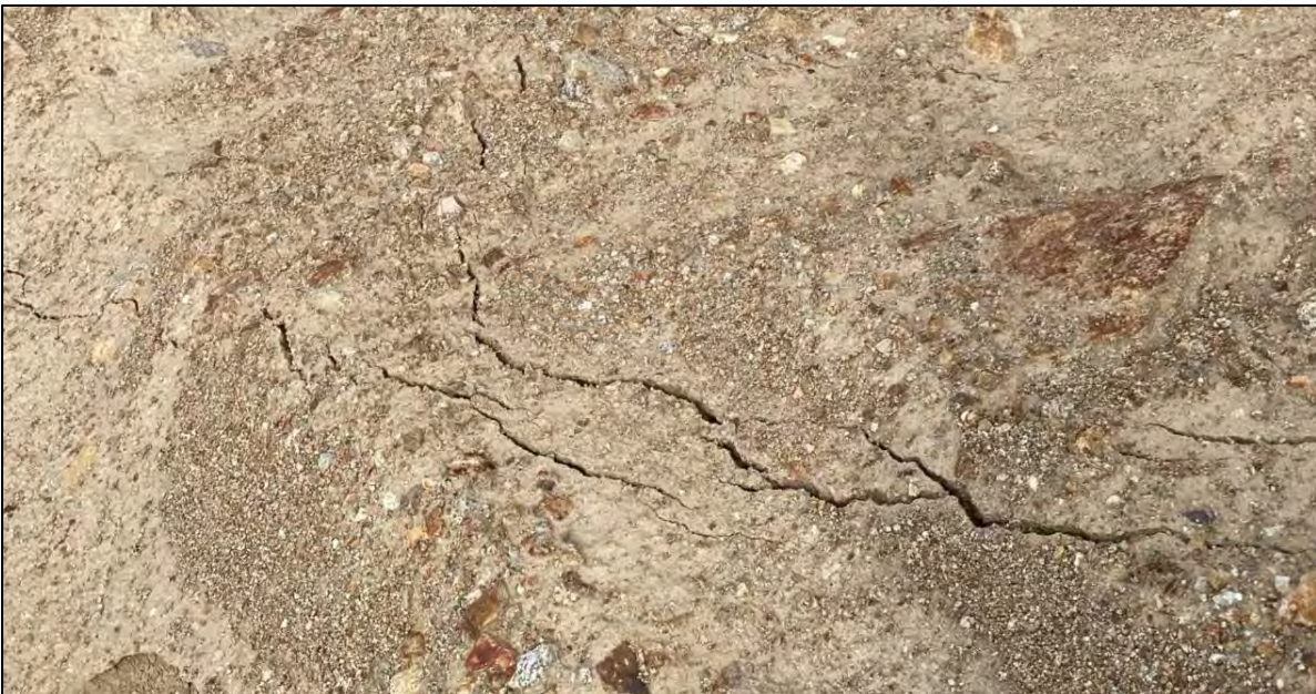
PHOTO 50 – Cracking observed along recently placed areas of the EL. 6,450 ft lift on the West Embankment.
