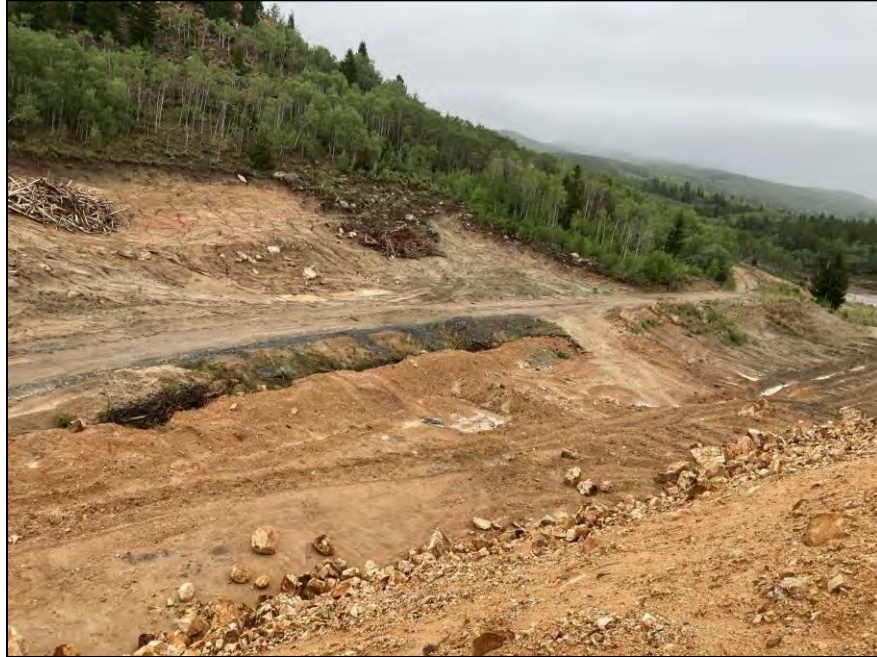
PHOTO 9 – West Embankment – North end of the EL. 6,450 ft lift, to be completed following municipal water pipeline relocation
