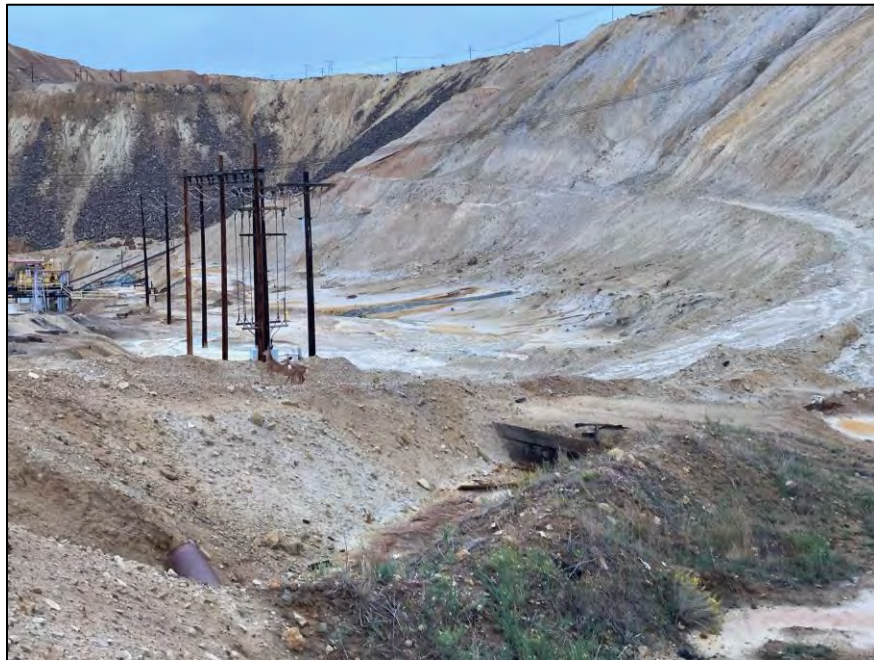
PHOTO 4 – East-West Embankment – General overview of the various seeps at the toe of the embankment
