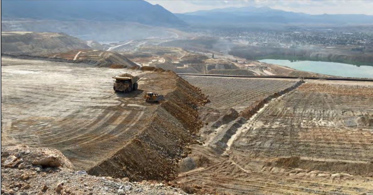
PHOTO 39 – East-West Embankment EL. 6,300 ft lift construction, facing south from EL. 6,400 ft lift crest in Central Pedestal Area.
