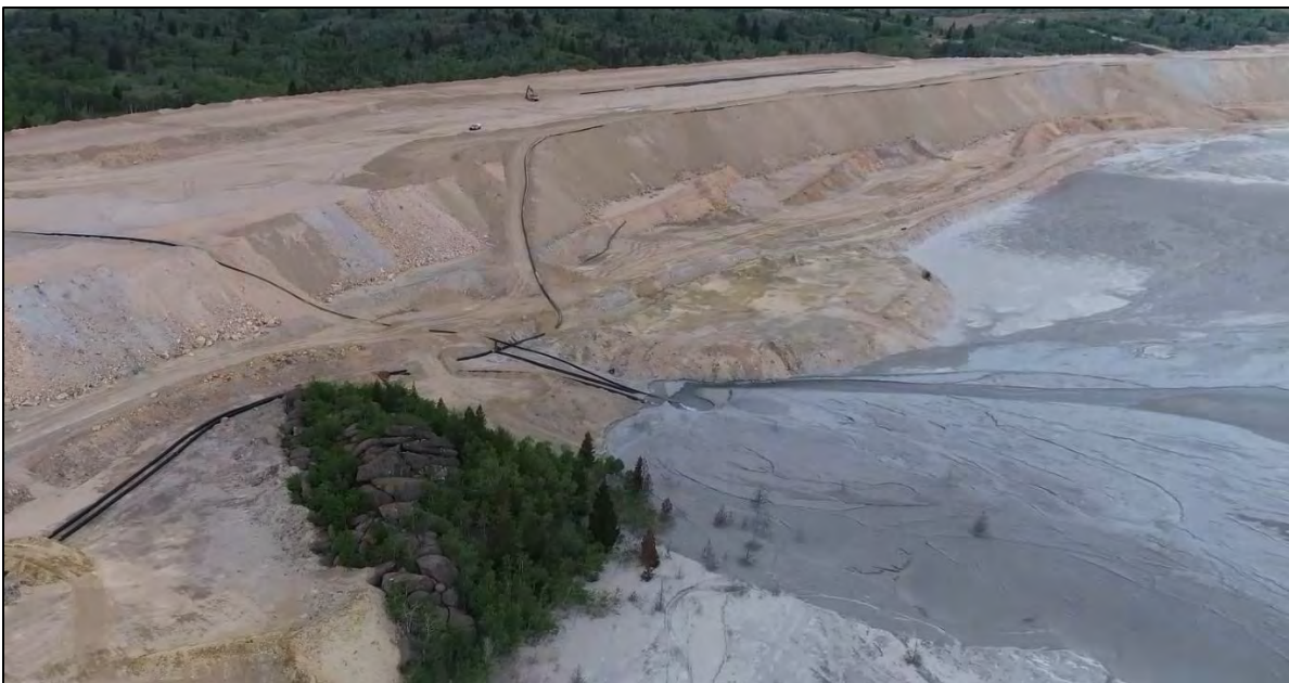
PHOTO 20 – East-West Embankment and West Embankment upstream side, near Rocky Knob and discharge location RK-1, facing west.
