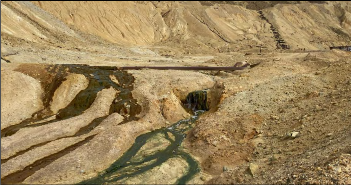
PHOTO 61 – Seepage along the YDTI downstream toe in the HsB Area, facing east.
