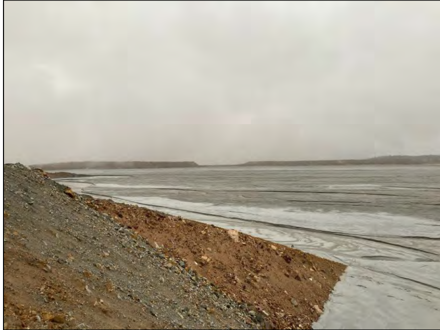
PHOTO 13 – East-West Embankment – EL. 6,450 Zone U Surcharge construction, viewed from the North-South Embankment
