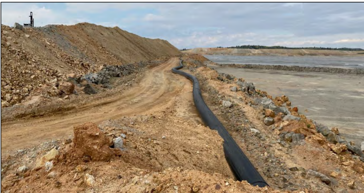
PHOTO 34 – East-West Embankment EL. 6,450 surcharge zone (left), tailings pipeline (middle), and tailings beach (right), west of tailings discharge location NS-1, facing west.
