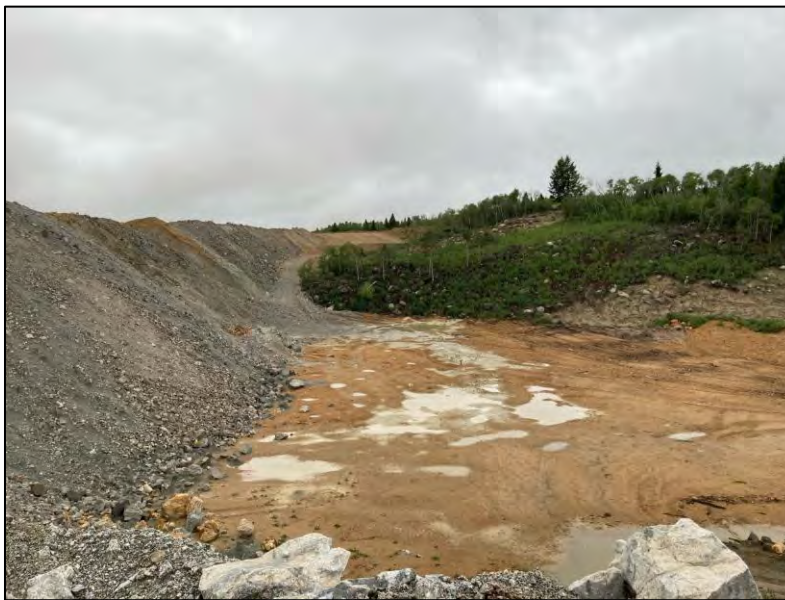
Photo 3.3 Incomplete D1 material placement at Ridge Road facing South
