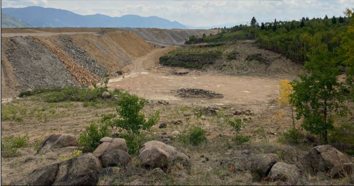
PHOTO 53 – Downstream side of West Embankment south of the Ridge Road. U material placement complete, D1 material placement ongoing in 2021. Facing southeast.
