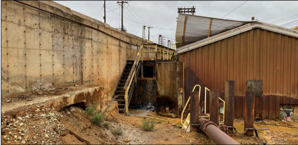
PHOTO 3 – Precipitation Plant – Recirculation pump house overflow
