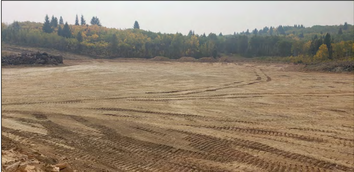
PHOTO 11 – West Embankment – EL 6,400 ft Zone D1 Material near Temporary Extraction Pond location
