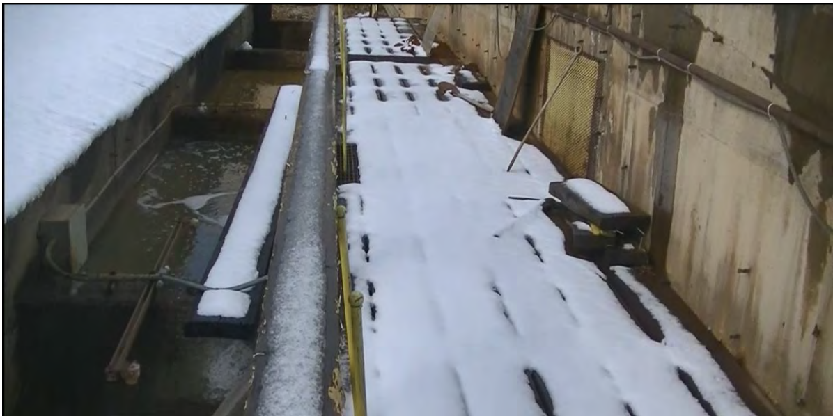
PHOTO 6 – Oct 15, 2020 – Precipitation Plant Recirculation Pump House head tank water level. Water is approximately 1 ft below the top of the concrete separators.
