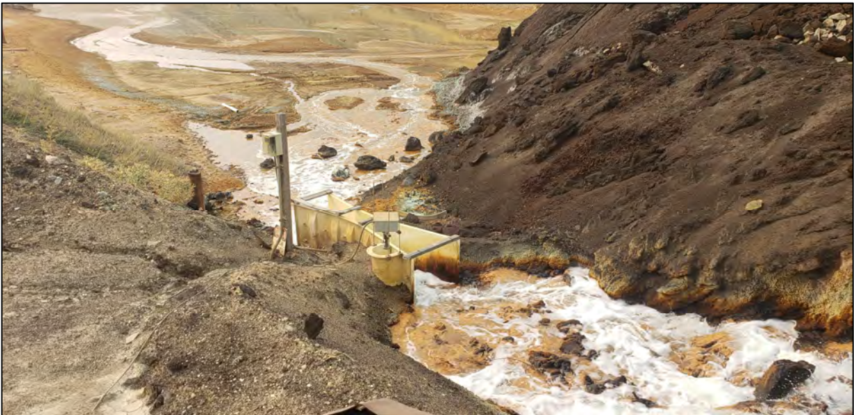
PHOTO 26 – HsB Area – Cell 10 Return Water Flume
