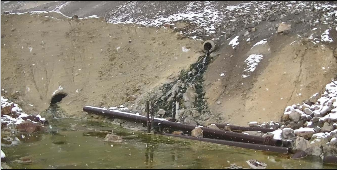
PHOTO 54 – Number 10 Seep collection area inflow.
