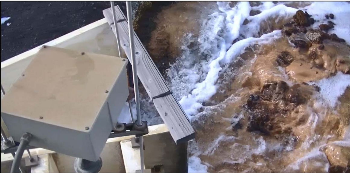
PHOTO 70 – Inlet of Parshall flume providing measurement of Cell 10 discharge flow.
