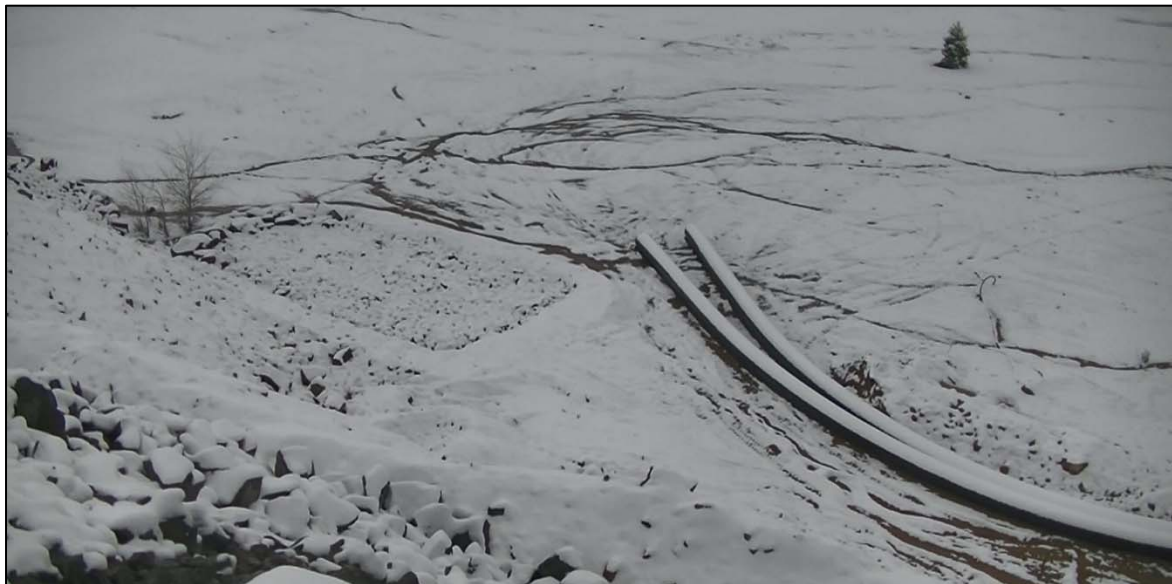
PHOTO 45 – Snow-covered WED Extraction Pond emergency overflow pipelines, boulders for energy dissipation and final alignment of pipeline discharge remains to be completed.
