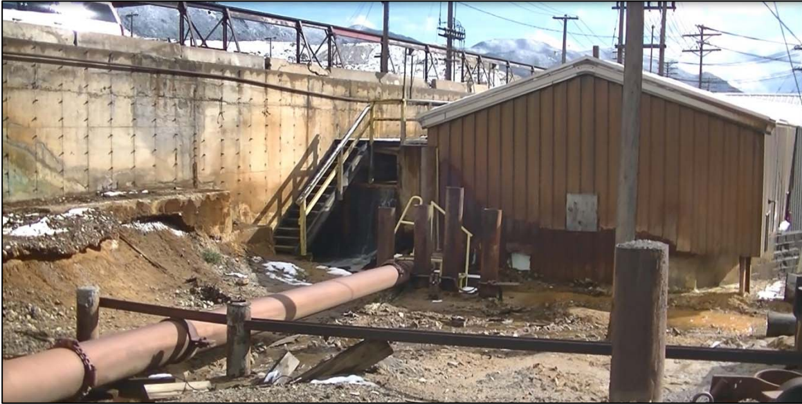
PHOTO 66 – Precipitation Plant Recirculation Pump House. There is overflow seen at the head tank under the stairs.
