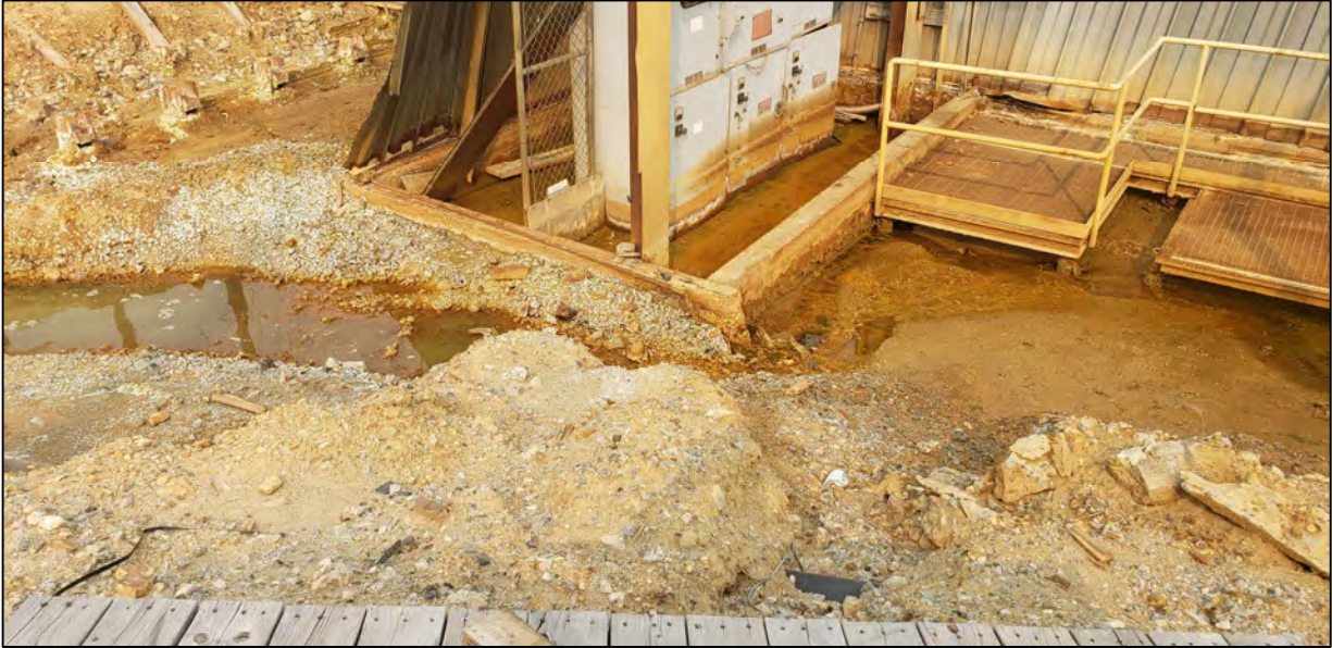
PHOTO 25 – HsB Area – Cell #10 Pump, minor overflow to HsB Lower Pond
