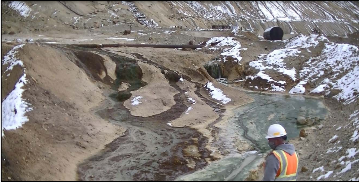
PHOTO 30 – Seepage (leach seeps) along the downstream toe of the East-West Embankment in HsB Area, looking east.
