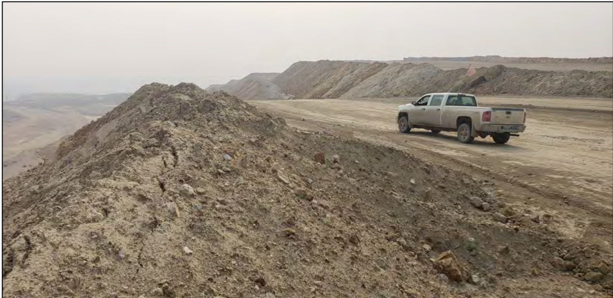
PHOTO 5 – North-South Embankment – Downstream edge of Haul Ramp showing minor settlement cracking along EL 6,400 lift
