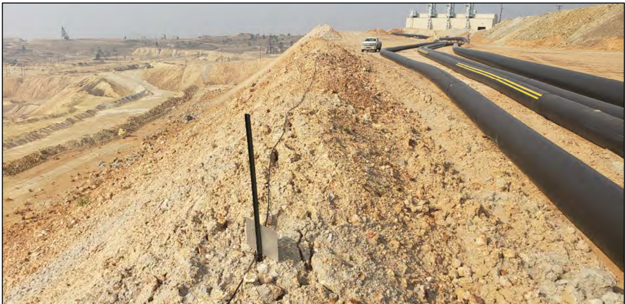
PHOTO 8 – East-West Embankment – Downstream edge of pipeline ramp showing minor settlement cracking
