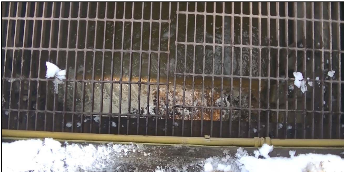
PHOTO 67 – Precipitation Plant overflow weir.
