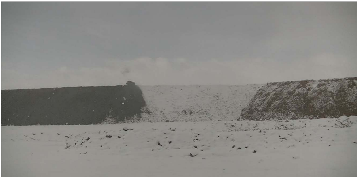
PHOTO 33 – Close-up of construction of EL. 6,450 ft lift on East-West Embankment near discharge location EW-2.
