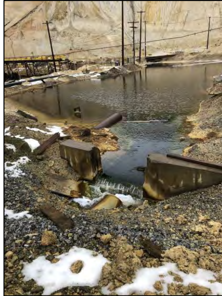
PHOTO 9 – Nov 18, 2020 – Hooligan Pond bypassing flows location A: Hooligan Pond and bypassing flow through weir.
