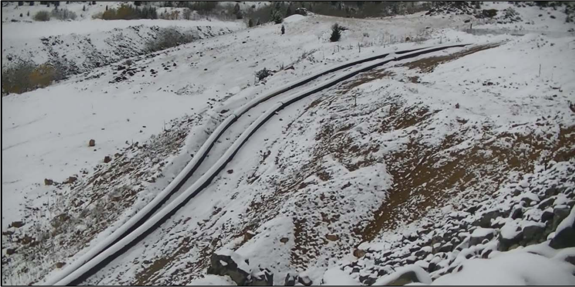
PHOTO 44 – Snow-covered WED Extraction Pond emergency overflow pipelines.
