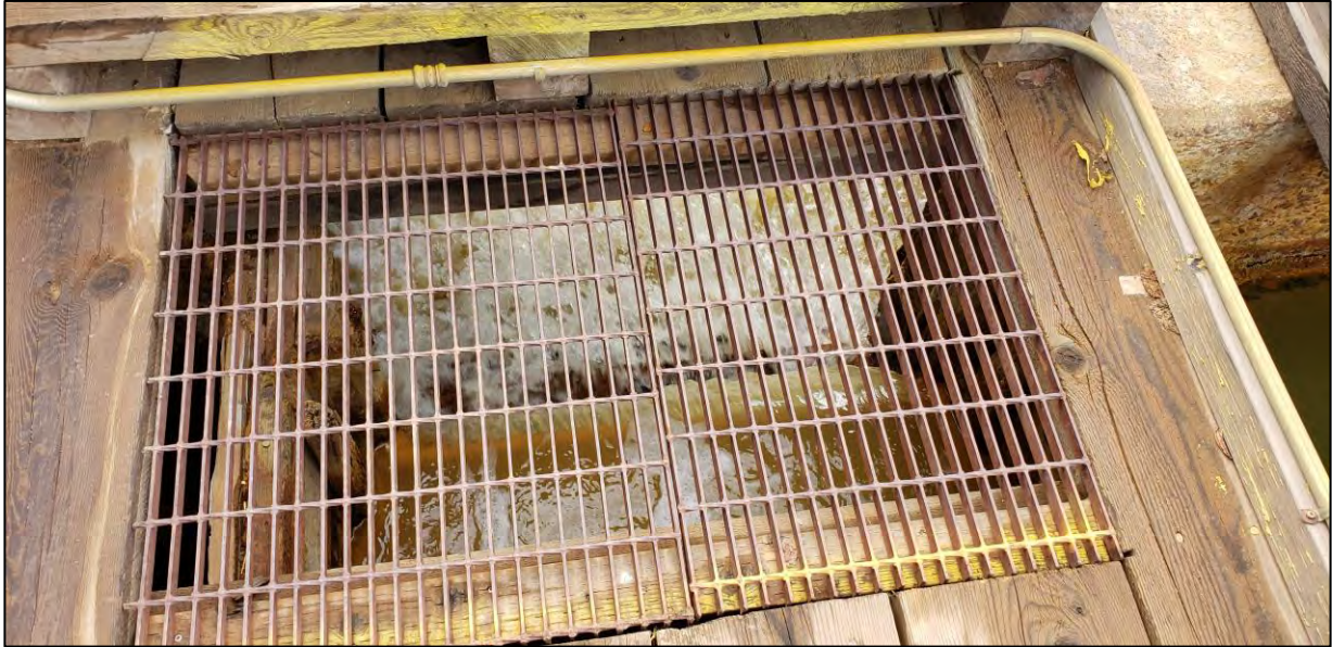
PHOTO 7 – Oct 30, 2020 – Flow through Precipitation Plant overflow weir.
