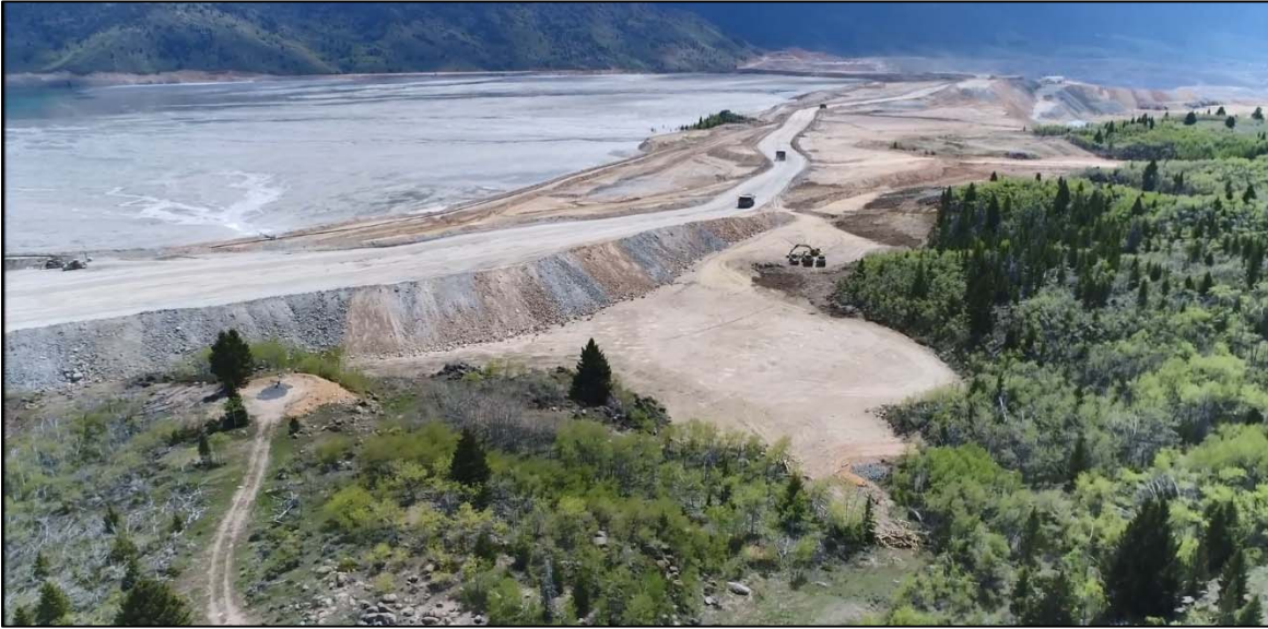
PHOTO 19 – West Embankment downstream shell with ramp up to EL. 6,450 ft, looking southeast.
