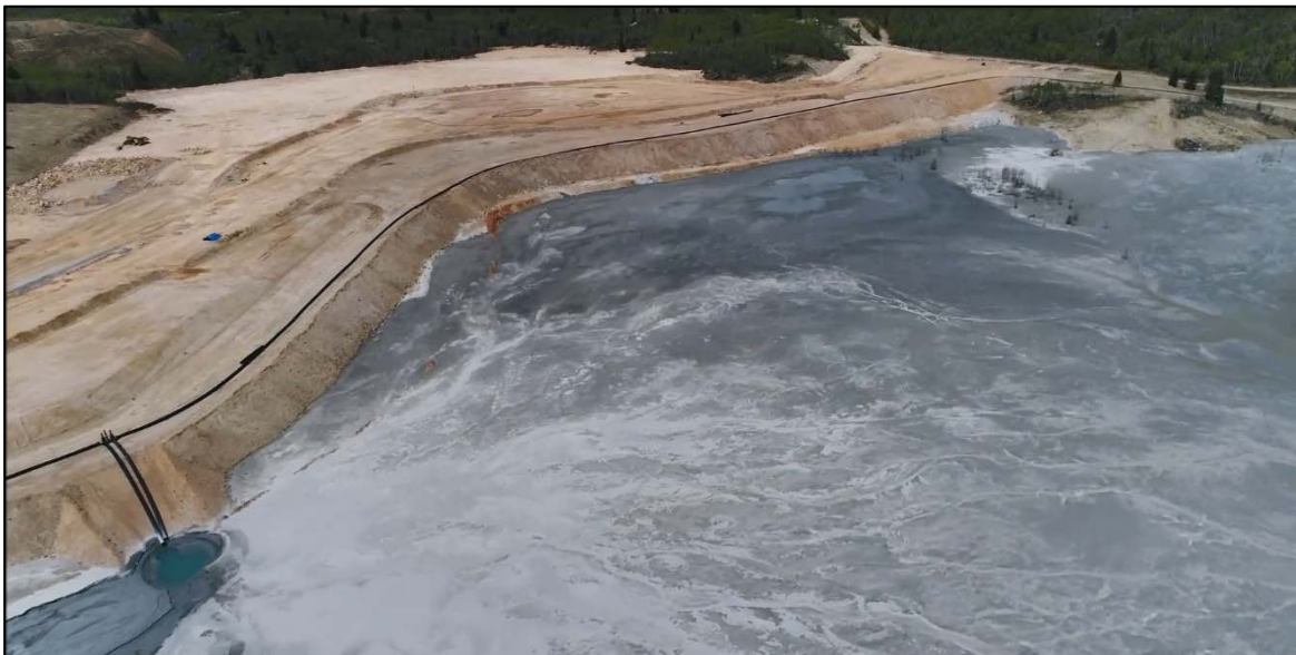
PHOTO 18 – Northern end of the West Embankment, upstream interface, looking northwest near discharge location RK-3.
