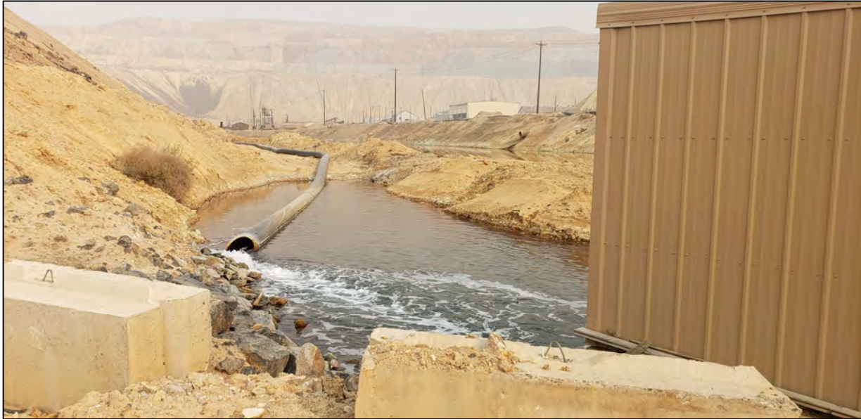
PHOTO 29 – HsB Area – HsB Water Treatment Plant Transfer Pond
