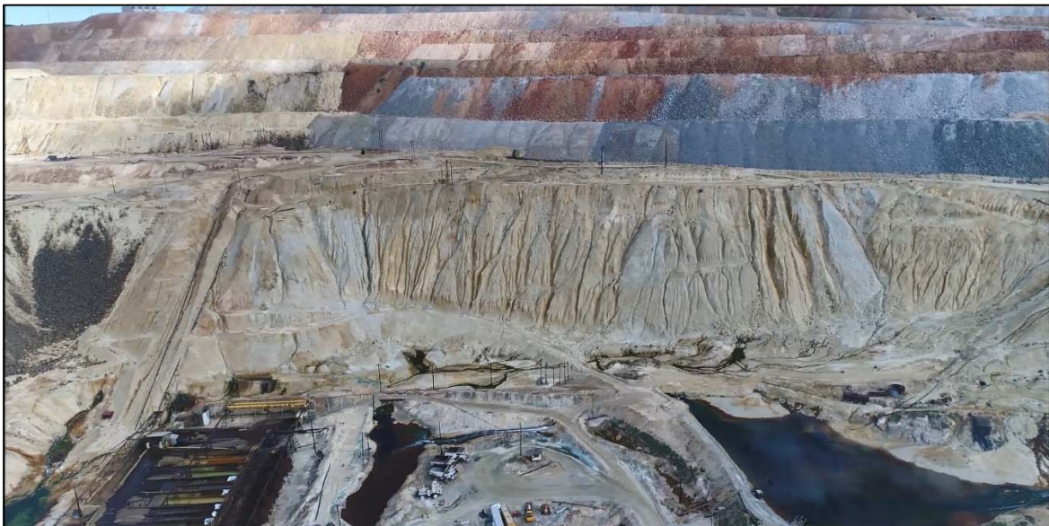
PHOTO 10 – East-West Embankment downstream slope, Number 10 Seep bench area, HsB and Leach Seeps area, looking north.
