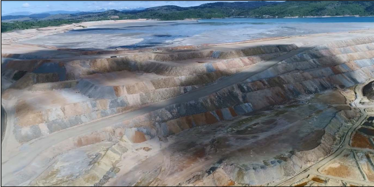
PHOTO 1 – North-South Embankment downstream shell, looking northwest from southeast end of YDTI at the new mine haul ramp.
