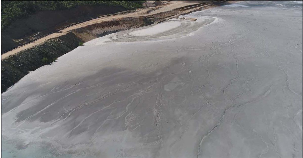
PHOTO 5 – Tailings beach beyond the northern end of the North-South Embankment near former position of tailings discharge location, NS-3, looking southeast.
