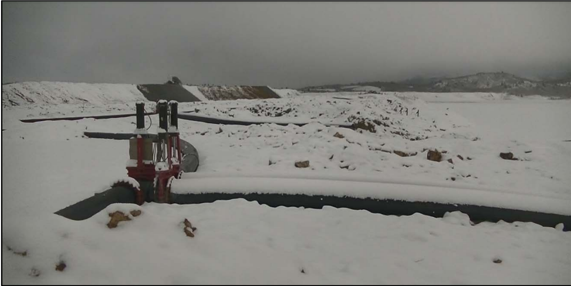
PHOTO 32 – Snow-covered tailings discharge pipeline valve near discharge location EW-1, and construction of a new EL. 6,450 ft lift on East-West Embankment near discharge location EW-2.
