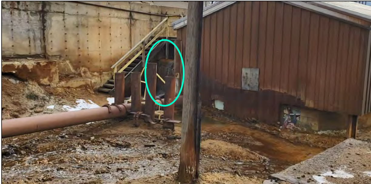
Photo 7.3 Precipitation Plant Recirculation Pump House. Water is overflowing from the head tank under the stairs.
