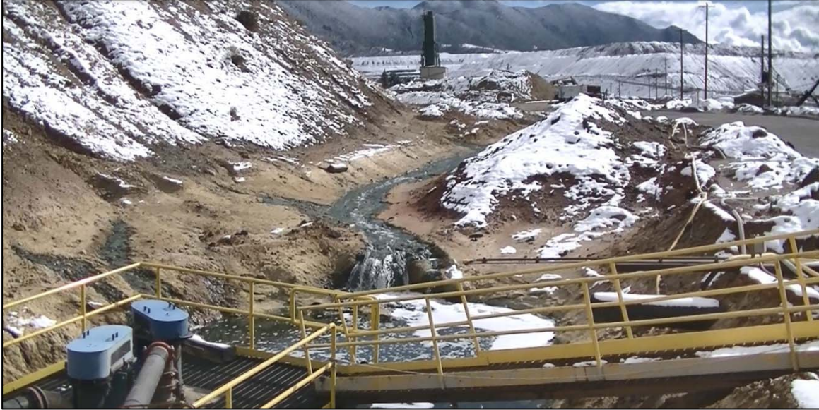
PHOTO 62 – Muddler Pump operating with a small overflow to the HsB Pond.
