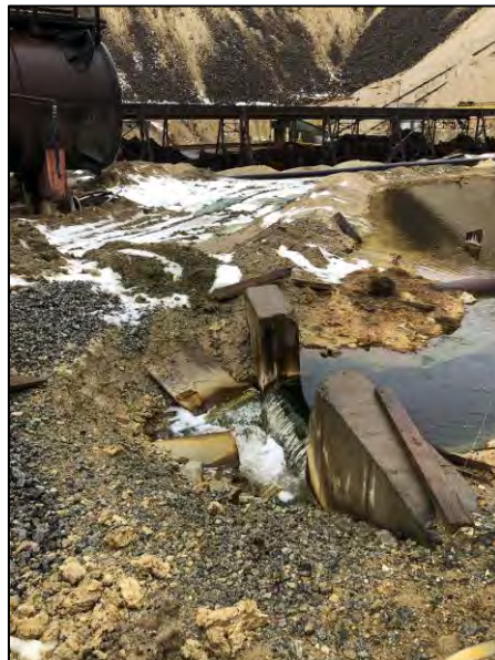
PHOTO 10 – Nov 18, 2020 – Hooligan Pond bypassing flows location A: close-up of flow bypassing through weir.
