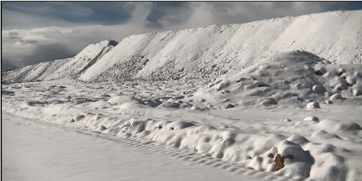
PHOTO 37 – Upstream face of recently construction EL. 6,450 ft lift along the West Embankment.
