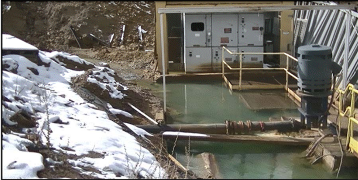
PHOTO 68 – Cell 10 Pump with overflow bypassing.
