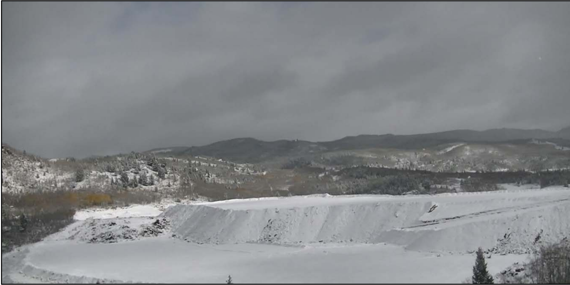
PHOTO 42 – Downstream side of the West Embankment at the northern end looking northeast. Zone U fill placement to EL. 6,450 ft completed; Zone D1 remains to be placed on the downstream side.
