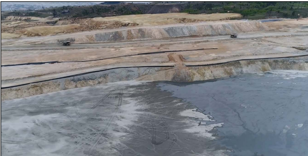
PHOTO 14 – Upstream side of the East-West Embankment located west of No. 3 (Tailings) Booster Pump House, facing ramp for placement of the EL. 6,450 ft lift
